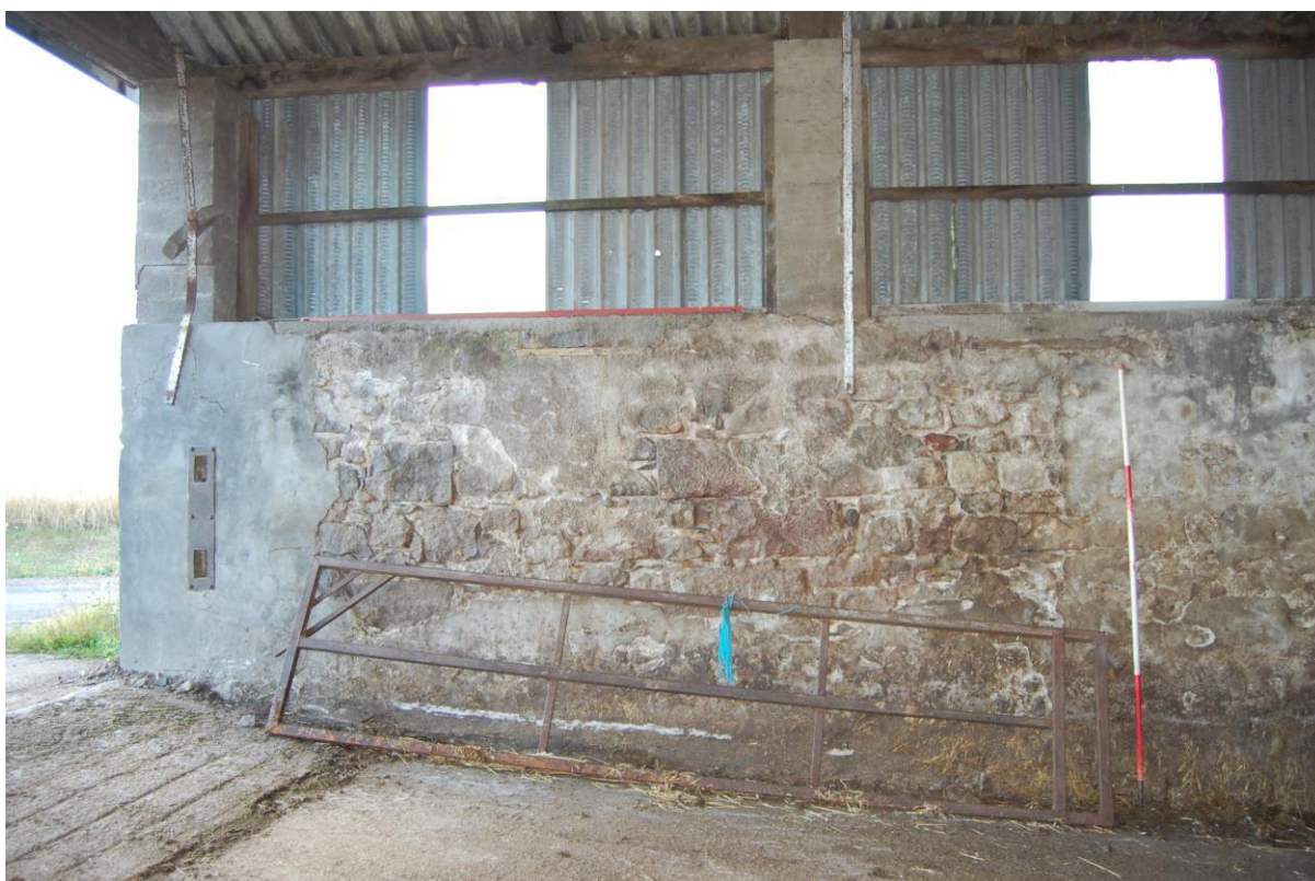
Illus 21 Shed 5 SSE wall with remains of blocked window W1 (left of centre), this end of the wall has been heavily rebuilt; facing SSE
