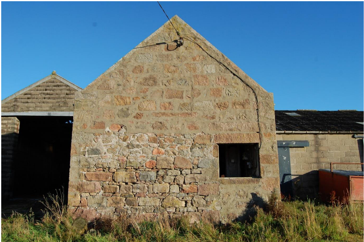
Illus 18 Shed 3 SSE gable with D1 (later converted to window); facing NNW
