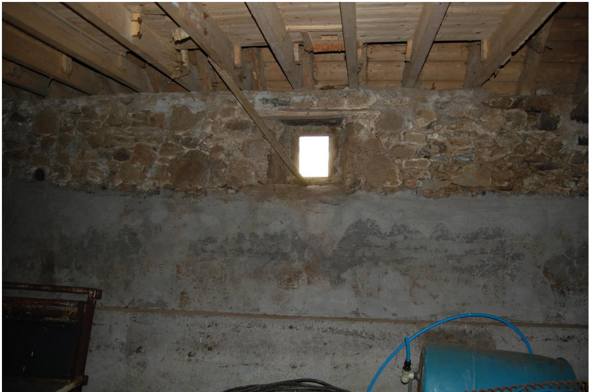
Illus 9 Room 7 S wall window W16 showing concrete lining when buildings modernized for animal use; facing SSE
