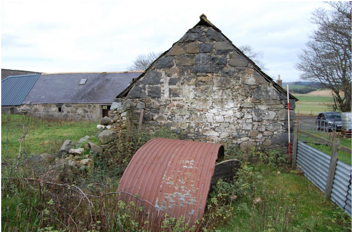
Illus 12 S gable Room 10 with blocked window W17 (first floor) and Room 11 as earthwork (foreground); facing NNW
