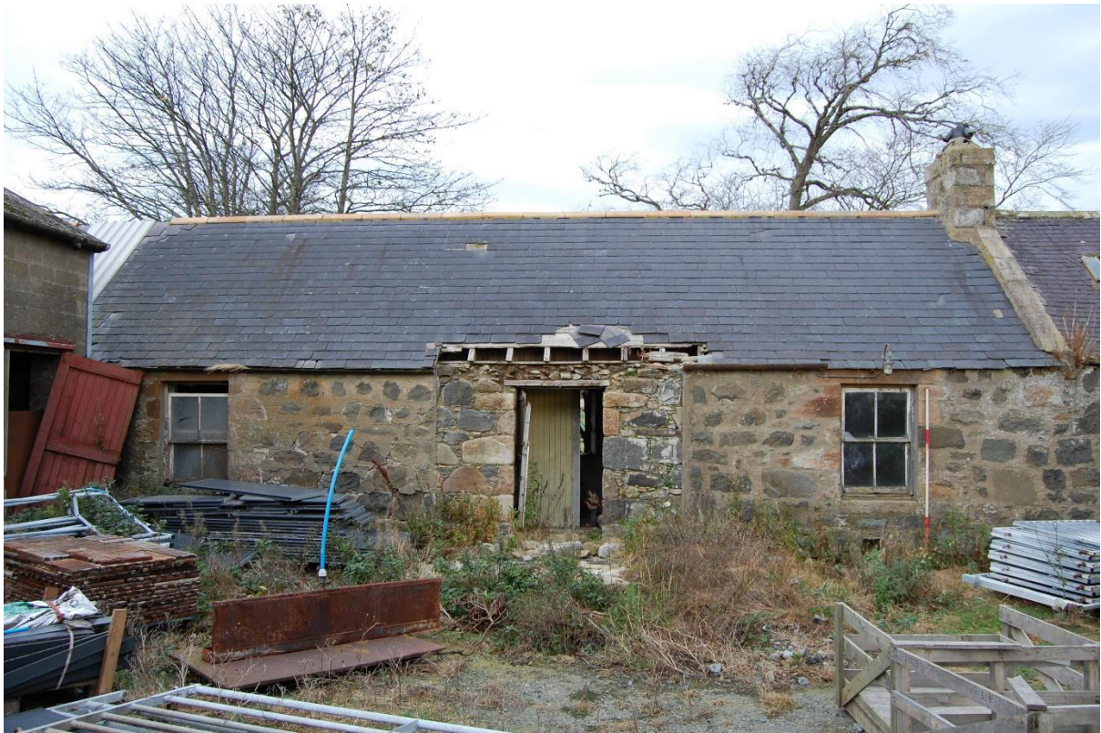
Illus 5 Phase 1 cottage S wall Rooms 3 and 4, W1, D1, W2; facing NNW
