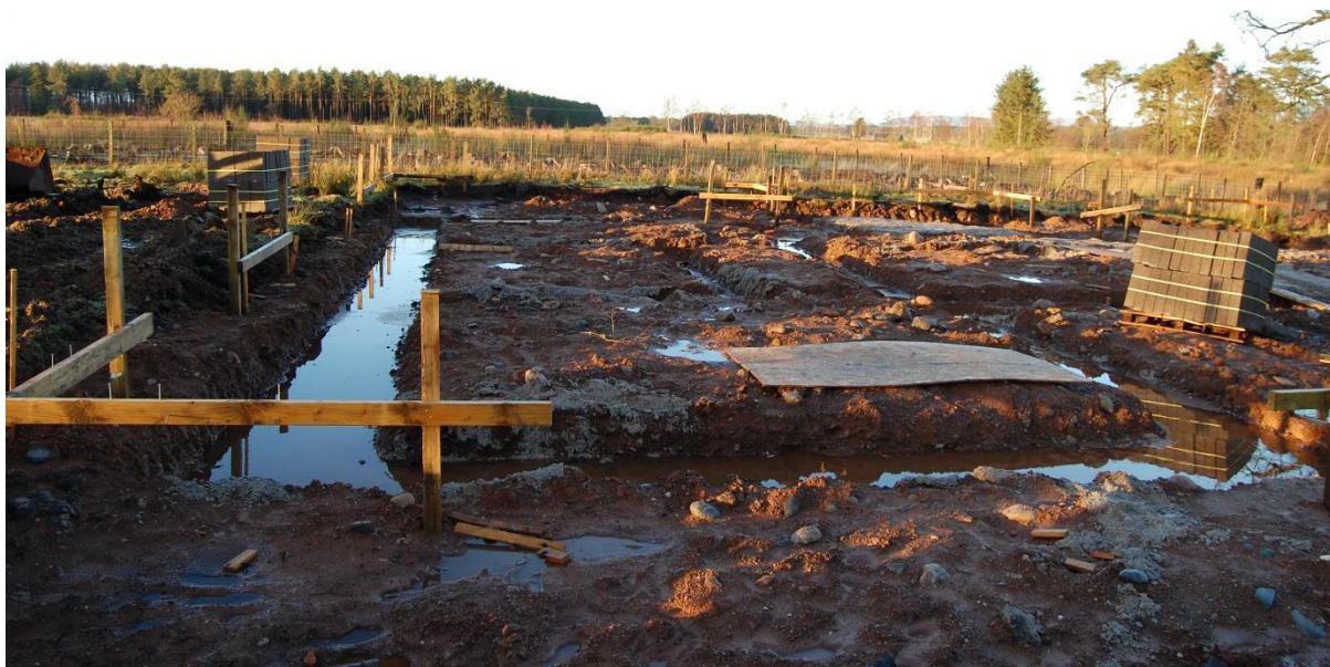
Illus 5 Site of house with topsoil removed and foundation trenches dug and cemented; facing W
