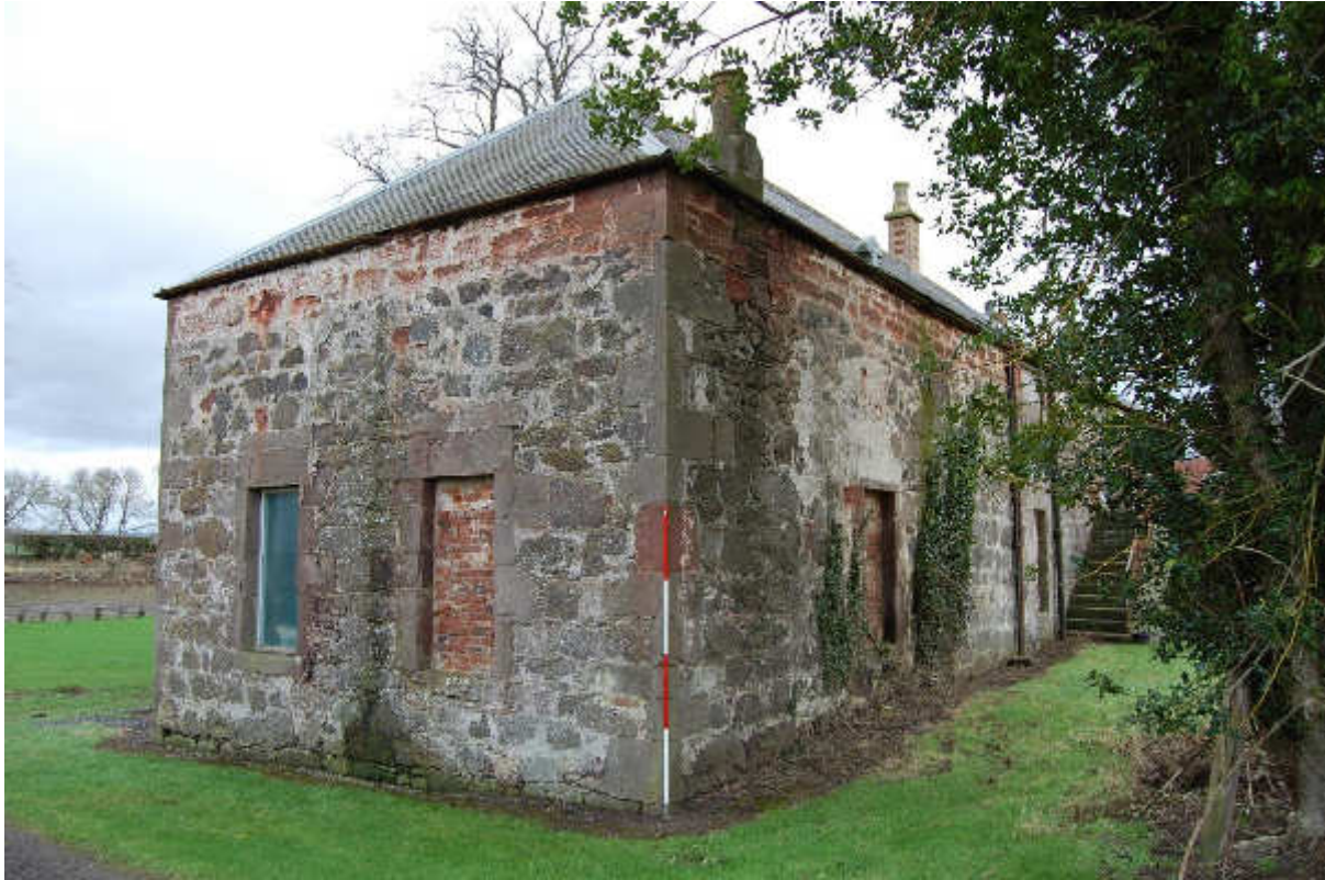
Illus 6 Building 1 SW corner showing red sandstone to raise height of building
