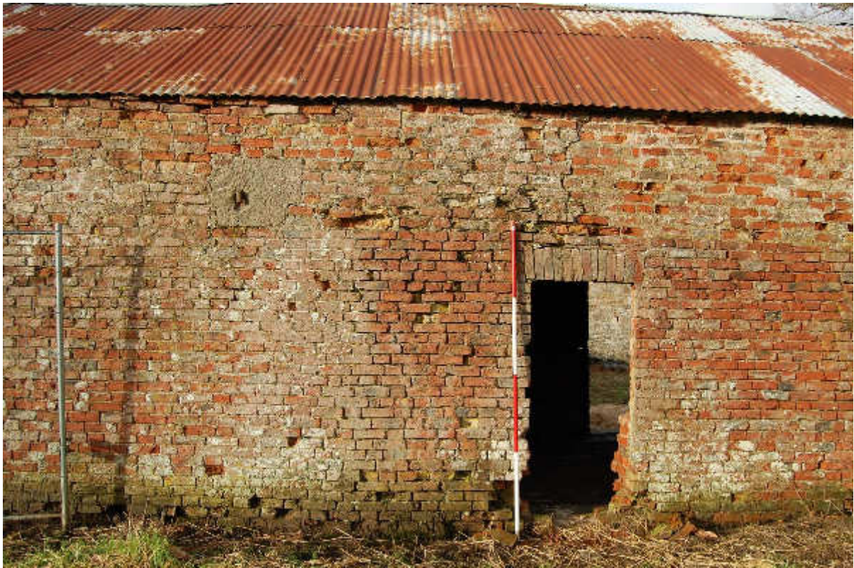
Illus 16 Building 2 E wall sandstone block F23 (left top) and arched brick door D8 (right); facing W
