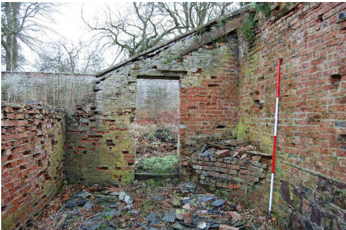
Illus 30 Building 5 interior E end with door D14 and brick base F40 (centre right); facing E
