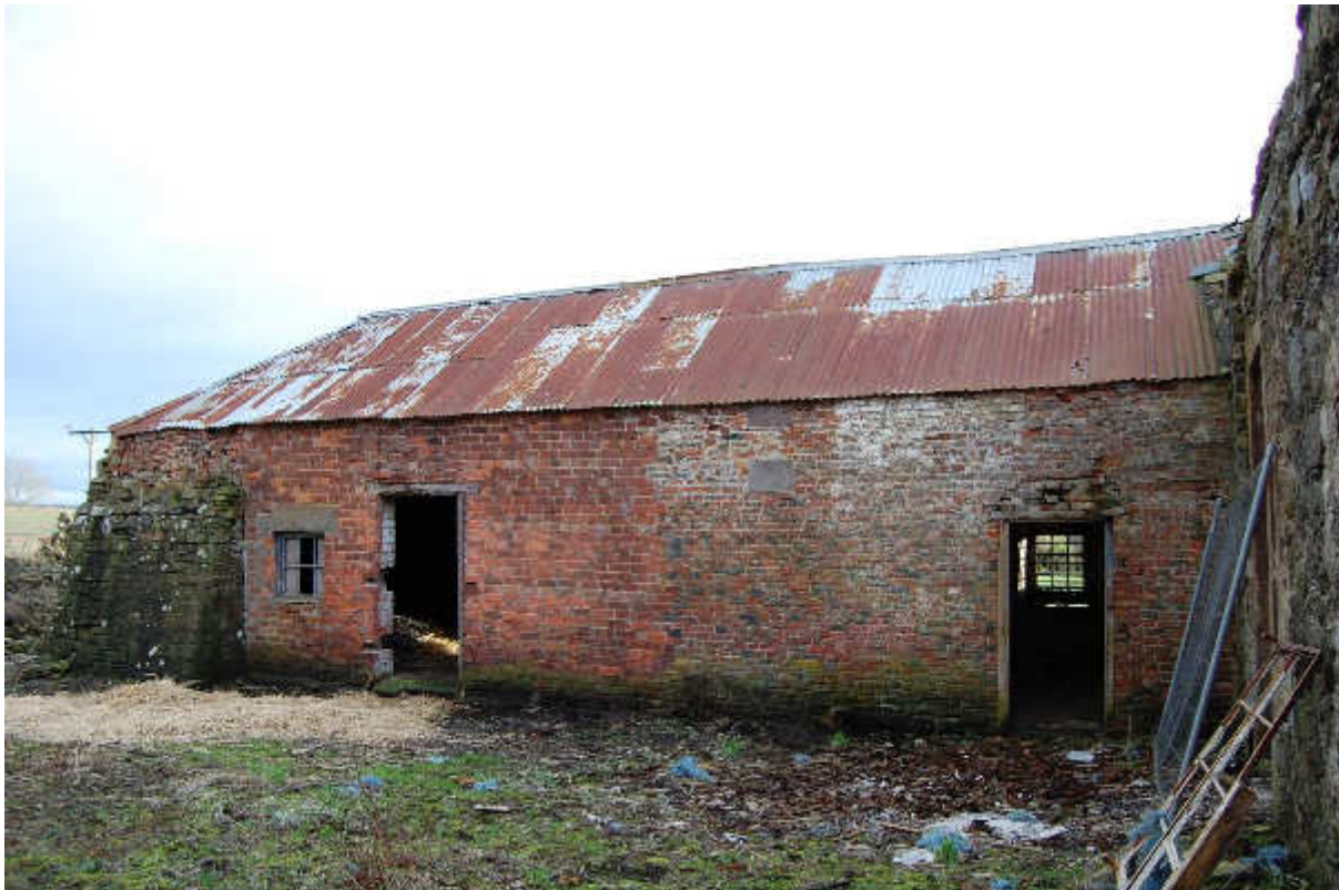
Illus 13 Building 2 W wall with buttress F20 (left) W19, D9, D16 showing two different brick types; facing NE
