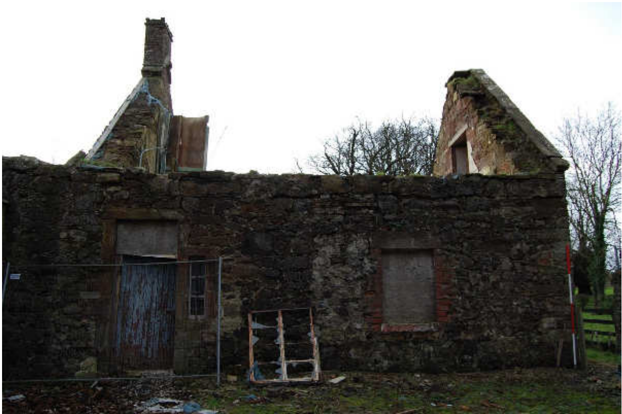
Illus 19 Building 3 N wall with D6, W16 and W21 (right) showing collapsed roof; facing S
