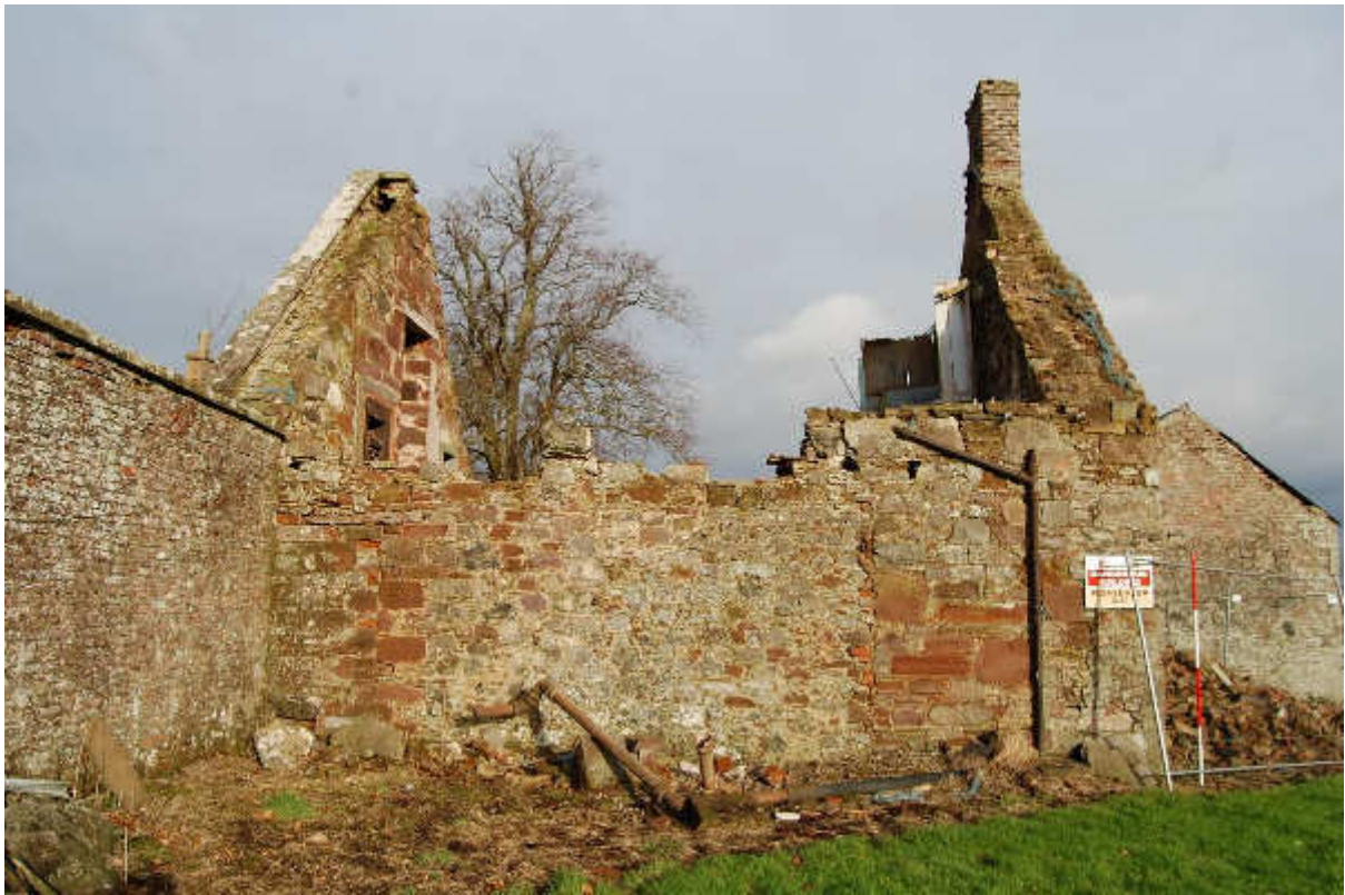
Illus 21 Building 3 S wall with garden wall F24 (left) blocked door D5 (centre left), sandstone blocks F26 (right centre); facing N
