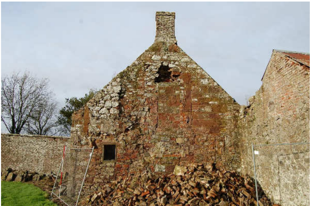
Illus 20 Building 3 E wall showing W18 (bottom left), wall scar F57 (above W18) and fireplace and flue F55 and F456 below; facing W
