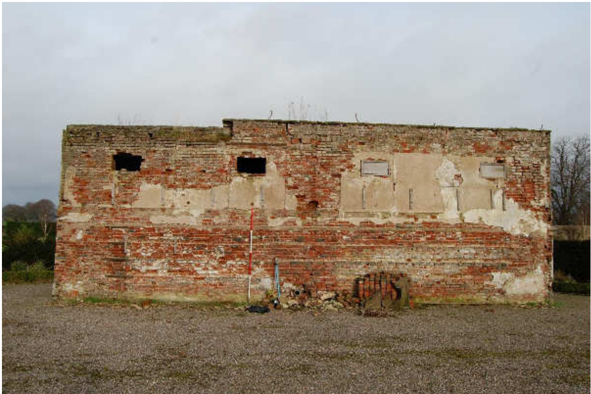
Illus 24 Building 4 S wall with firebrick flue F29 behind rubble in centre; facing N
