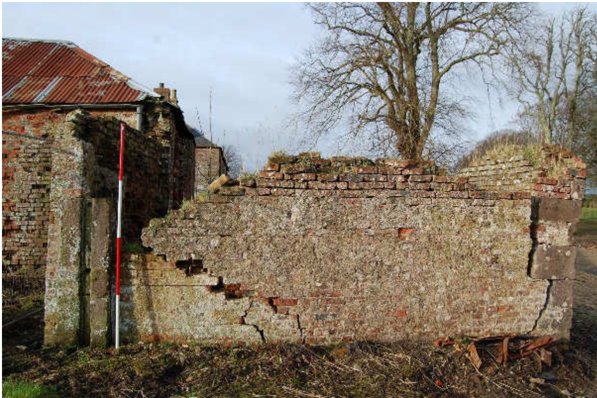
Illus 18 Building 2 Room 3 E wall showing gate post F60 (left); facing W
