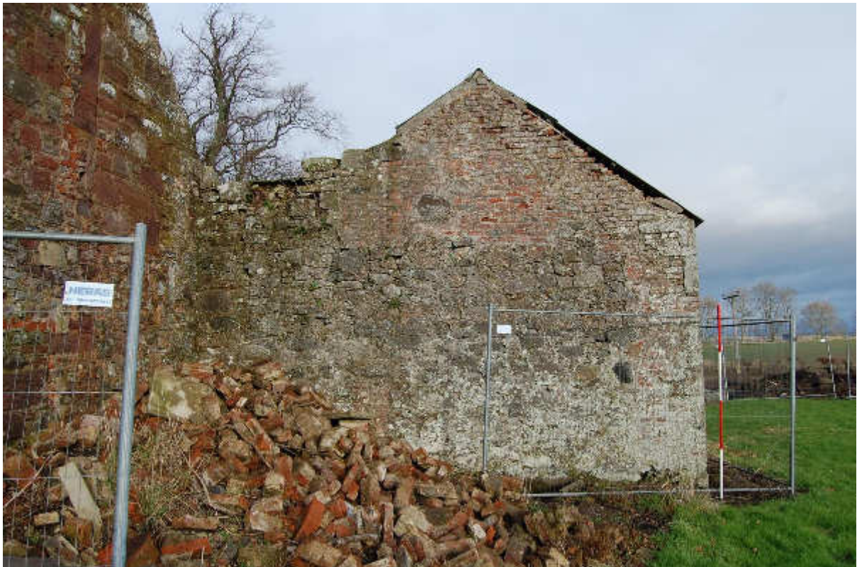
Illus 17 Building 2 s wall showing rebuilding in brick (top) and building scar F66; facing N
