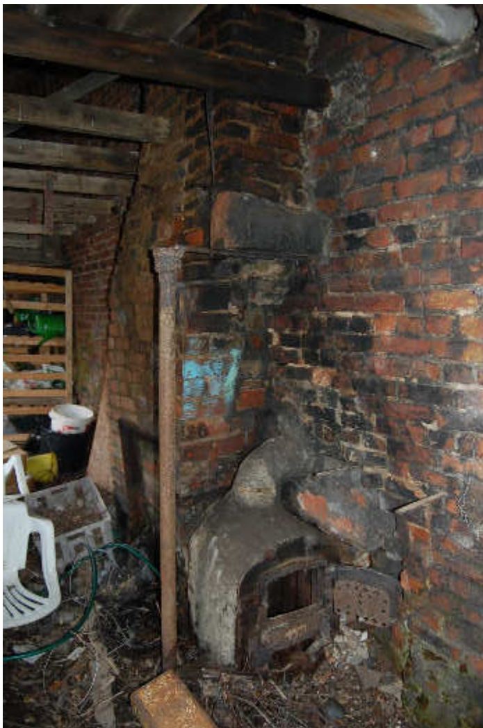
Illus 27 Building 4 interior with boiler F33 and flue F32; facing ESE
