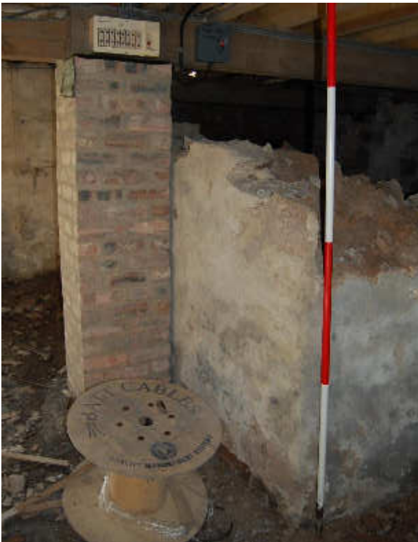
Illus 9 Room 4 NE corner of wall showing partially demolished wall (right), new wooden ceiling beams (top) and brick support for new ceiling (left); facing SSW
