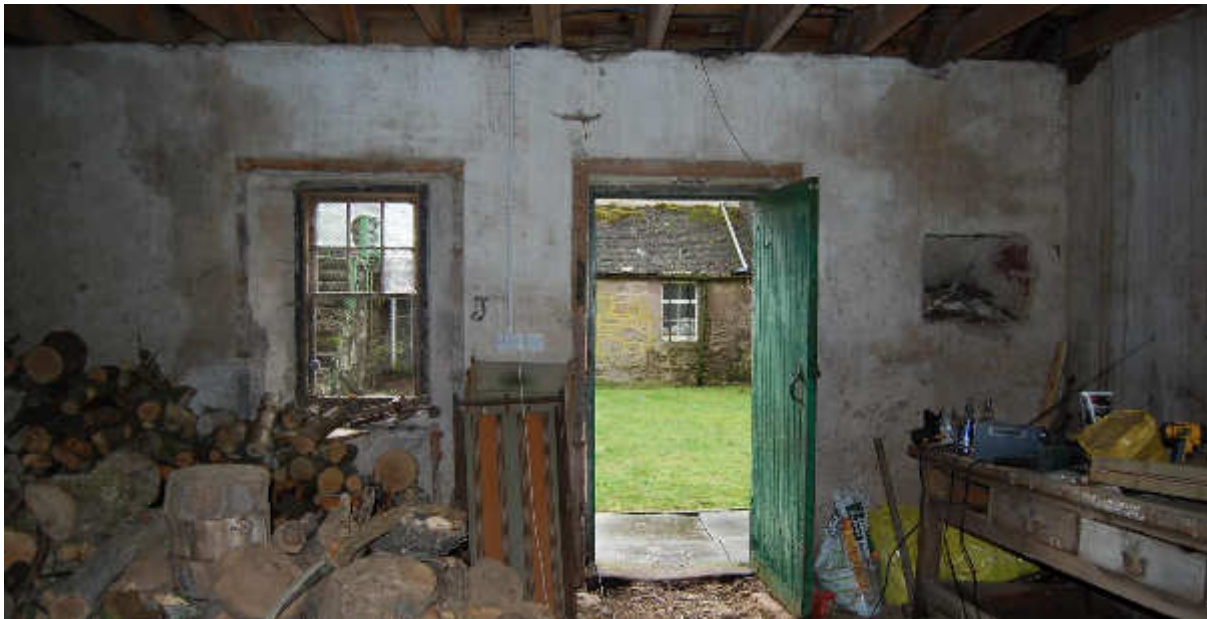
Illus 33 S wall Room 23 interior W63, D19, alcove F18 (L-R); facing S.
