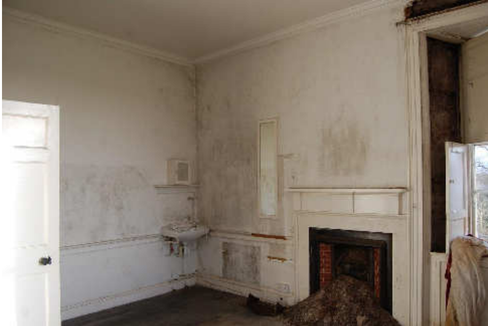
Illus 37 Room 28 NE corner showing coving and later fireplace (F8) set into earlier fireplace surround with W15 (right); facing NE.
