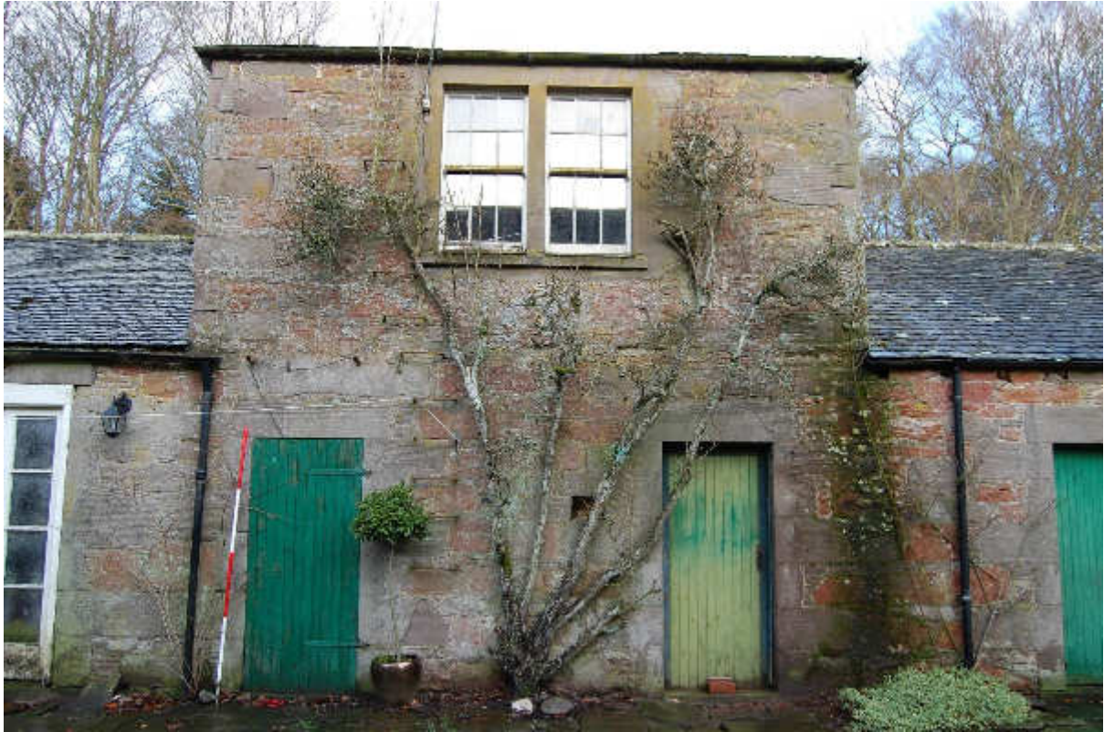
Illus 35 Room 24 S wall onto courtyard showing metal rung steps F24 (left of centre) and two lintels above each door (D17 left and D18 right) indicating that the height of the doors has been reduced and new lintels inserted.
