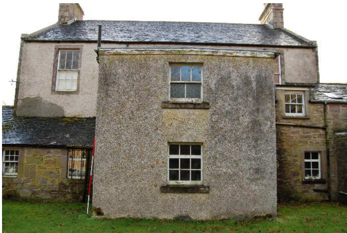
Illus 22 Room 16 N wall W28 (below) W25 (top) with Phase 1 house N wall at rear; facing S
