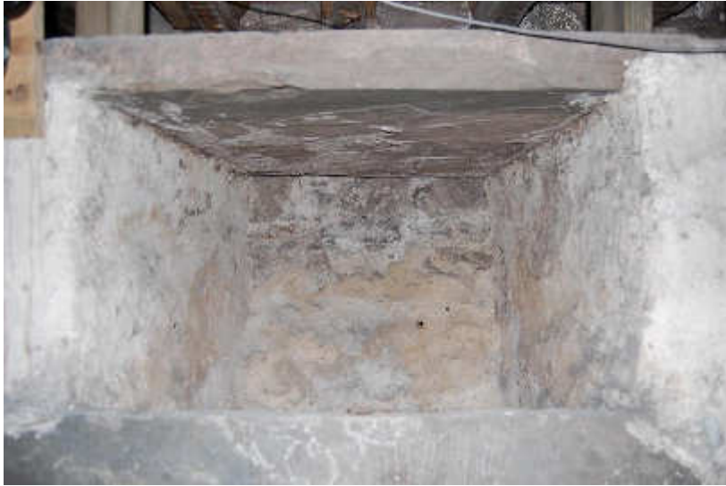
Illus 11 One of the upper alcoves showing sandstone shelf (top and bottom) and plastered masonry supports; facing N
