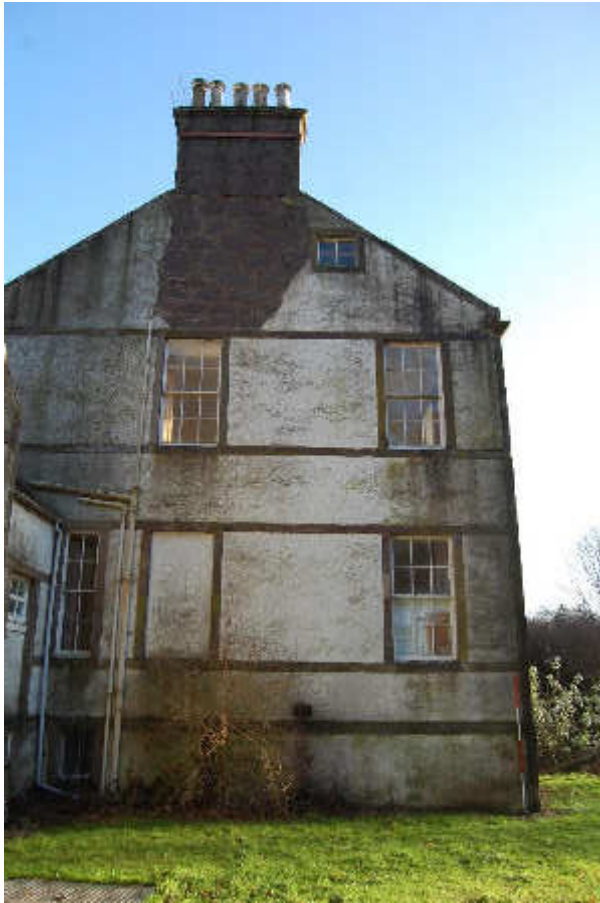
Illus 18 Phase 1 house W gable with Room 11 windows (W8, W9 blocked, W10 centre); facing E
