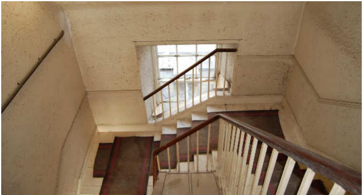
Illus 6 Stairwell F23 covers central window of Phase 1 house N façade suggesting the stairs were located elsewhere in Phase 1; facing N
