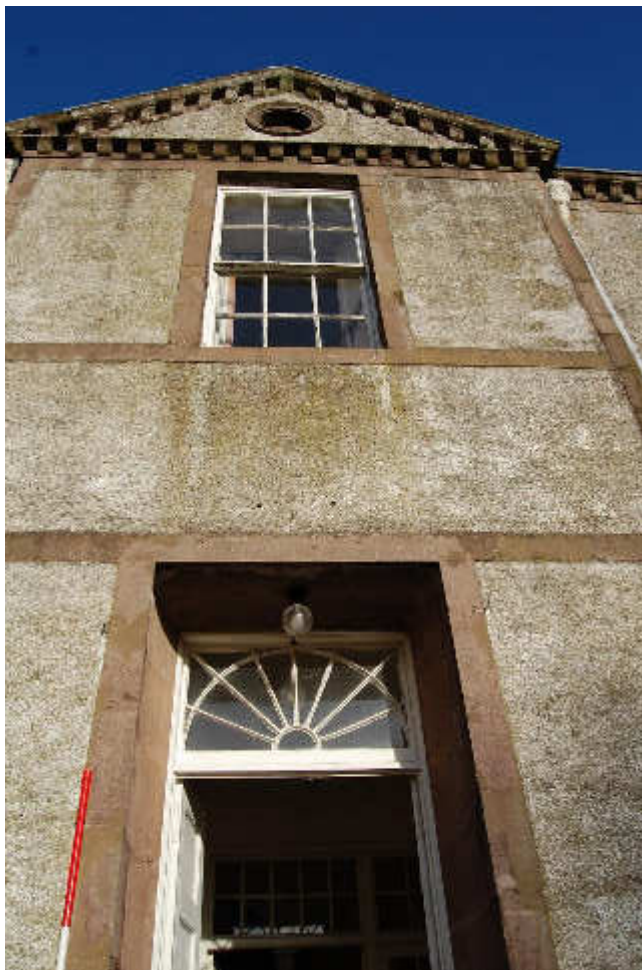
Illus 16 Phase 1 house S façade central door D2, W17 with roundel F2 (top); facing N
