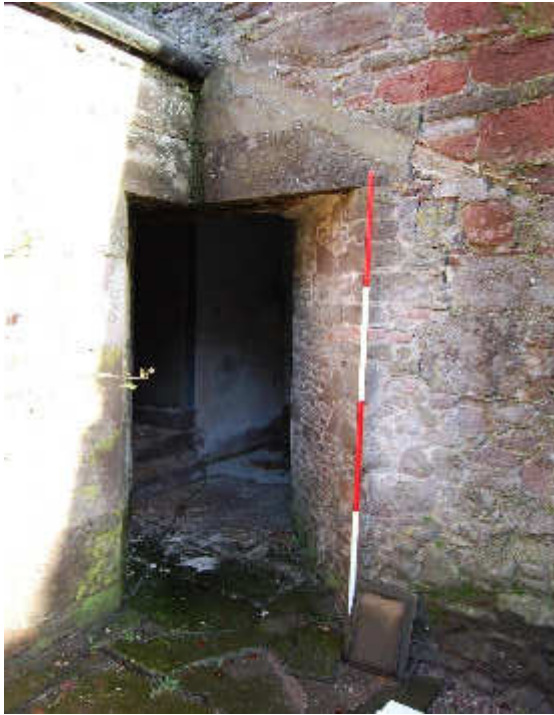
Illus 31 Door D20 a short stone-lined corridor through from the courtyard to the E wing rooms 21 and 22 showing scar of demolished structure (top right); facing NE.
