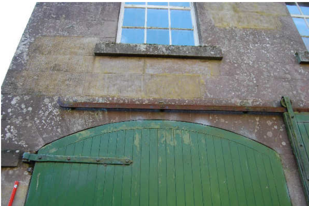
Illus 34 Detail of ashlar sandstone forming lintel of cart door D12; facing S
