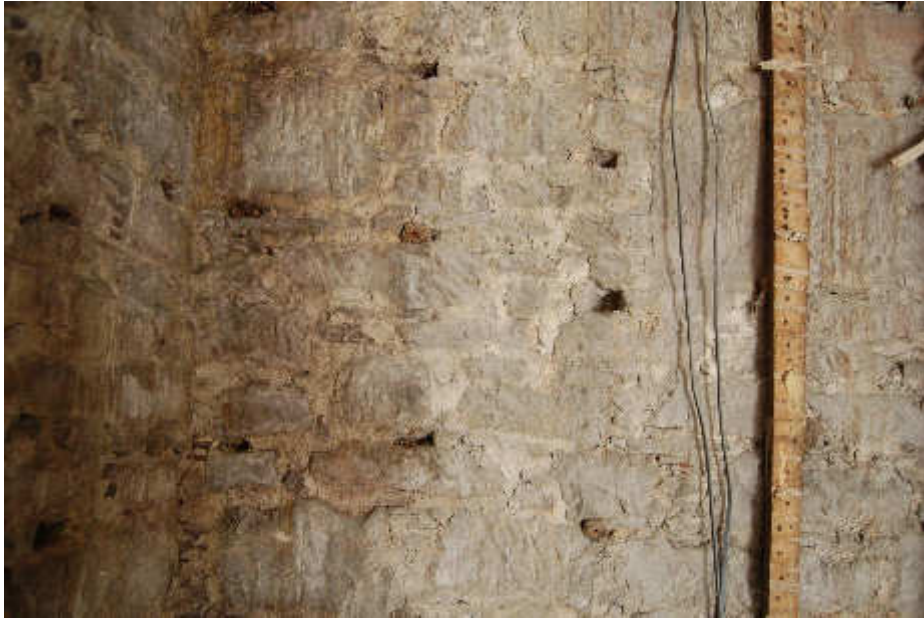
Illus 13 Detail of S wall Room 7 showing sandstone block and rubble construction; facing S
