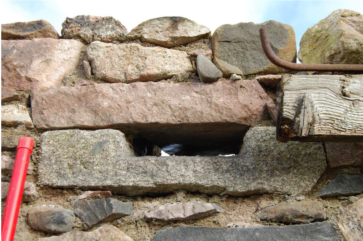
Illus 13 Room 4 S wall ventilation aperture F7, possibly a small first floor window lintel reused after re-roofing; facing N
