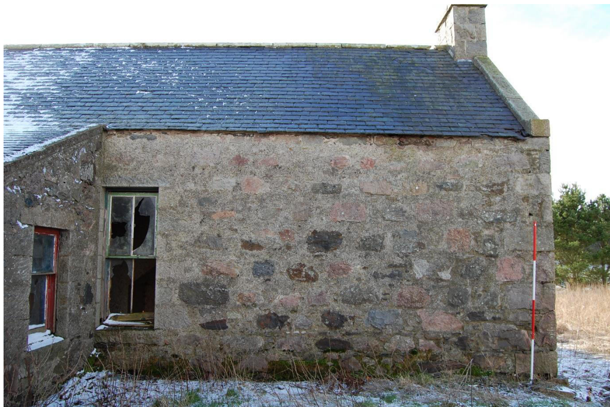
Illus 2 Building 1 Phase 2 lean-to extension (left) covering jamb of Phase 1 window W6; facing S
