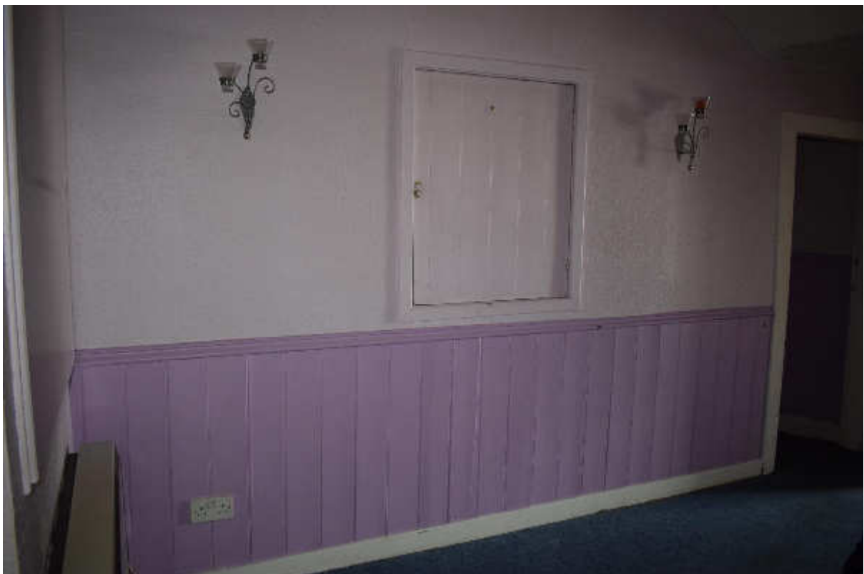
Illus 5 First floor window W67 originally an exterior window on NE wall Phase 1 building; facing W
