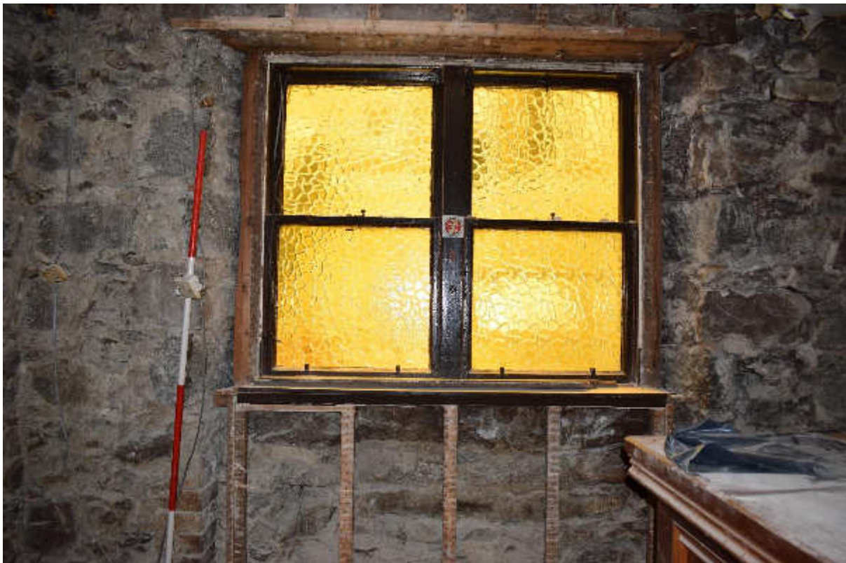
Illus 3 Blocked window W66 in the SW wall Phase 1 Room 26; facing SW
