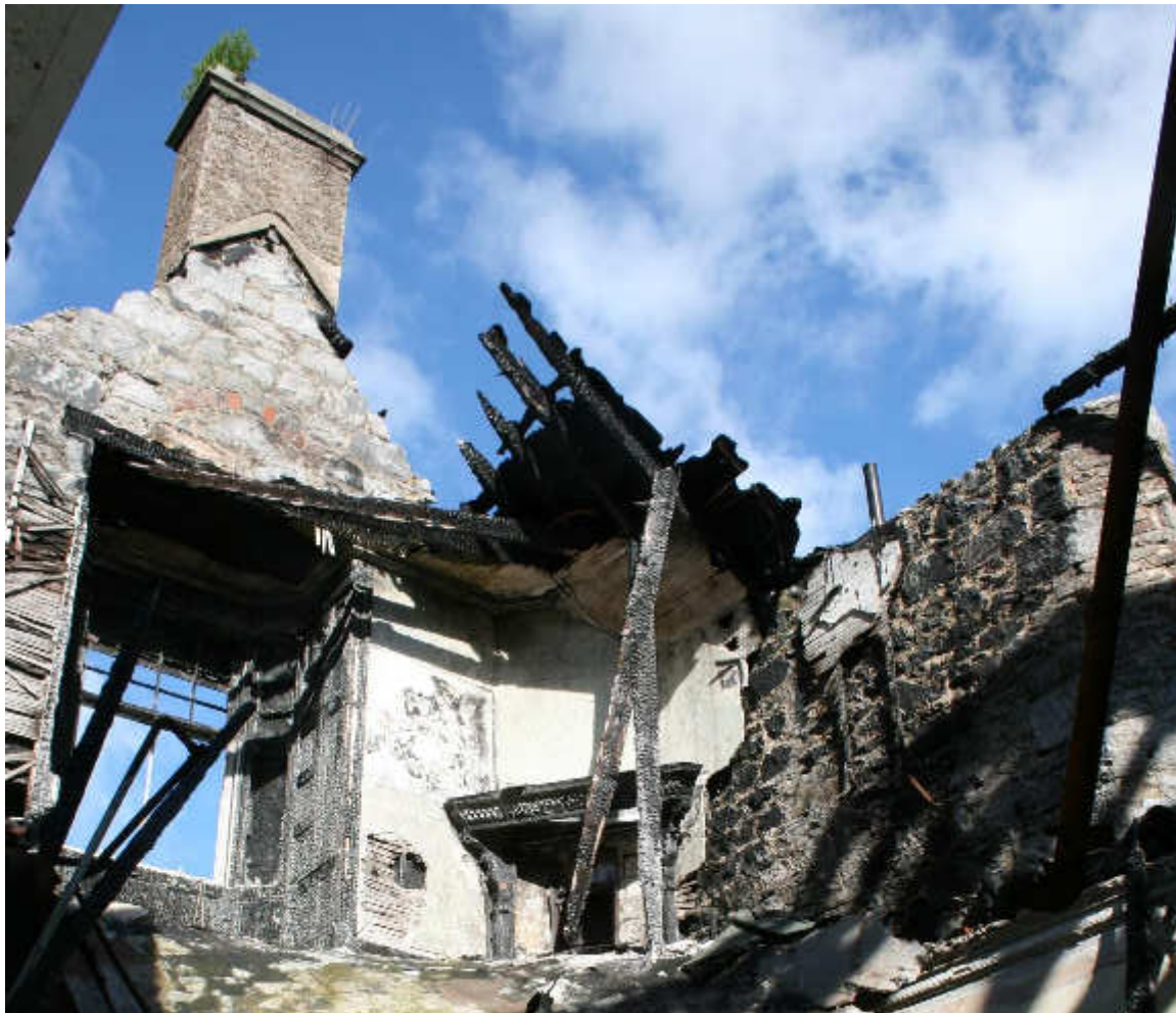
Illus 13 View into Building 1 first floor window W38 (left) and fireplace F6 (right); facing WNW
