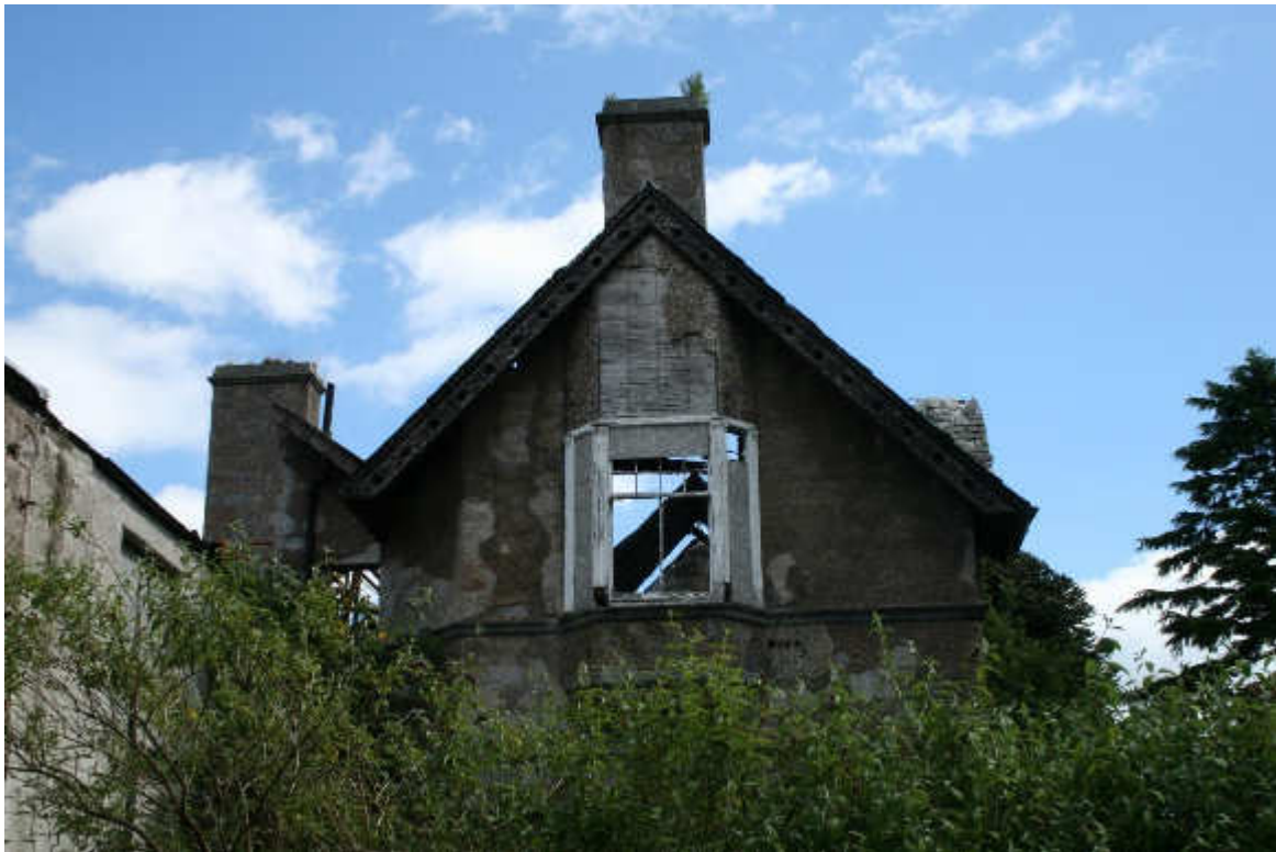
Illus 12 Building 1 W façade W38 with large pebble dash around over granite rubble construction and decorative pierced timber bargeboards above; facing E
