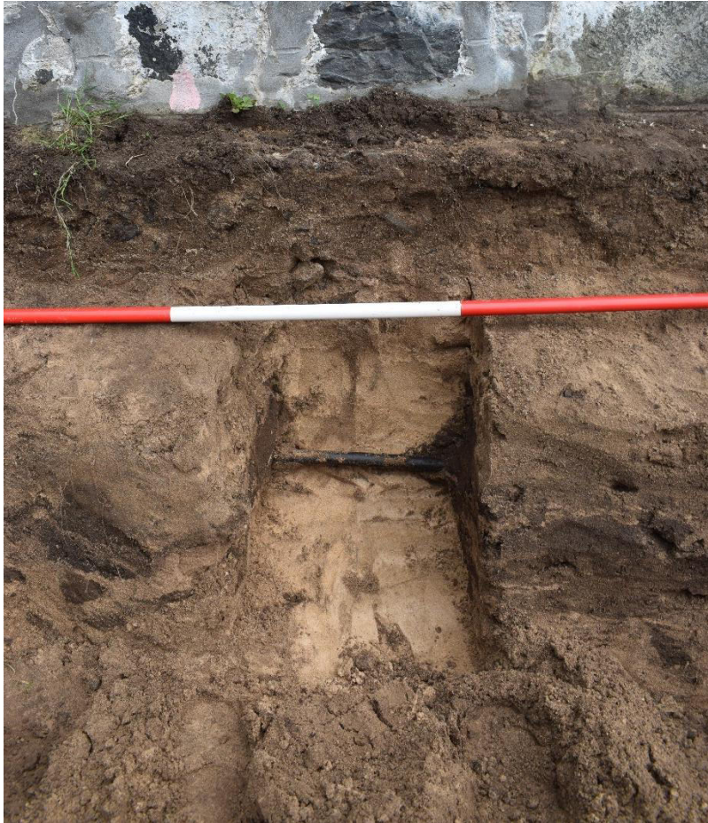
Illus 5 Phase 2 alkathene pipe trench 5, with 1870s cemetery wall and foundation (top); facing N
