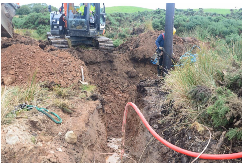
Illus 6 Insertion of new utility pole at eastern extent of project corridor. This particular pole required the most soil removal for completion while the remainder required substantially less ground disturbance.
