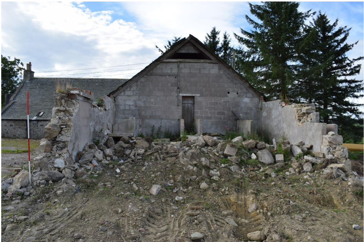
Illus 5 The interior of the demolished steading showing concrete lining, stalls and wall; facing S
