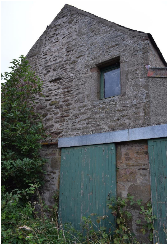
Illus 17 Room 6 W wall with D9 (bottom) and W10 (above, open); there are the remains of two windows which have been blocked and the new roofline cut through them, F3 and F4 (top). The original large sandstone quoins can be seen between the two green wooden doors; facing NE
