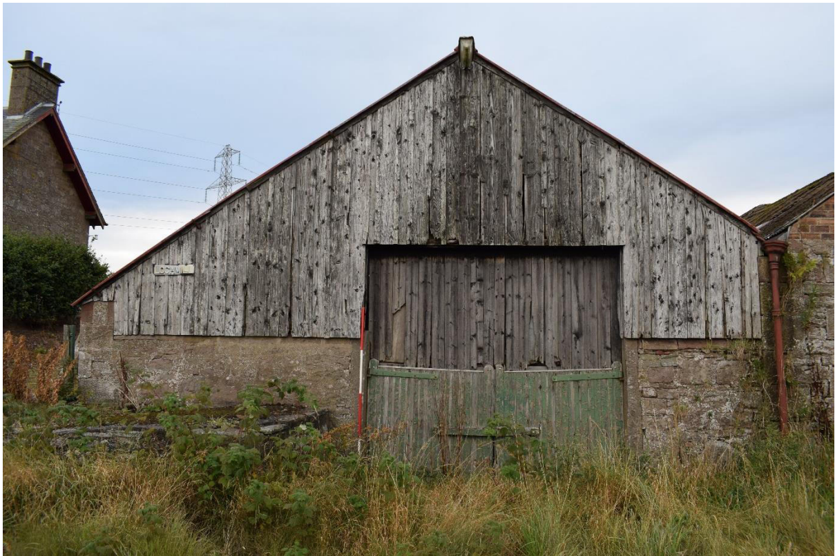
Illus 12 Phase 1 Room 1 S wall; this low wall originally surrounded a courtyard and was covered with wood and tin roof in Phase 2
