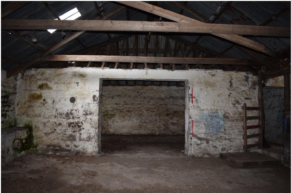
Illus 10 Phase 1 cart door D1 on S wall Room 3; the area in the foreground was an open courtyard surrounded by a low wall in Phases 1 and 2; facing NNW
