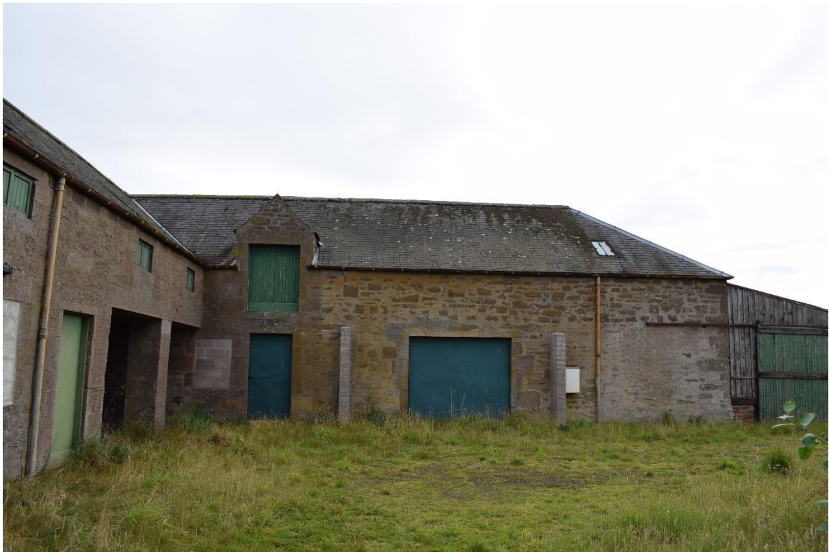
Illus 24 Phase 1 W wall Room 9 (right) with Room 8 and cart doors D21 and 22 (left); facing ENE
