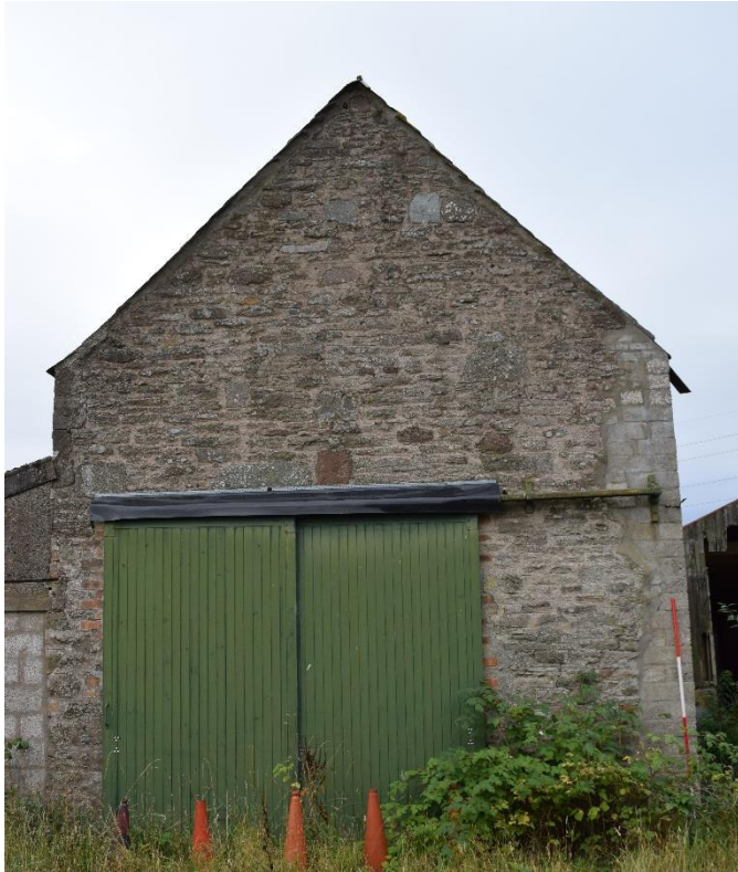
Illus 18 Room 6 E wall with D25; an extension on the N side of this building was removed in Phase 4 and the wall rebuilt with concrete bricks; this wall has been heavily rebuilt; facing WSW
