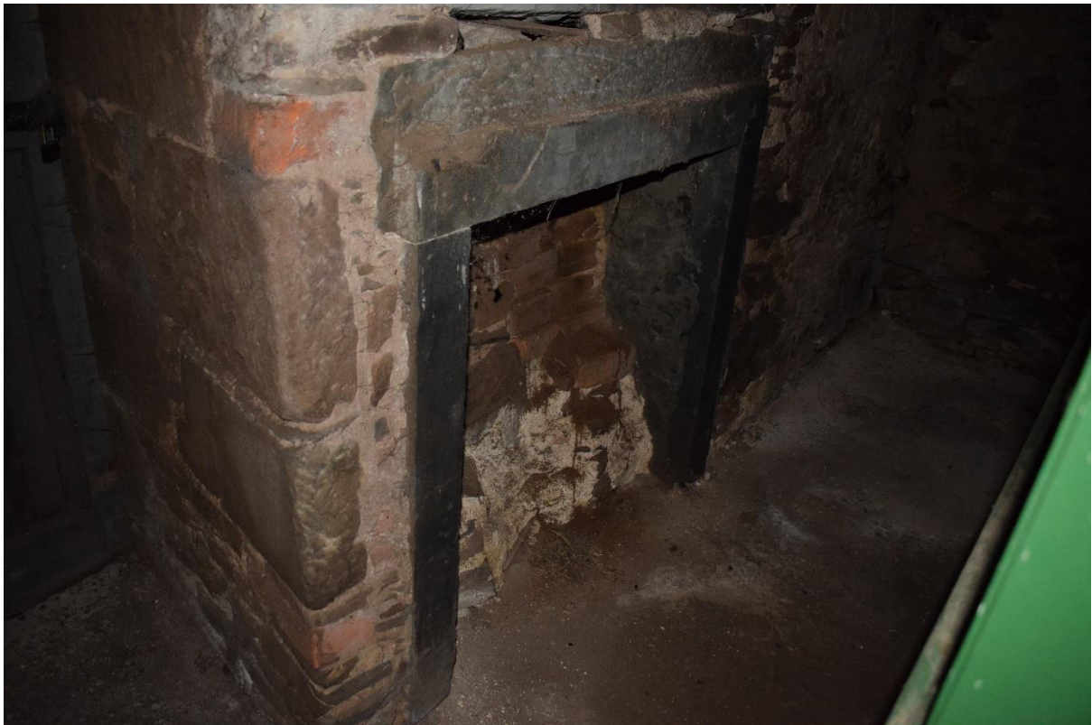
Illus 21 Room 6 W wall fireplace F1; there was poor access to this room; facing NW
