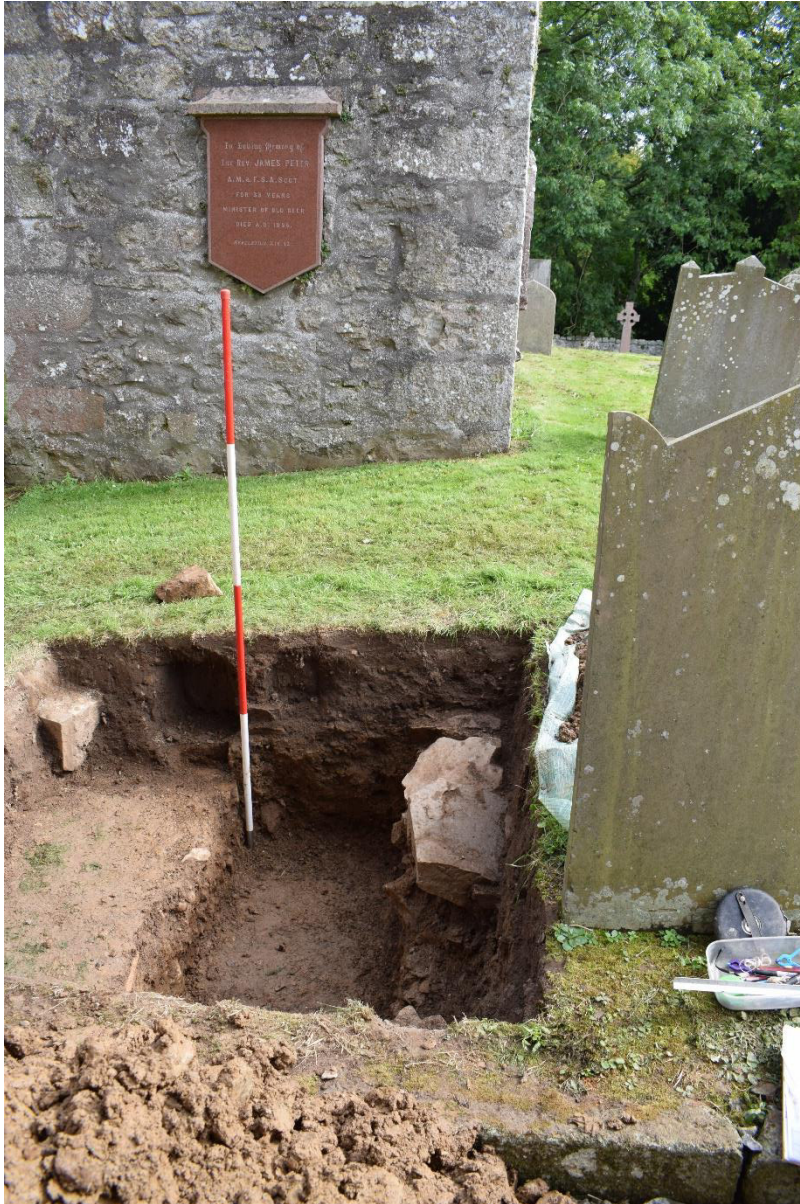
Illus 17 Trench 6 wall foundation 64 in line with S wall of medieval church, robbed out by grave cut 66; facing E
