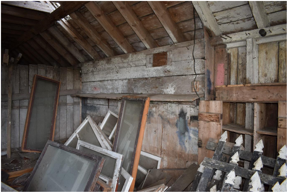
Illus 9 Building 1 interior S wall of W room from D7 showing repairs and alterations; facing SE
