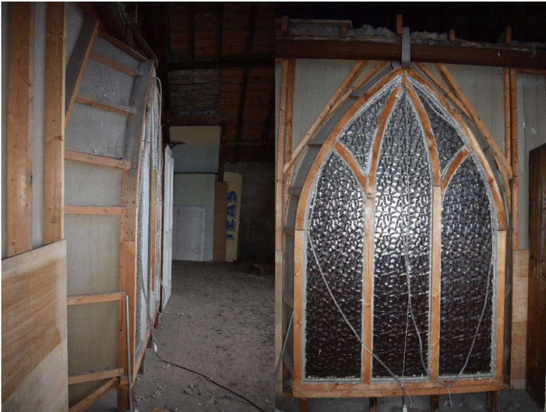
Illus 19 W23 built into the Phase 2 first floor partition to allow light from the main W window W6 into the church; left facing SE. right facing ESE
