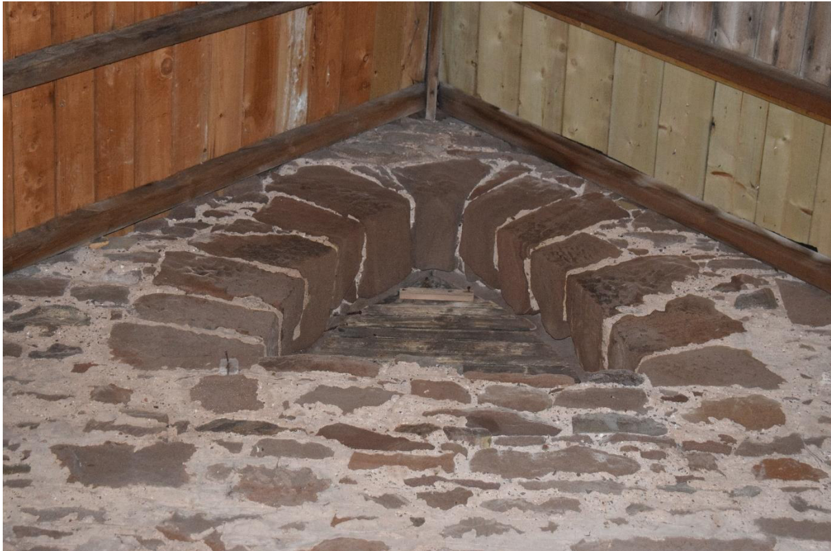
Illus 13 Phase 1 small window W5 (later blocked) in the top of the W gable; facing WNW
