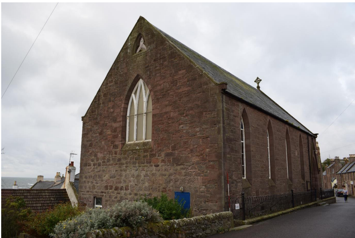
Illus 17 ESE gable showing repointing of lower section with W20 (top), W6 (centre) and small window W22 and D3 (below); facing SW
