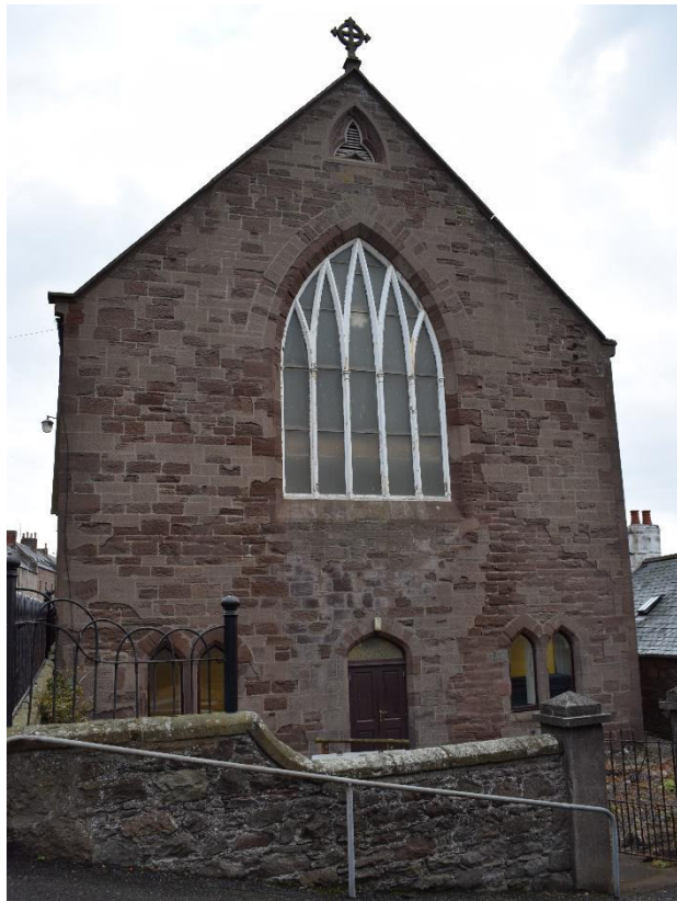
Illus 8 WNW gable with stone celtic cross finial (F11, top) small window W5, main window W6 and basement floor access door D2 with W7 (left) and W8 (right); facing ESE.
