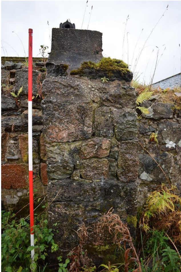
Illus 9 Stone plinth F1 built after blockage of D3 to support concrete block and metal shaft; facing SSE
