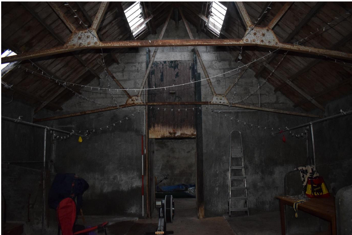
Illus 10 Room 4 SSE wall showing reroofing and conversion for dairy; facing SSE
