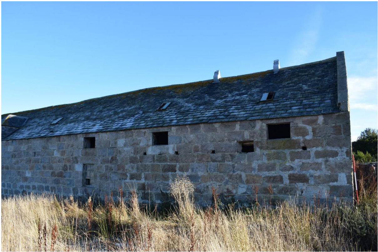
Illus 4 Building 1 W wall W1 (right), W2, W3, W5 (left); facing ENE
