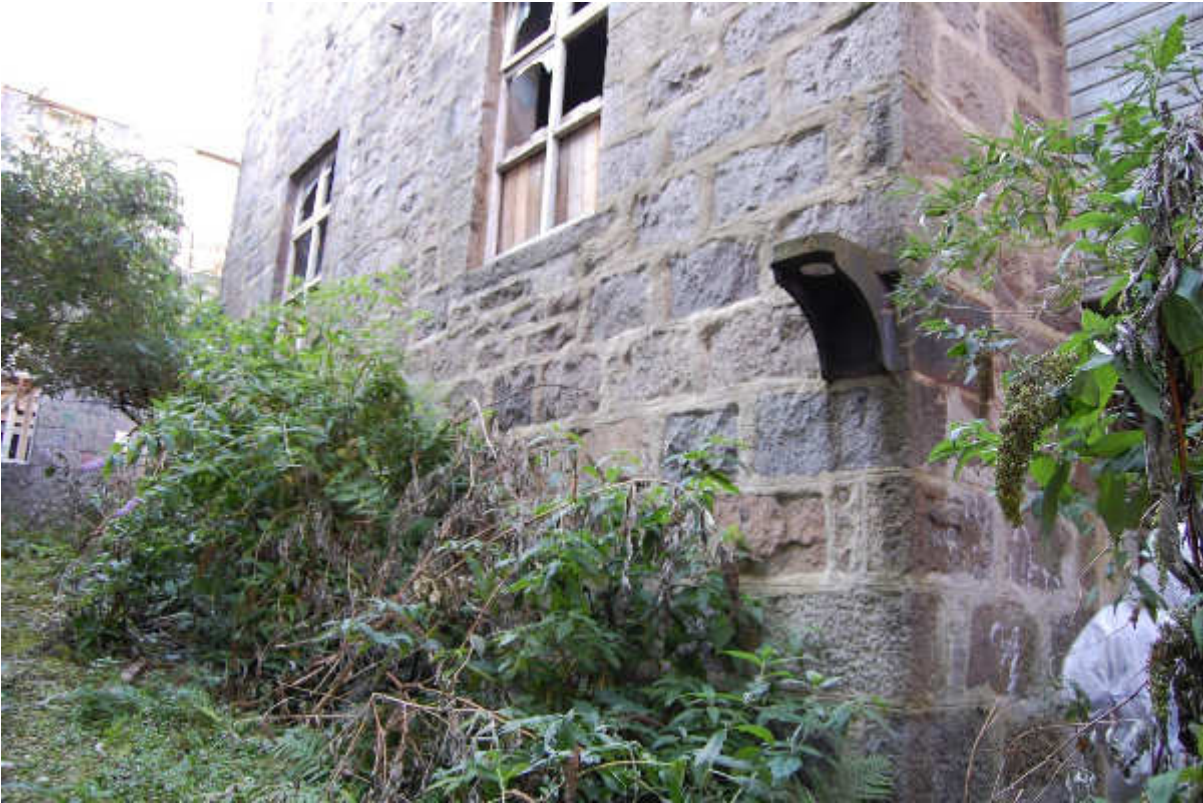
Illus 38 Building 26 SSE gable W26/2 (left) 26/3 (right) and cast iron bracket F28 (bottom right); facing NW
