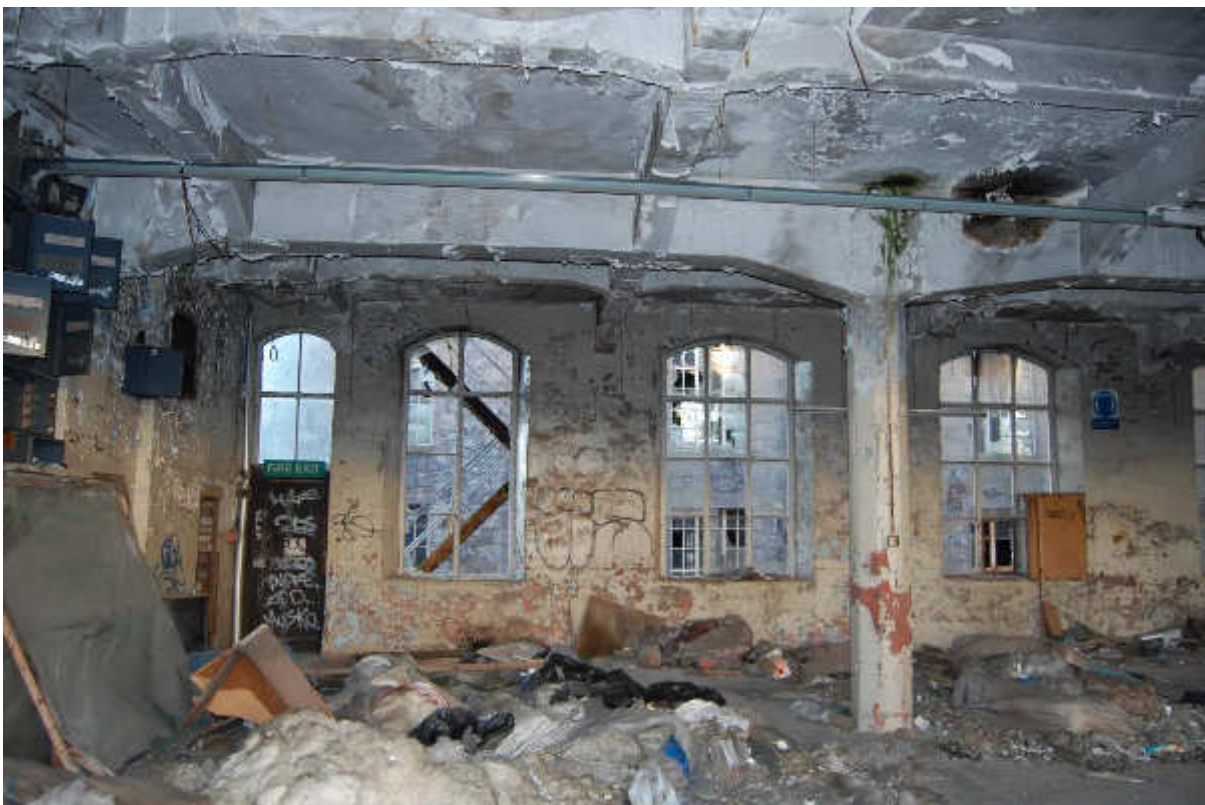
Illus 32 Building 21 2nd floor E wall windows W21/8, 9, 10, 11, 12 (L-R) with concrete octagonal pillar and concrete roof; facing ENE
