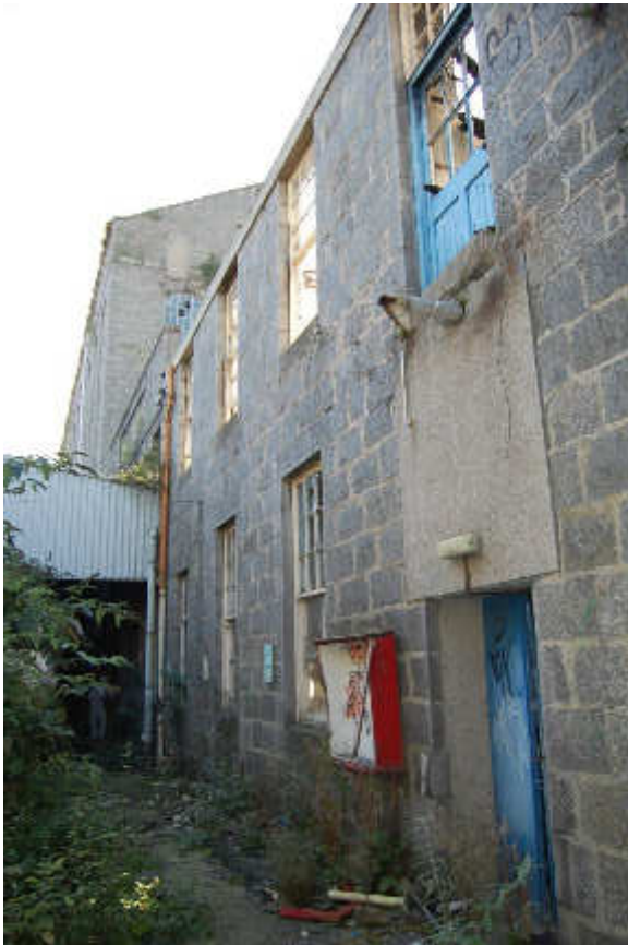
Illus 43 Building 30 ENE wall with Building 26 (left) and metal roof of post-1980s loading bay Building 29 (left centre); facing S
