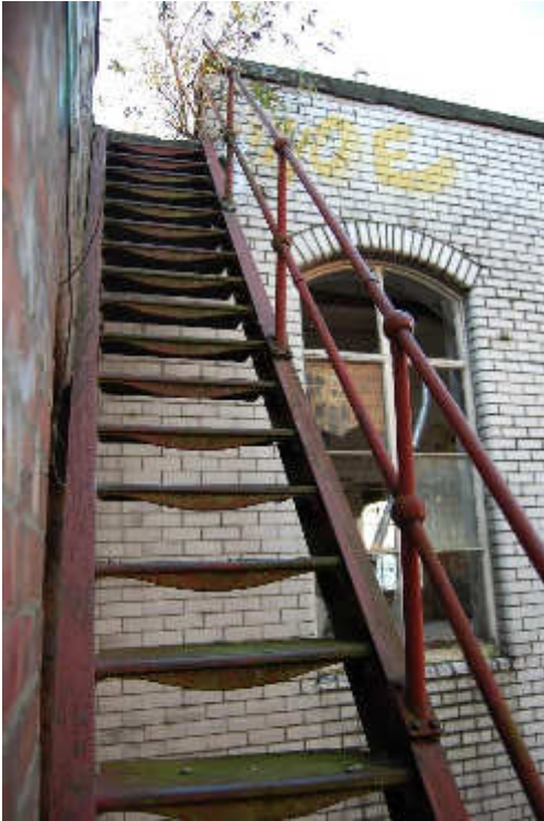
Illus 29 Building 21 E façade cast iron stairs to roof (F53) and detail of window W21/14 clad with white brick; facing W
