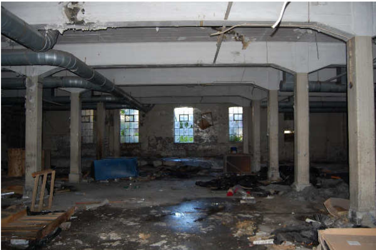
Illus 100 Building 83 (1910) ground floor showing concrete square-sectioned pillars, concrete floor and roof; facing WSW.
