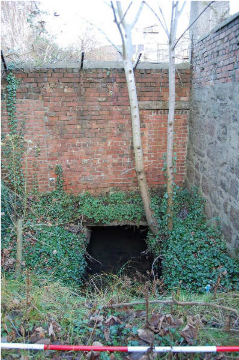
Illus 147 Culvert F41 with N brick boundary wall with Hutcheon Street (centre) stone E boundary wall (right) with blocked apertures DHS/2 (left) and DHS/1 (right) and low blocked aperture in between; facing NNW
