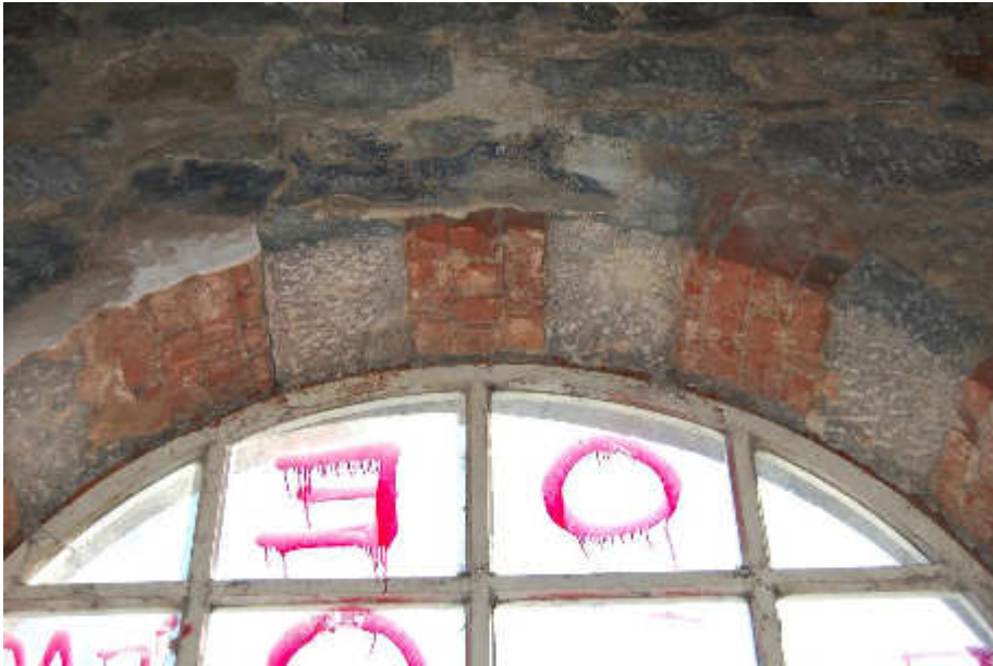
Illus 51 Building 32 4th floor window W32/17 showing stone and brick detail; facing NNW
