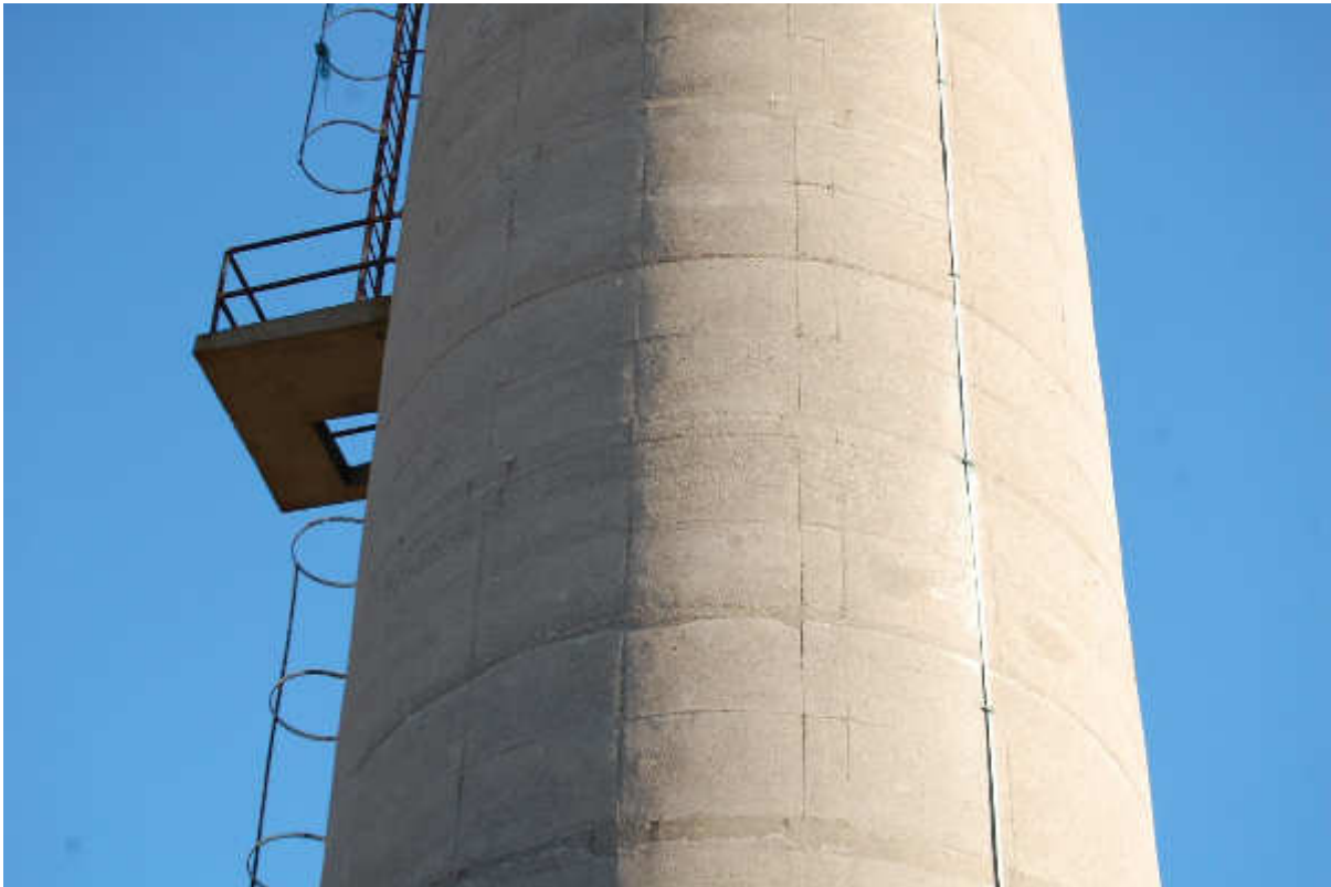
Illus 129 Detail of concrete chimney Building 98 showing poured concrete sections, external ladders and platforms
