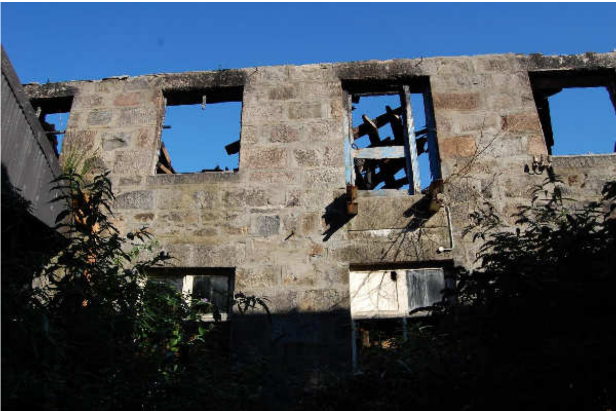
Illus 39 Building 26 W wall showing fire damage with W26/9, /10, D26/1, W26/12 (top L-R) and W26/16, /17 (bottom L-R); no access so far; facing E
