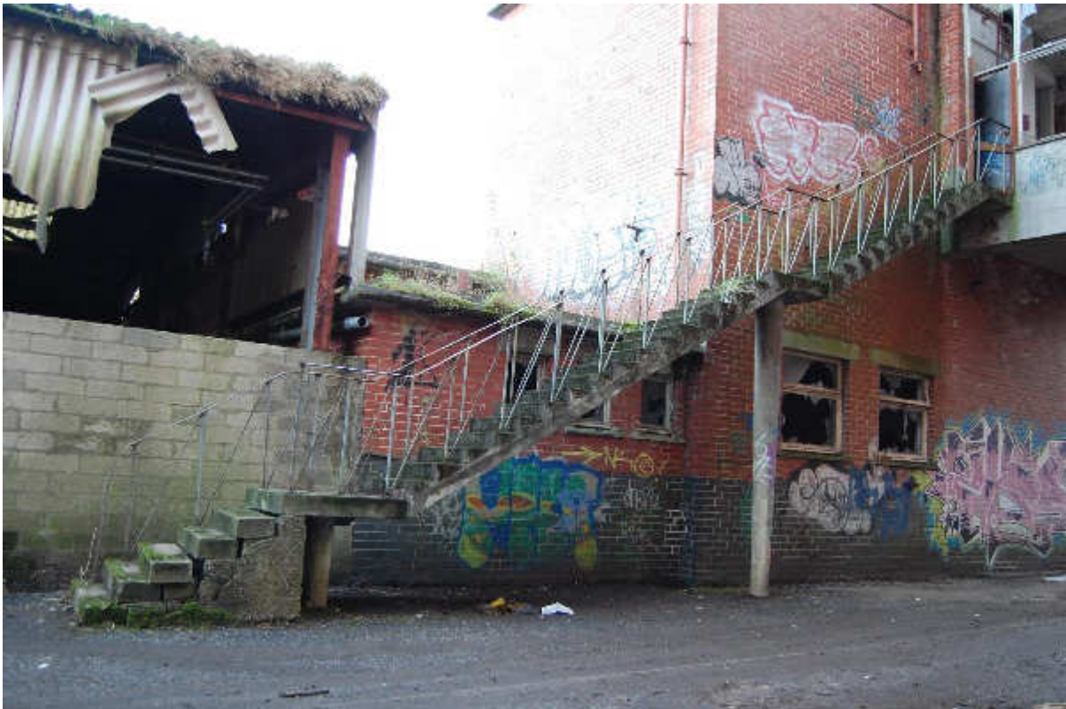
Illus 148 Concrete steps to Building 100 (top right) along W wall Building 99; facing NE
