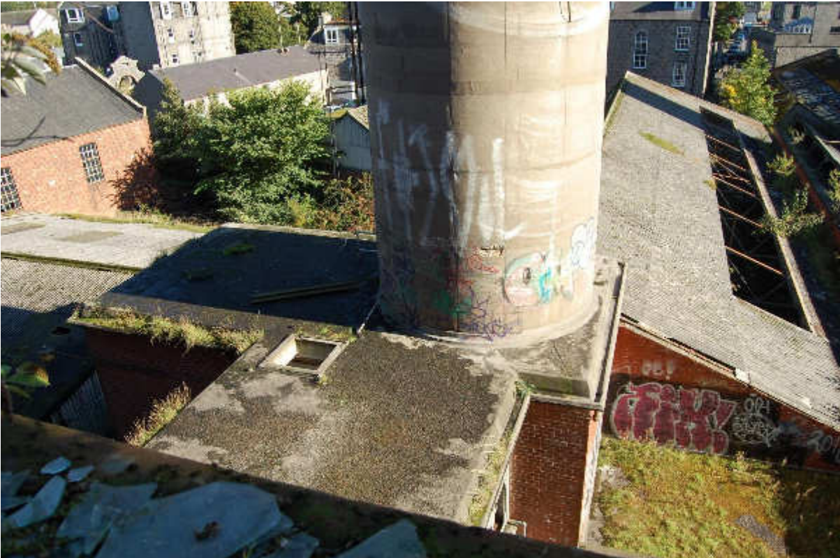
Illus 131 Base of concrete chimney Building 98 from 2 nd floor Building 86; facing ENE.
