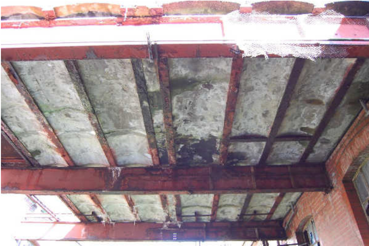
Illus 112 Gantry Building 87 underside showing street structure with concrete infilling between; facing NW.
