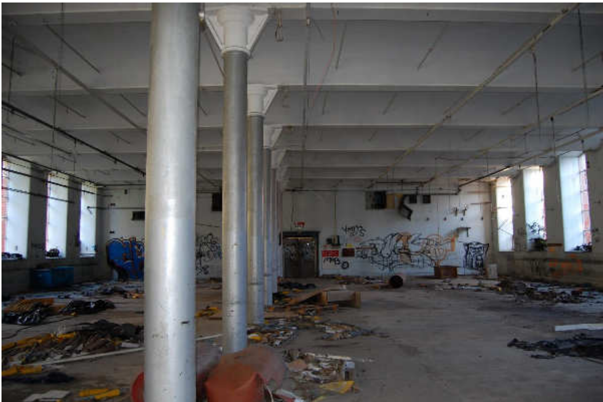
Illus 105 Building 84 ground floor showing cast iron pillars and roof; facing NNW
