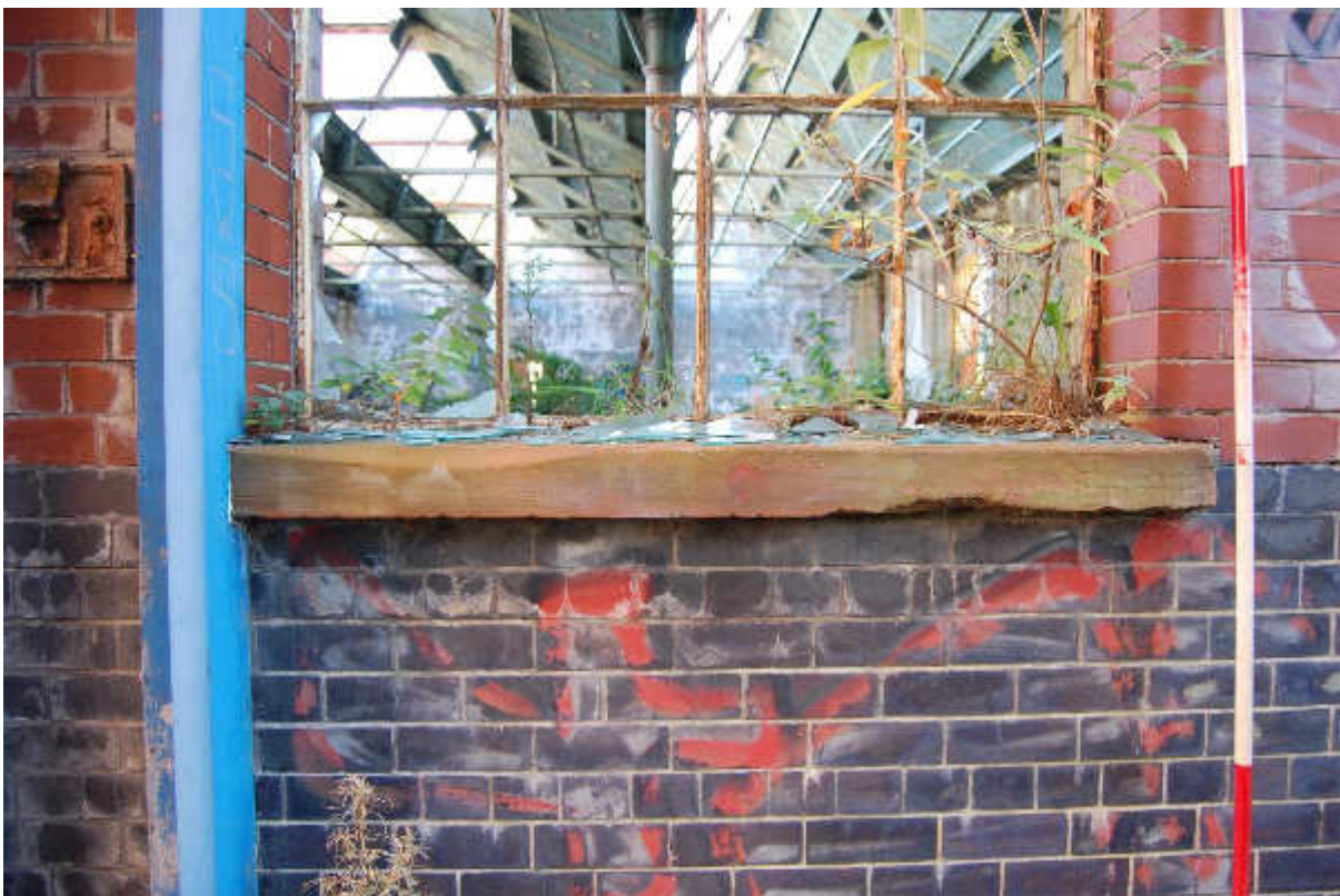
Illus 114 Detail of Building 90 window with sandstone sill and grey bricks below and red brown above; facing NE
