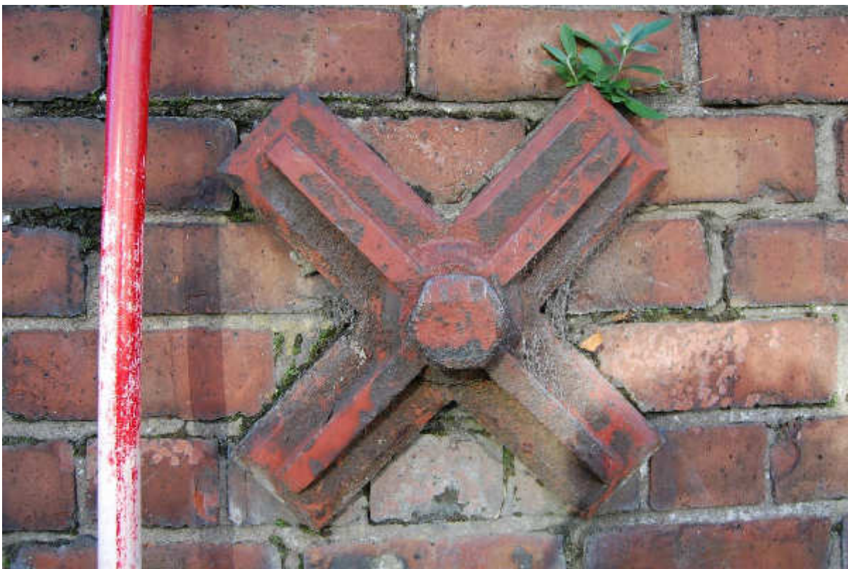
Illus 152 One of four horizontal prop heads with hexagonal bolt head F64; facing S
