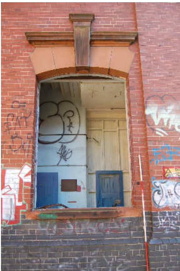
Illus 103 Building 84 W84/1 showing reddish brown sandstone sill and lintel details and two colour brick wall; facing ENE
