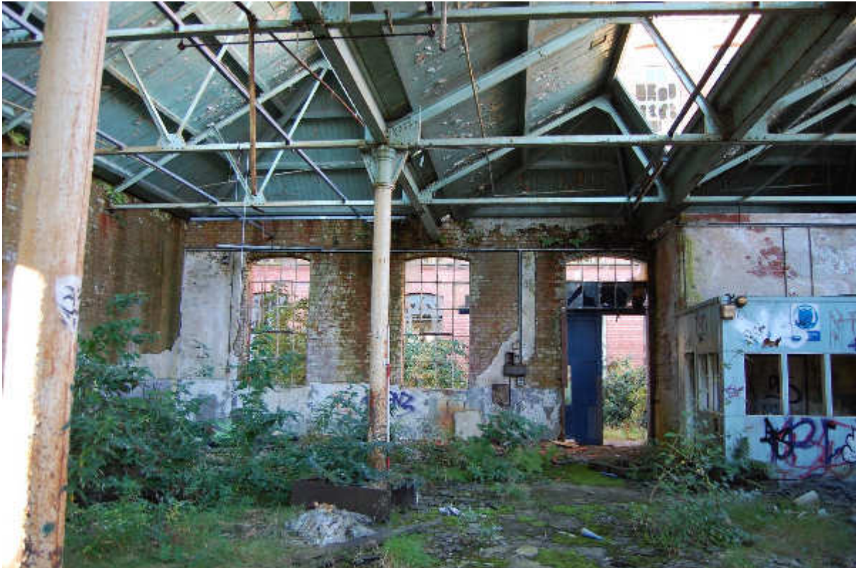
Illus 115 Building 90 interior SW wall showing cast iron pillars and roof beams with more recent replacement roof; facing SW
