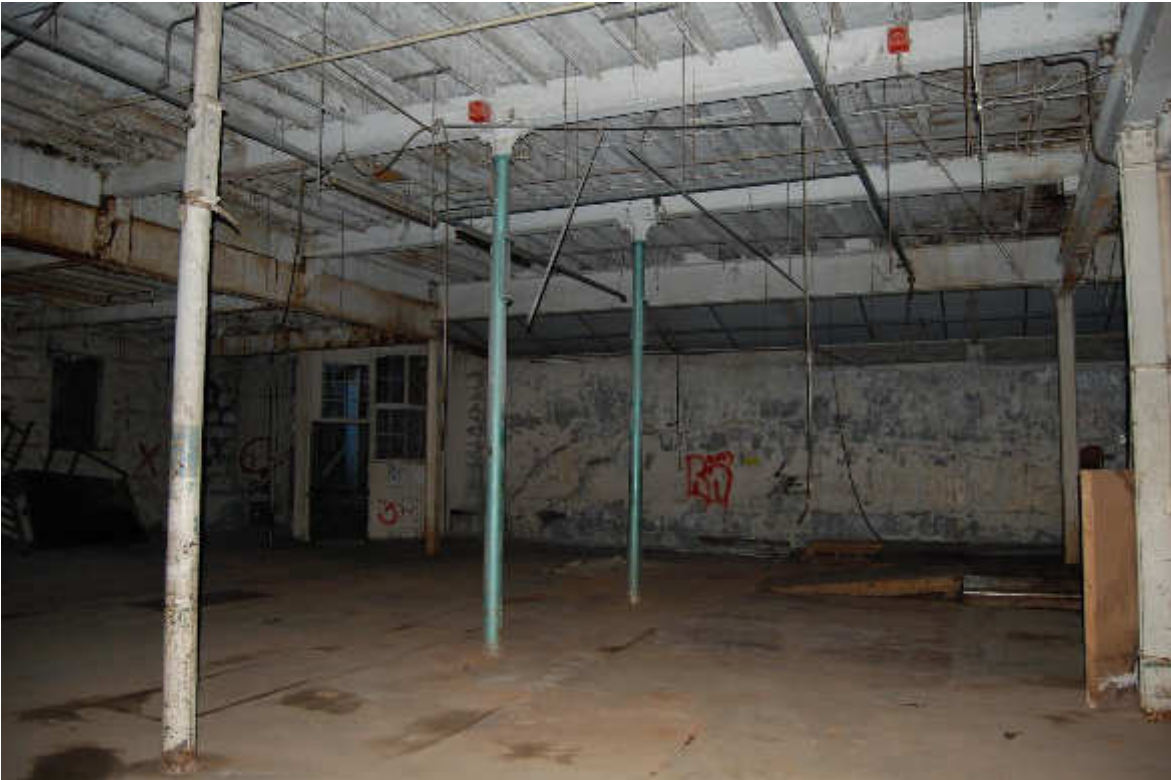
Illus 70 Building 51 interior showing round cast iron pillars, newer concrete wall (right) and replacement ceilings; facing SE
