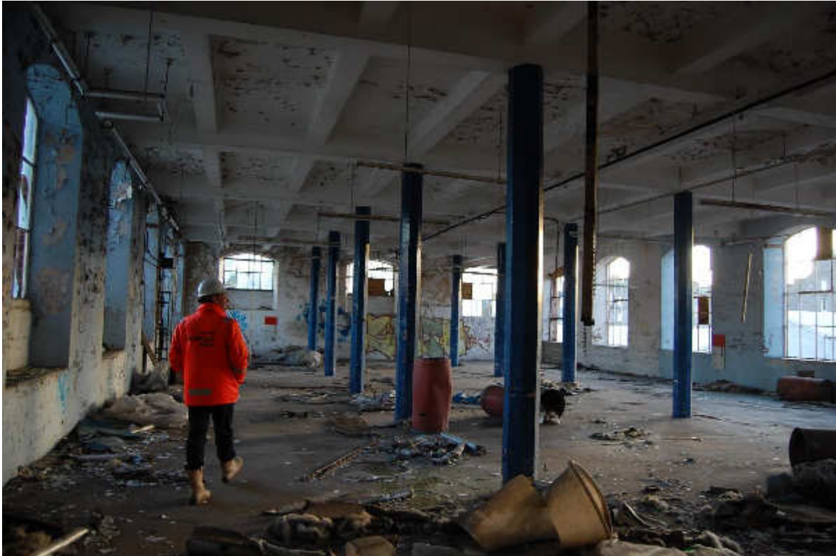
Illus 33 Building 20 3 rd floor showing concrete octagonal section pillars and concrete ceiling; facing SSE
