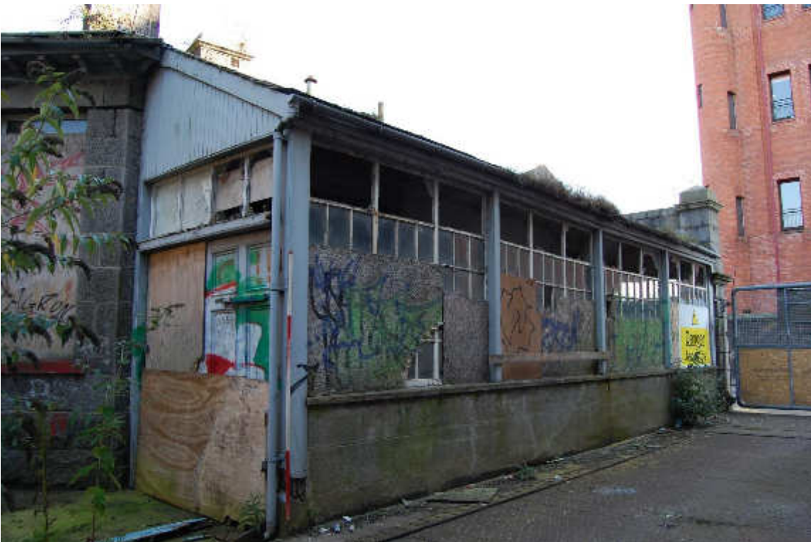
Illus 11 Building 1A cast iron and wood lean-to extension, gate F46 lead through this building which was presumably the main employee entrance leading into complex; facing SSE
