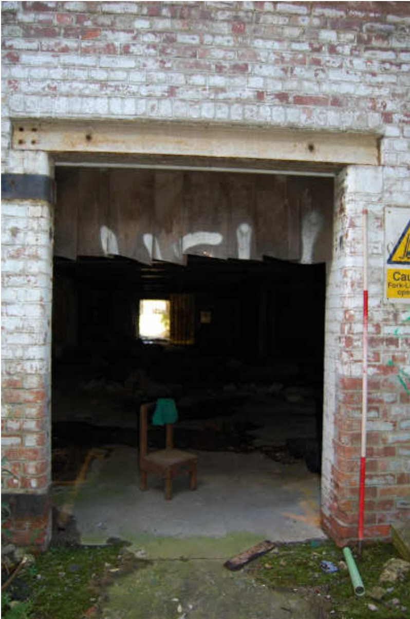
Illus 65 Building 47 N wall door D47/1 showing steel beam lintel with brick above and bullnose bricks used for rounded corners for jambs; facing SSE
