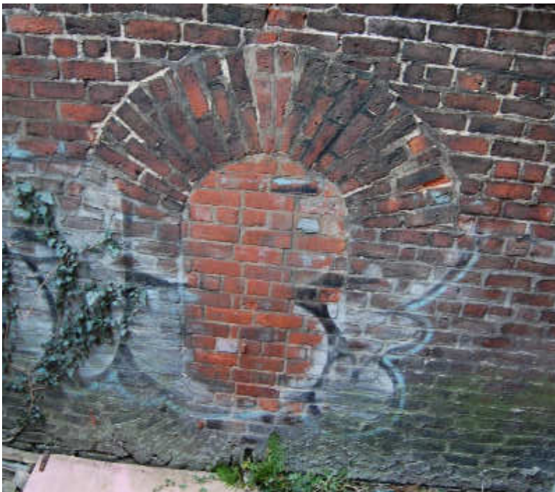
Illus 80 Building 53 stoke hole/door D53/1 in base of chimney Building 53 W face; facing E
