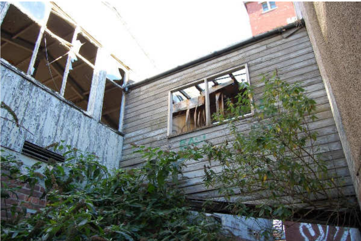
Illus 67 F21 wooden walkway between Building 51 (left) and Building 47 (right); facing ENE
