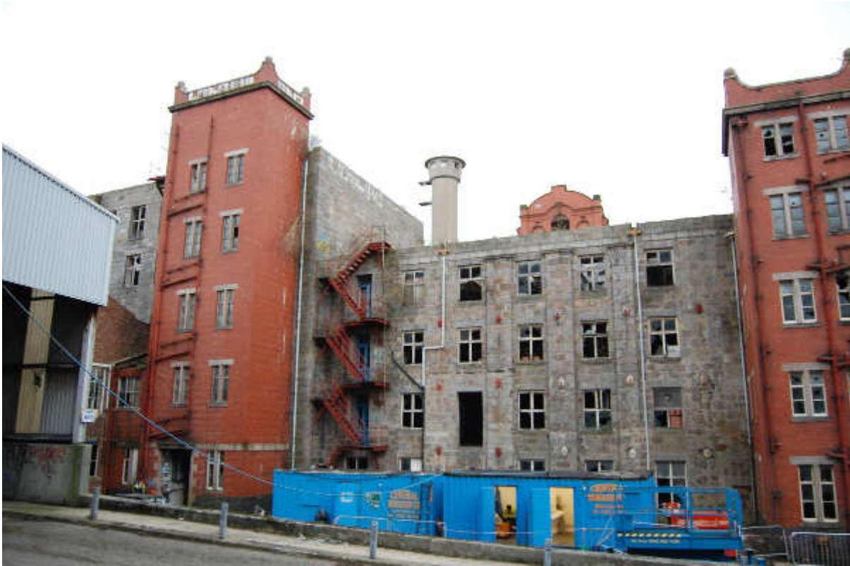
Illus 62 Building 45 (centre) W façade with brick extension B48A (left) and B44 (right); facing NE
