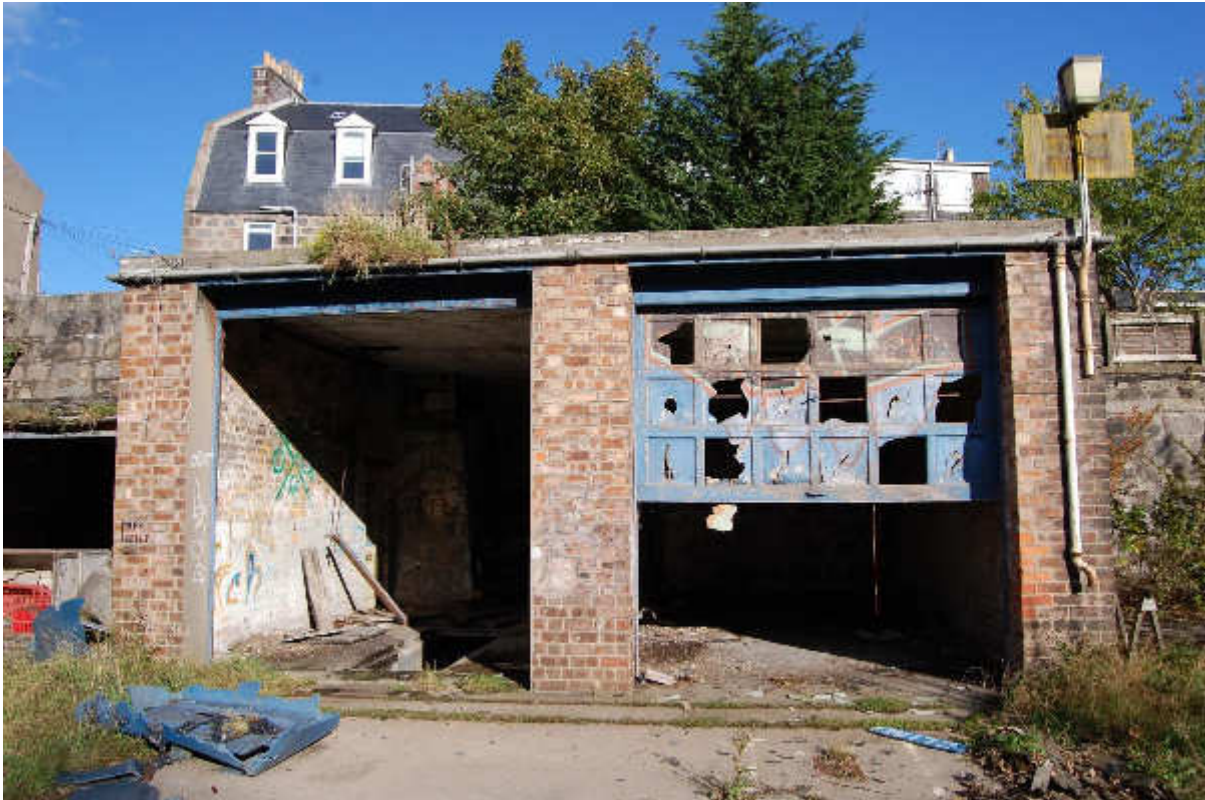
Illus 126 Building 95 garage with inspection pit at E edge of site; facing ENE
