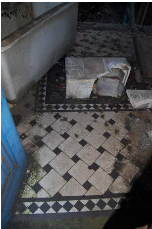
Illus 83 Interior Building 54 entranceway at N of building to be recorded more fully once building is empty; facing S
