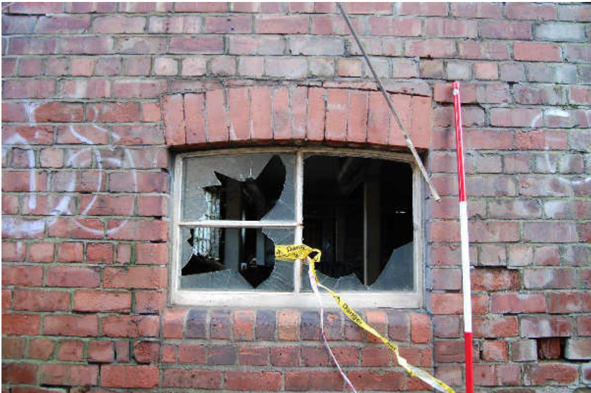
Illus 97 Window 83/12 showing arched brick lintel, bullnose brick sill and infill below of former door; facing N
