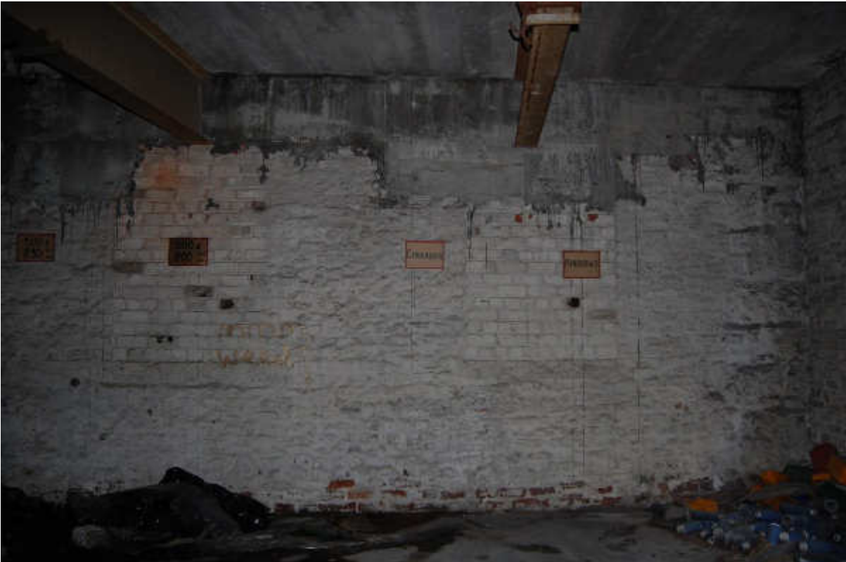
Illus 66 Building 47 W wall with blocked windows W47/3 (right) and W47/2 (left); facing WSW
