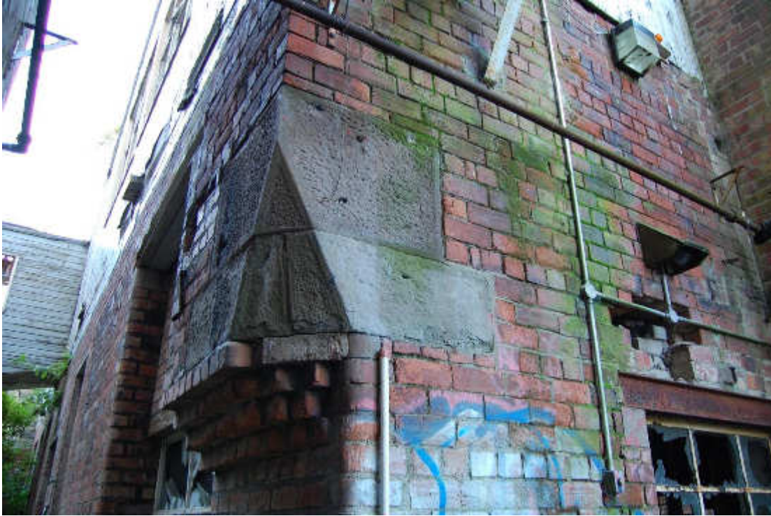
Illus 69 Building 51 SE corner showing sandstone and bullnose brick corner detail; facing WNW
