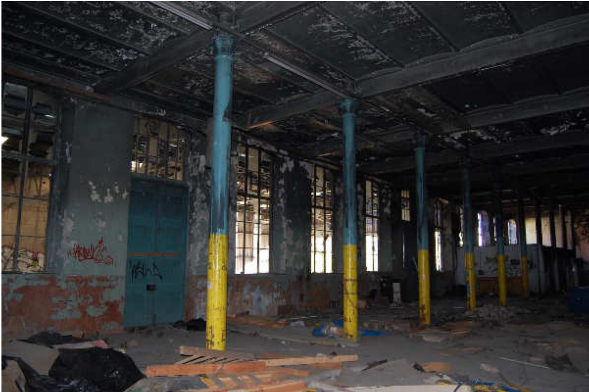
Illus 47 Building 32 ground floor interior E wall showing round cast iron pillars and beams; facing SE
