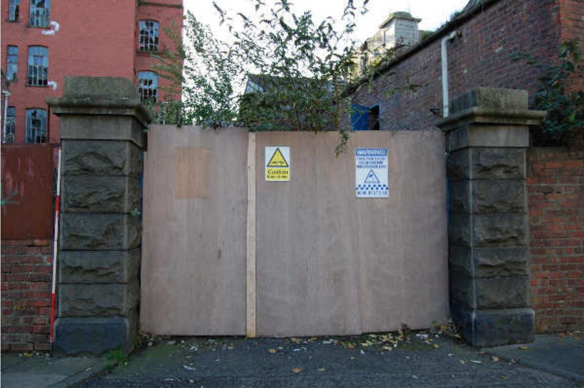
Illus 146 F34 Hutcheon St gate with rusticated granite gate piers; facing S
