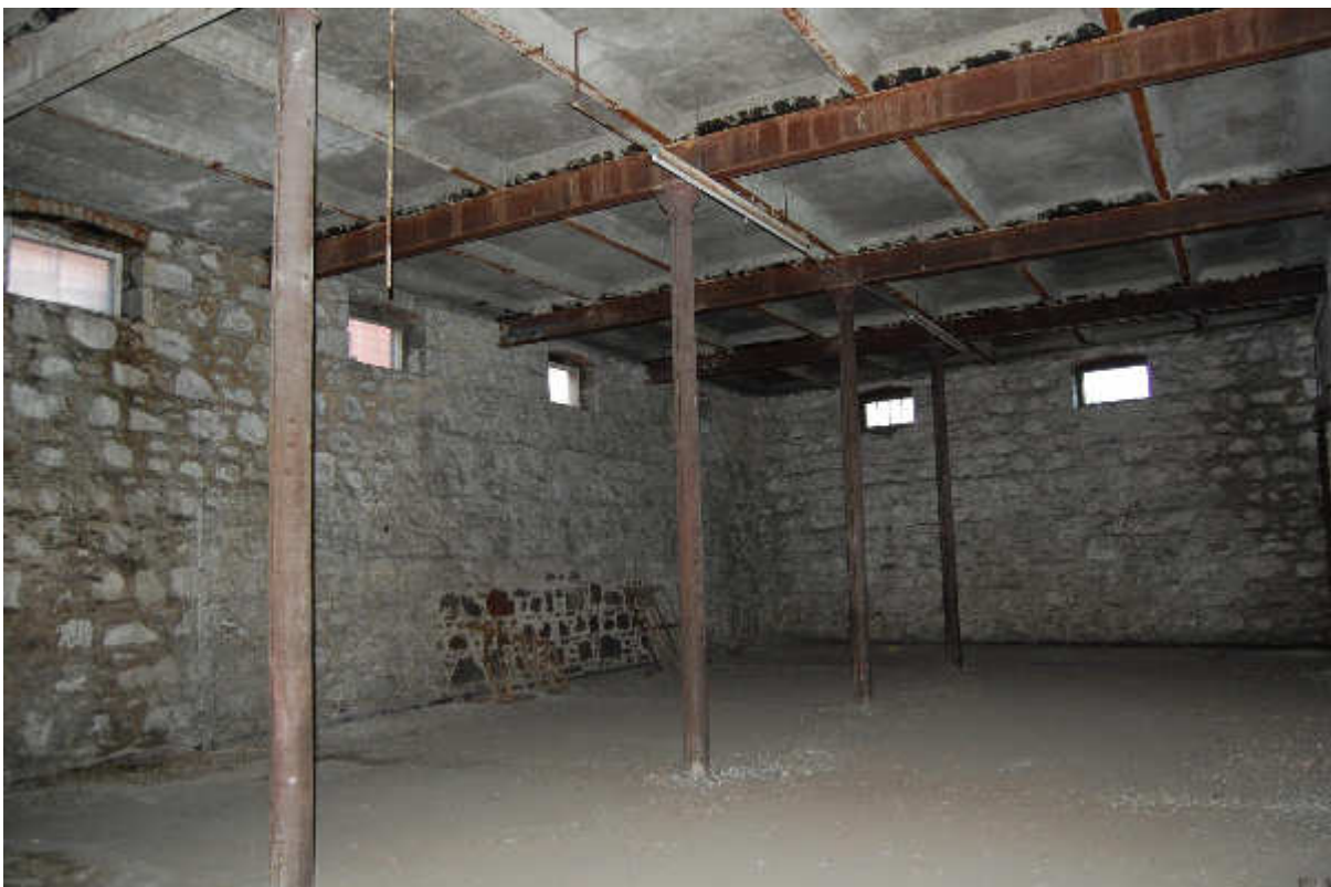
Illus 18 Windows W5/17, 18, 19, 20, 21 (R-L) interior showing brick relieving arches, cast iron pillars and beams and poured shuttered concrete ceiling; facing SW
