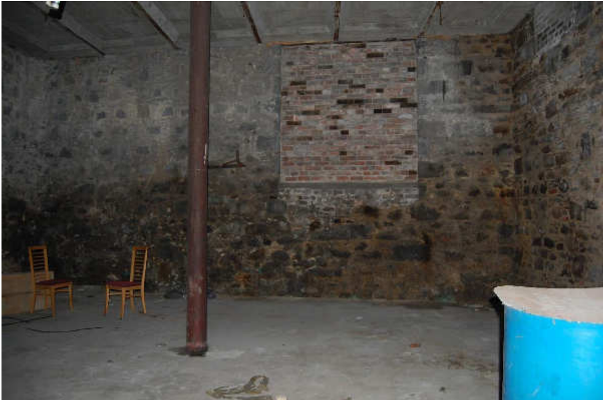
Illus 19 Building 7 lower ground floor showing brick blocked door D5/1, cast iron circular section columns and shuttered poured concrete ceiling; facing WSW.
