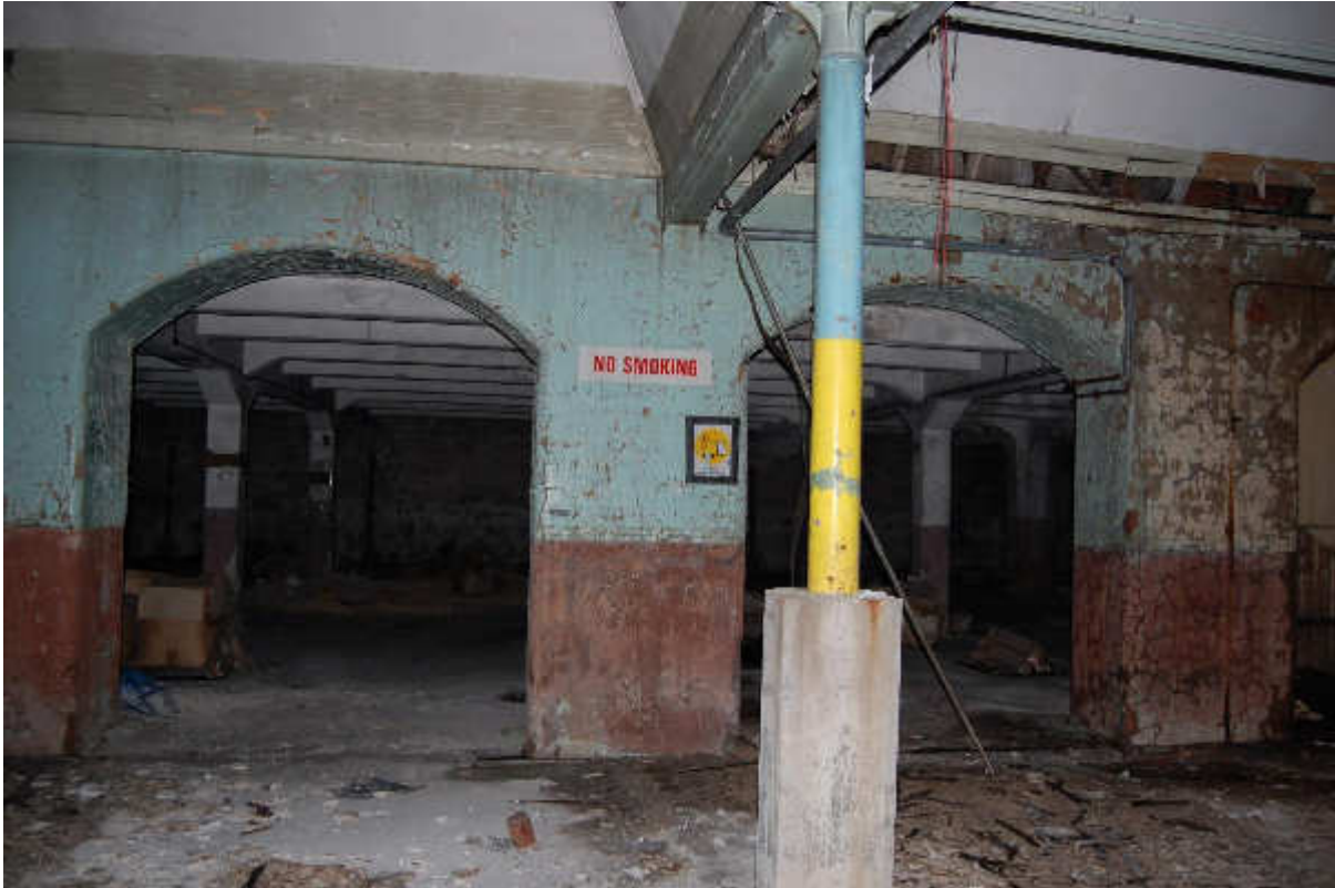
Illus 49 Building 32 ground floor WSW wall leading to basement Building 32A and Building 21; facing W
