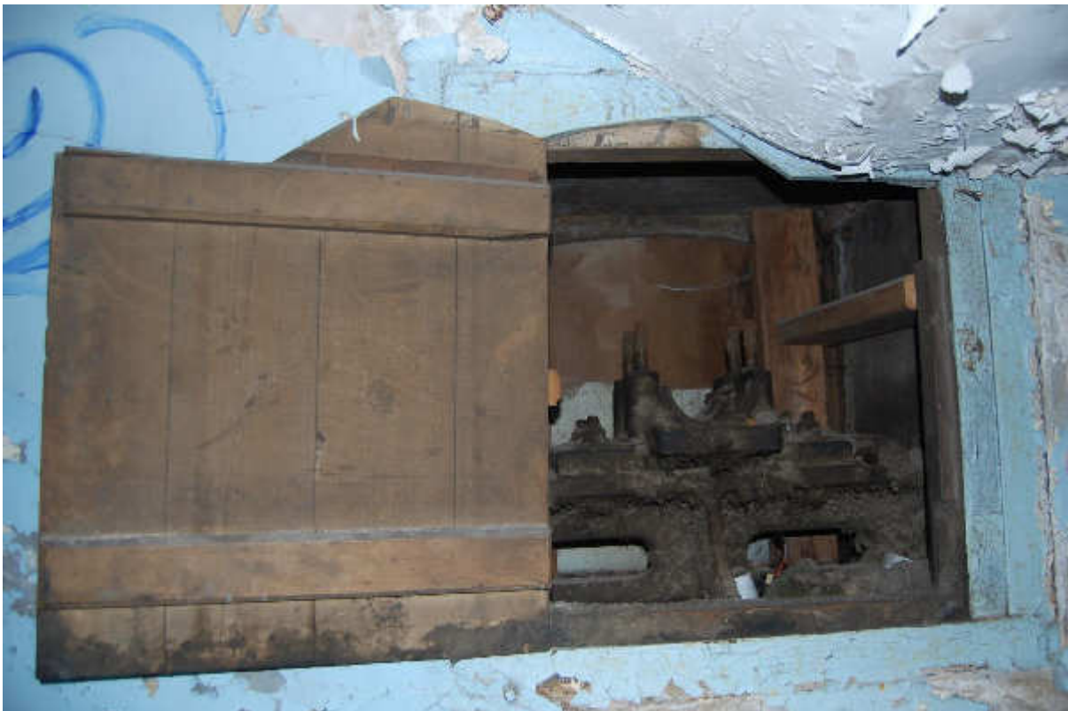
Illus 34 N wall Building 21, cast iron framed inspection hatch with FRASER inscribed on lintel (F51) partially covered by later internal stair to Building 22; facing S
