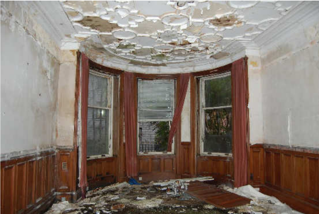
Illus 10 Building 1 Board Room W1/27 interior showing parquet floor and plaster ceiling; facing SSE
