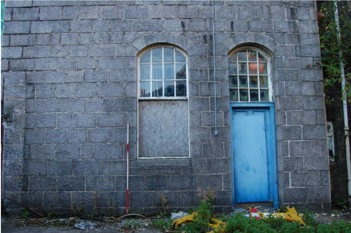
Illus 17 Building 4A window W4A2 (left) and Door D4A/1 (right); facing WSW
