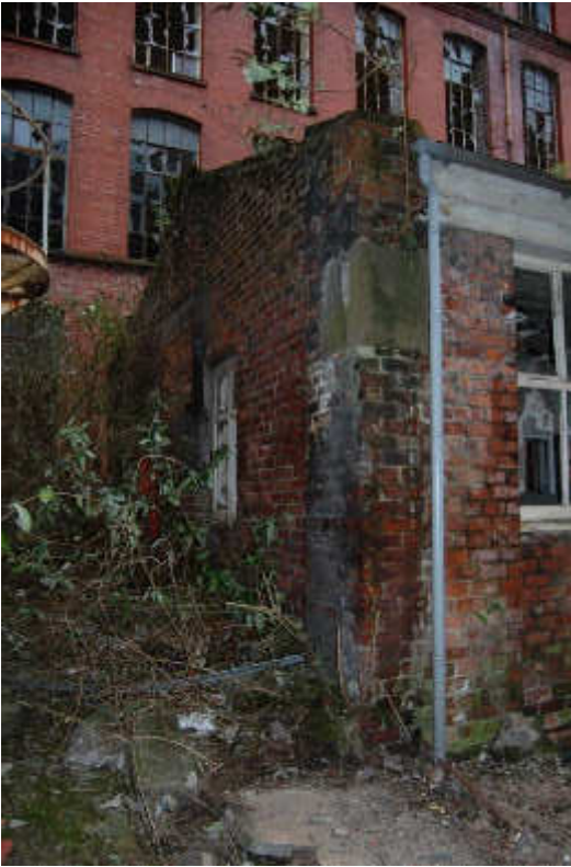
Illus 87 Building 55 N gable showing rebuilding with later grey brick, facing ESE
