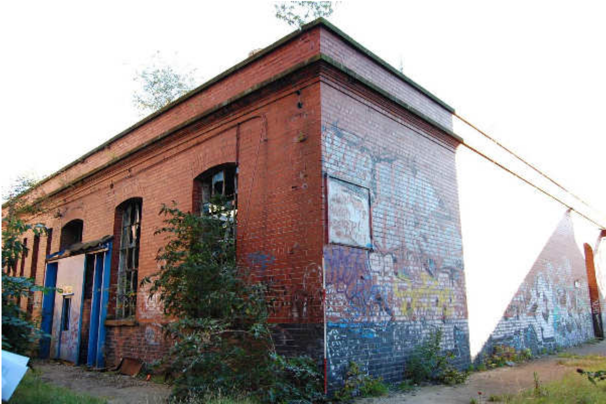
Illus 113 SW corner Building 90 showing two colours of modern brickwork; facing NNE
