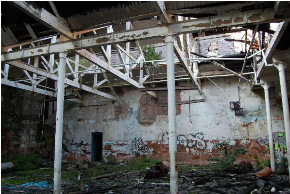
Illus 44 Building 30 interior N wall with door D30/10 showing granite W wall, brick N wall and replacement roof; facing NW
