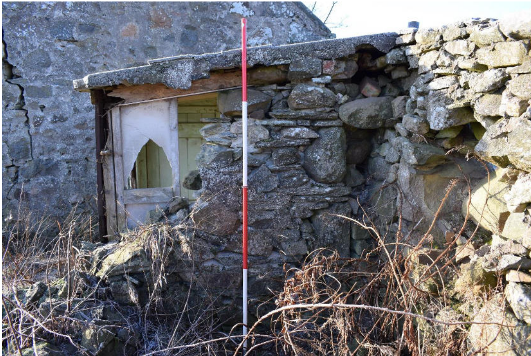
Illus 9 Wall F2 part of the original stone range of buildings, now mainly demolished; facing SE
