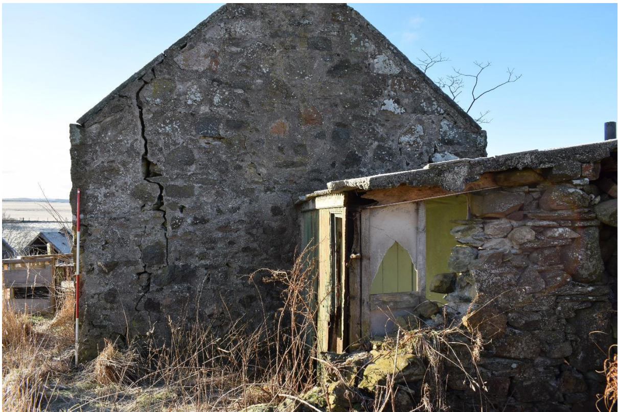
Illus 8 NE gable with tin shed (Rooms 4/5) added later; stone wall F2 (right) remains from demolished building and scar (F7) on the left side of the gable where a wall has been demolished; facing SW
