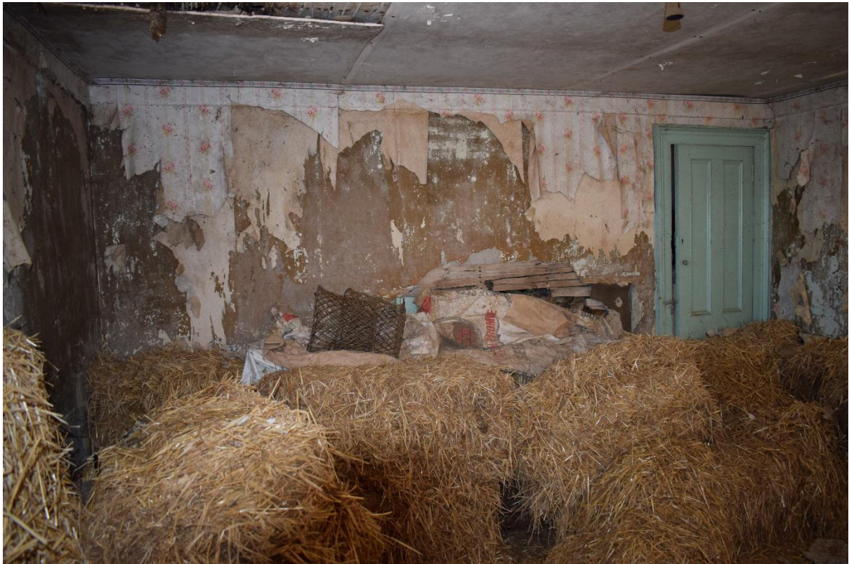
Illus 6 Room 1 interior SW wall showing alcove cupboard F8 (right) which was built in after blocking W3; facing SW.
