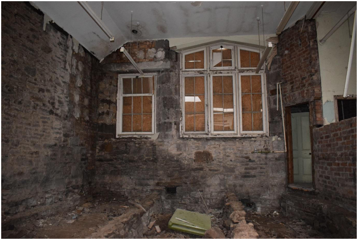
Illus 14 Room 7 E wall windows W30 (left) W29 (right) with sleeper walls and vent; facing E
