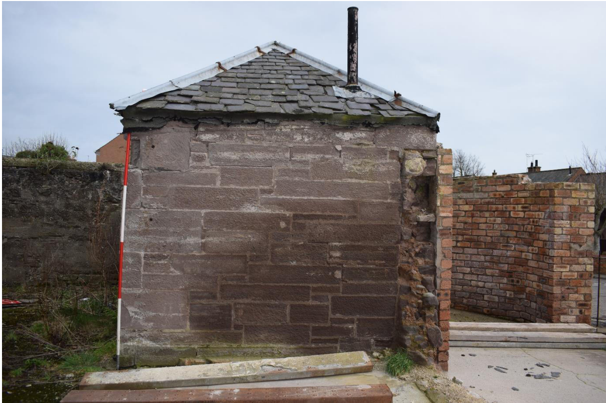
Illus 22 Building 2 W wall showing scar (F11; right) where wall has been removed; facing E
