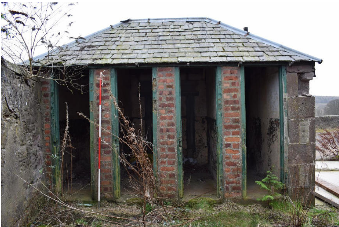
Illus 21 Building 2 N wall stone walls with brick partitions between four cubicle doors; facing S
