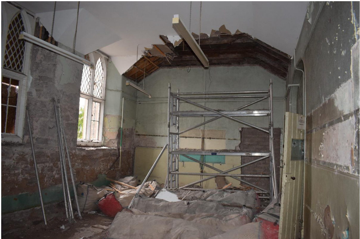
Illus 7 Phase 1 Room 3; the S wall and windows (left) is original and the N wall (right) was rebuilt in Phase 2; facing W
