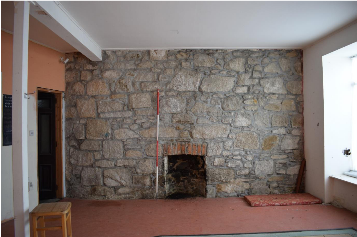
Illus 18 Room 7 ESE wall showing outer face of wall of cottage next door (26 Bogie St) with 24 Bogie St attached later with fireplace F9; facing ESE
