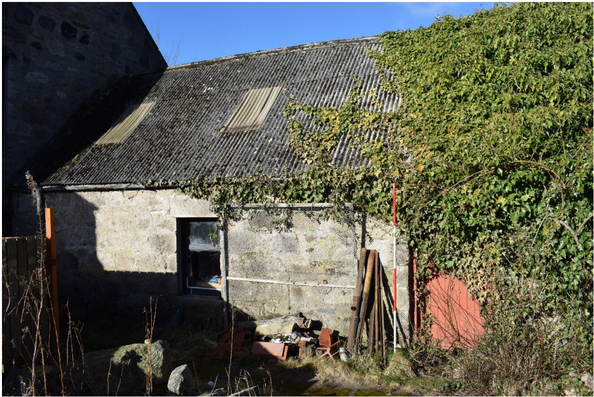
Illus 7 Building 1 E wall showing door D7 and W21 and ivy covering N end of wall; facing WSW
