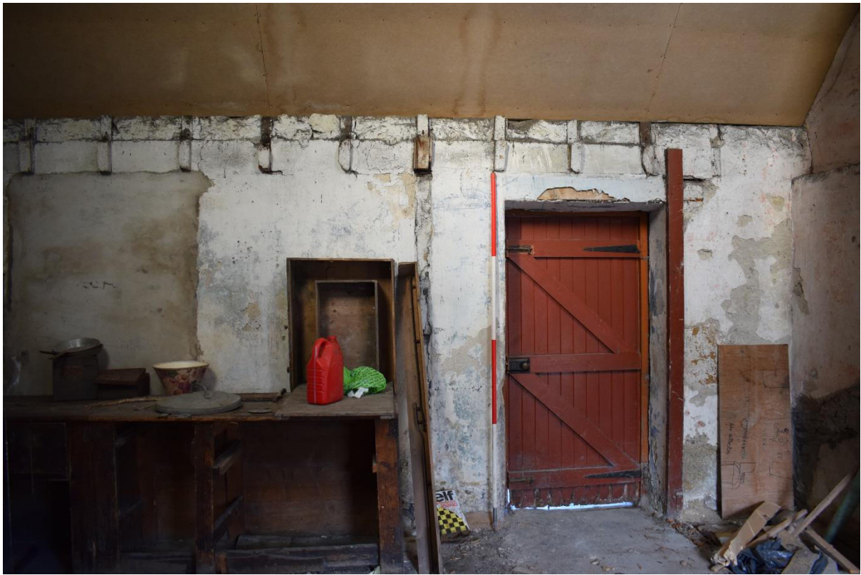
Illus 11 Building 1 Room 2 WNW wall blocked window W2 (left) D2; facing NW
