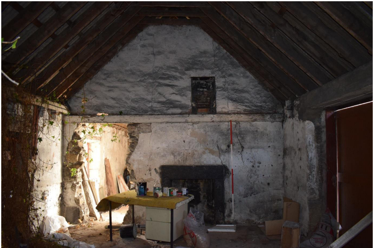
Illus 10 Room 1 SSW wall fireplace F11 (ground floor) and small fireplace F23 (first floor); facing SSW
