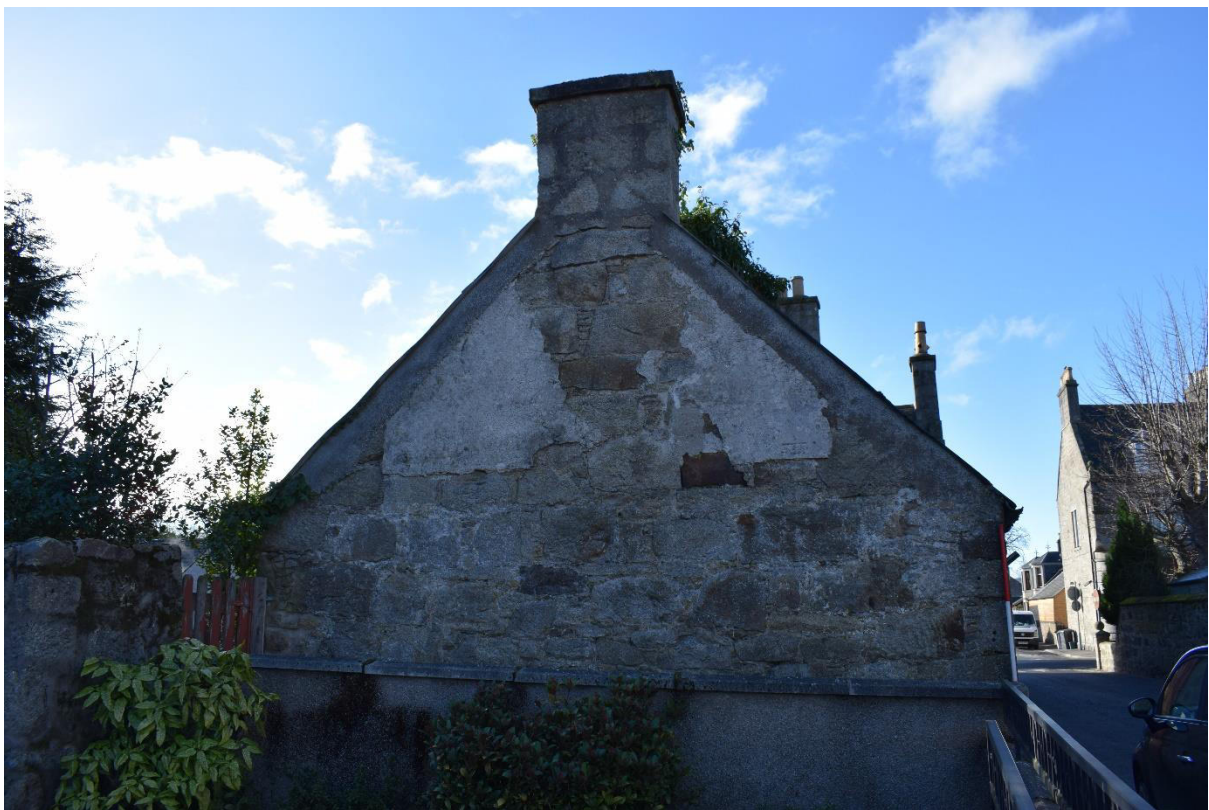
Illus 6 NNE gable Building showing plaster from interior of room (now demolished); facing SSW
