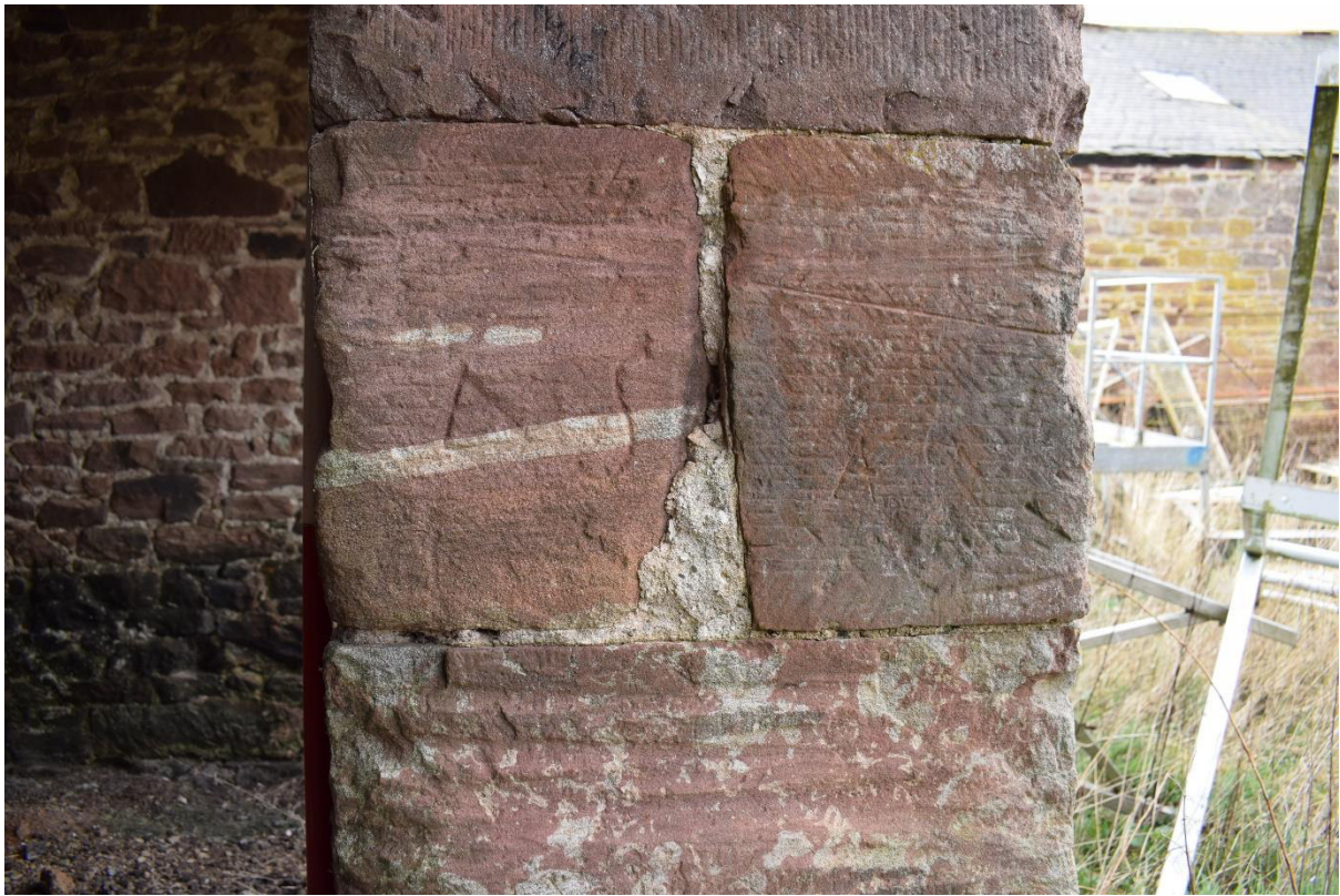
Illus 11 D13 S jamb pillar with graffiti in sandstone blocks
