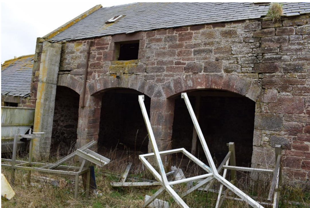
Illus 10 Room 3 cart shed doors D12, D13, D14 (l-r) on E wall of inner courtyard
