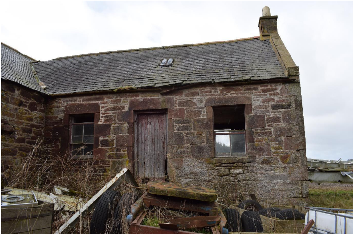
Illus 19 Room 6 the bothy exterior E wall onto inner courtyard W9, D8, W10 (I-R0 facing W)
