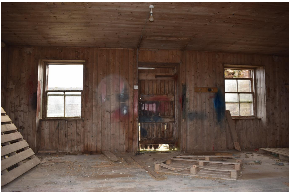
Illus 18 Room 6 the bothy interior with W10, D8, W9 (l-r); facing E
