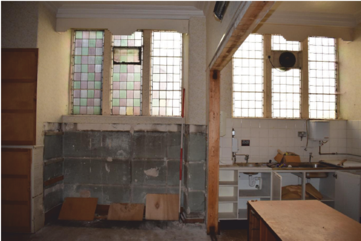
Illus 7 Room 3 (left) and 5 (right) windows W33 (left) W32 (right); facing SE
