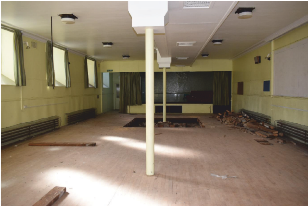
Illus 11 Lower ground floor hall Room 8 with cast iron pillars (F30 and F31 (centre), windows on SW wall W13, W12, W11, W10 (left) and stage (centre); facing NW
