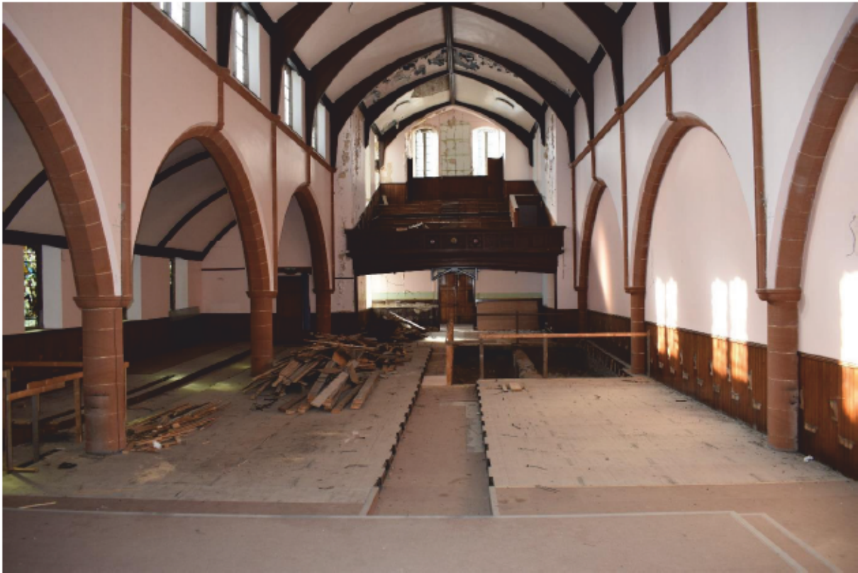
Illus 18 Room 10 interior showing sandstone pillars (F17 and F18 left; F15 and F16, right) with gallery F32 (centre); facing NW
