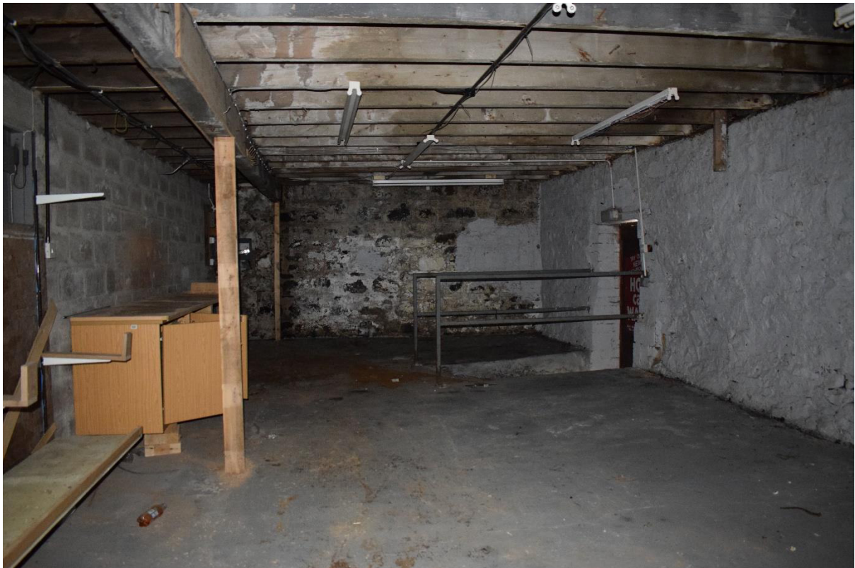
Illus 16 Building 2 interior with stone wall S wall Building 6 (centre); facing N
