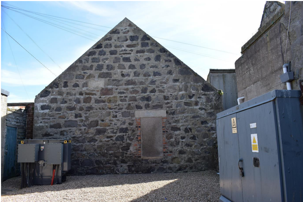
Illus 40 West wall seen through gates of electricity sub-station; no access; facing E
