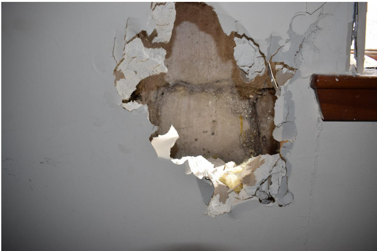
Illus 24 Concrete block construction seen on interior were asbestos contractor had removed plasterboard wall coverings
