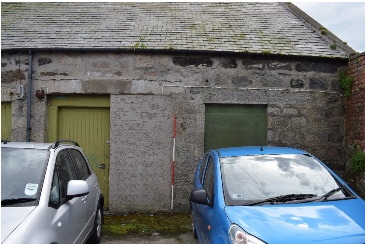
Illus 39 Building 6 N wall D6 (left) showing reduction in with using harled concrete blocks and w34 (right); facing S
