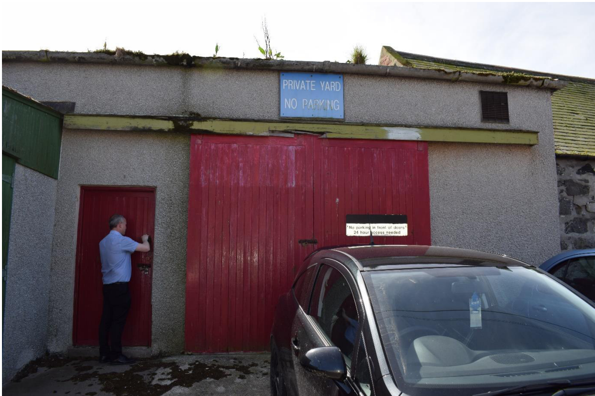
Illus 27 Building 4 N wall showing replacement wall in harled concrete block; facing S
