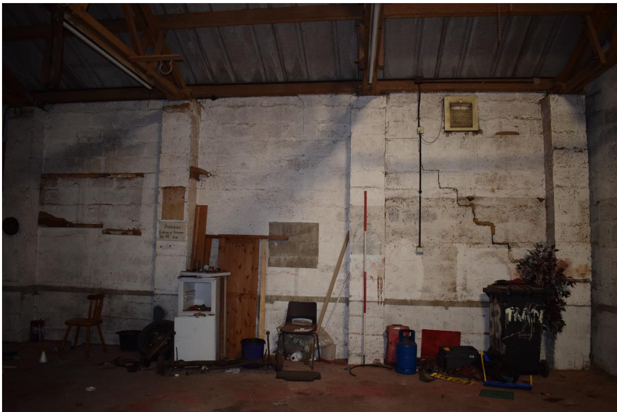
Illus 28 Building 4 N wall interior showing buttresses constructed of concrete blocks; facing N
