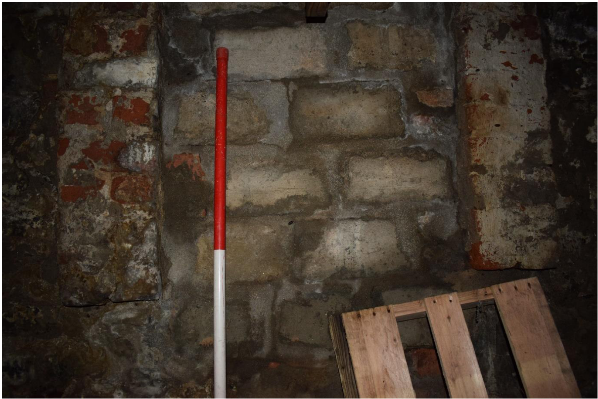
Illus 31 Detail of blocked fireplace F16 which is unpainted, showing brick construction; facing S
