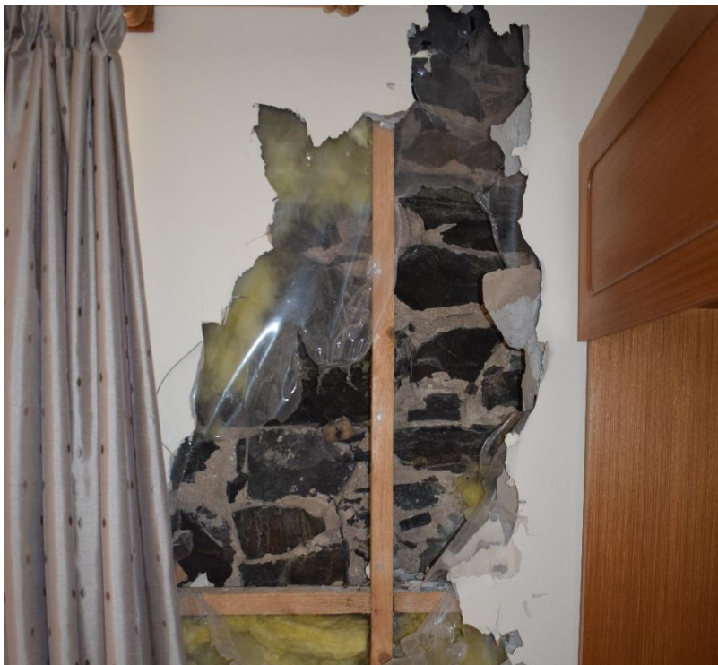
Illus 9 Interior first floor Building 1 showing original stone w wall uncovered by asbestos contractor; facing E
