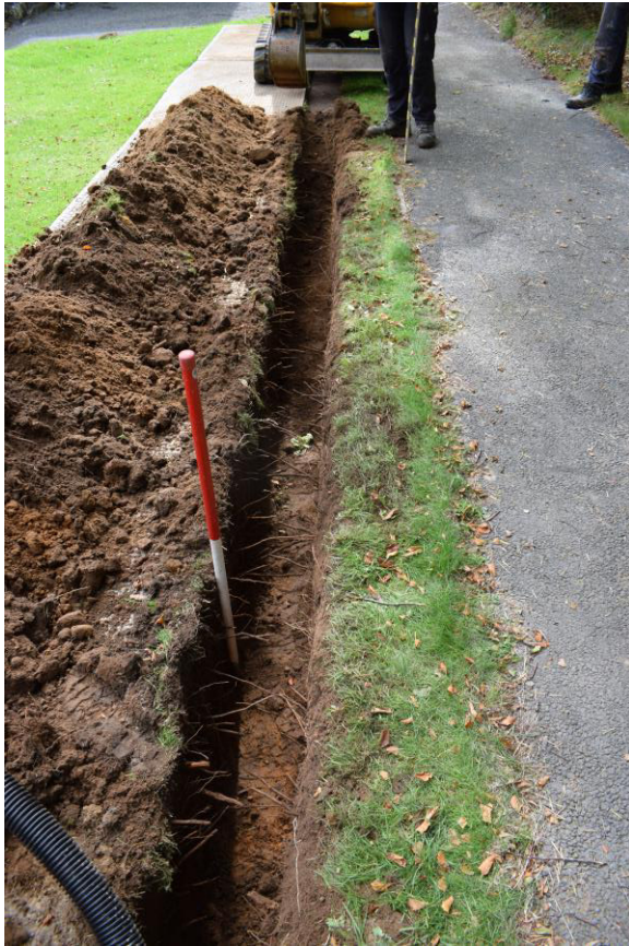
Illus 5 Trench 3 showing sandy natural subsoil; the existing electric supply is under the path (right); facing S
