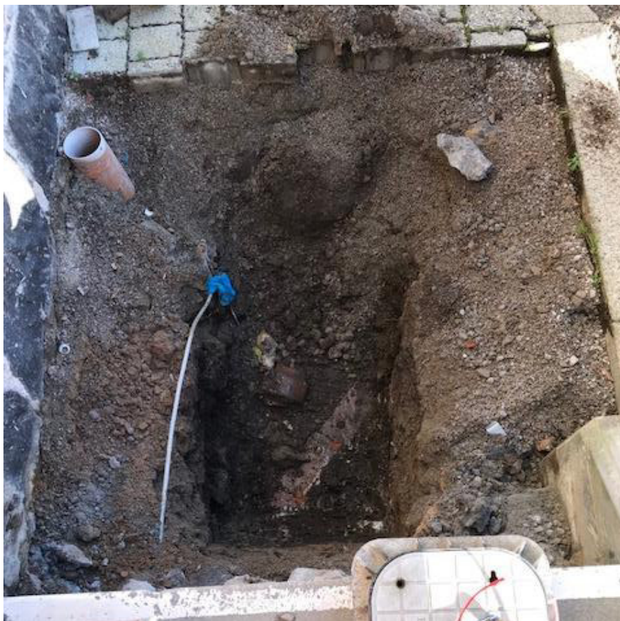
Illus 3 Trench dug through old cable trenches and line of bricks marking 1m deep iron pipe; facing NE
