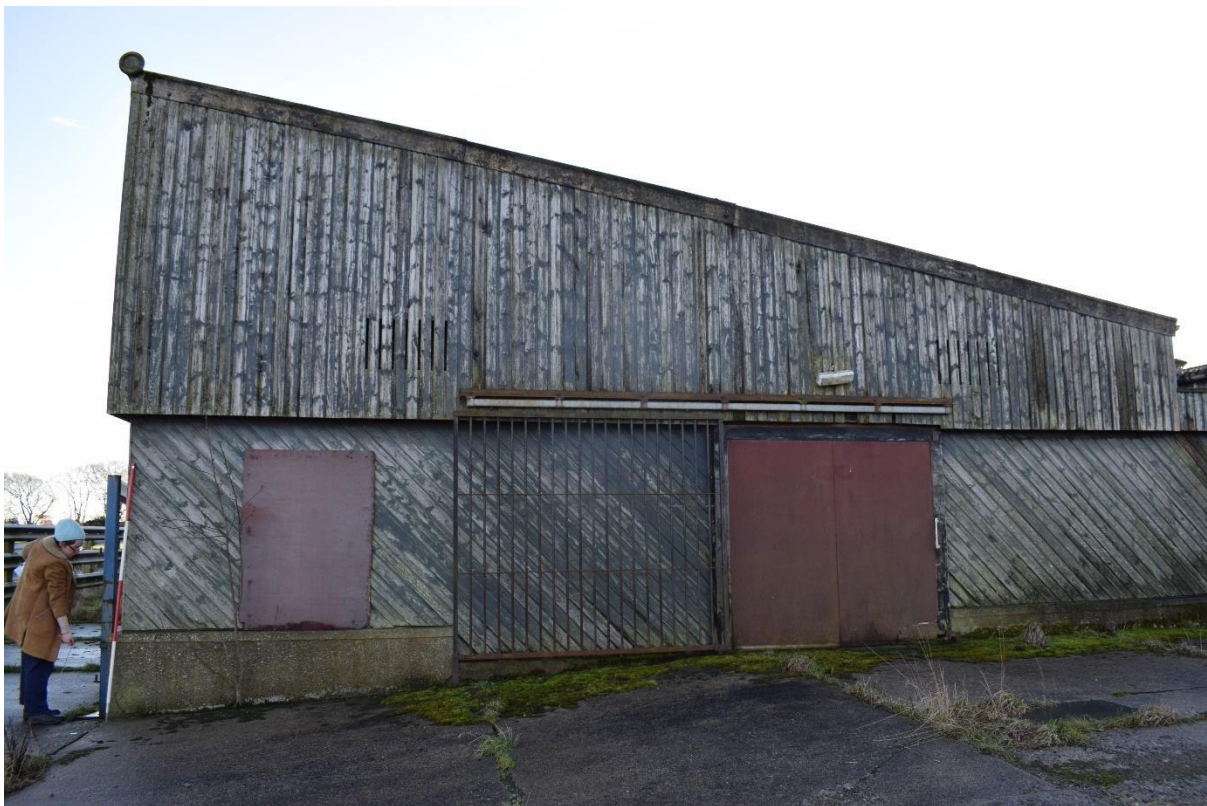
Illus 29 Building 7 NE section NW wall W34 and D21 showing vertical wooden slats above diagonal slats with asbestos roofing; facing SE
