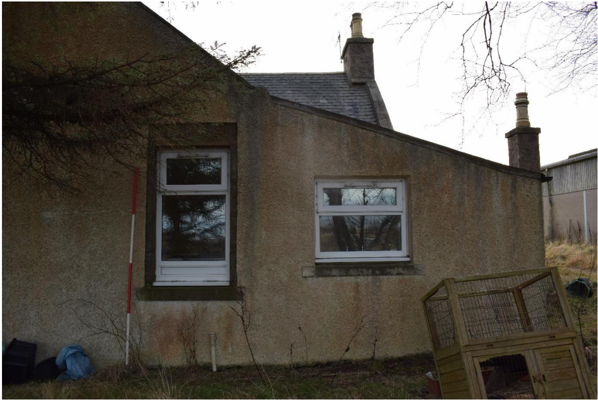
Illus 18 Building 3 N wall W21 (left) with granite lintel and sill in Phase 1 cottage with later addition lean to W22 (right)
