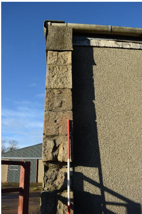
Illus 21 Building 4 SE corner showing granite steading reused as wall of warehouse; facing NW
