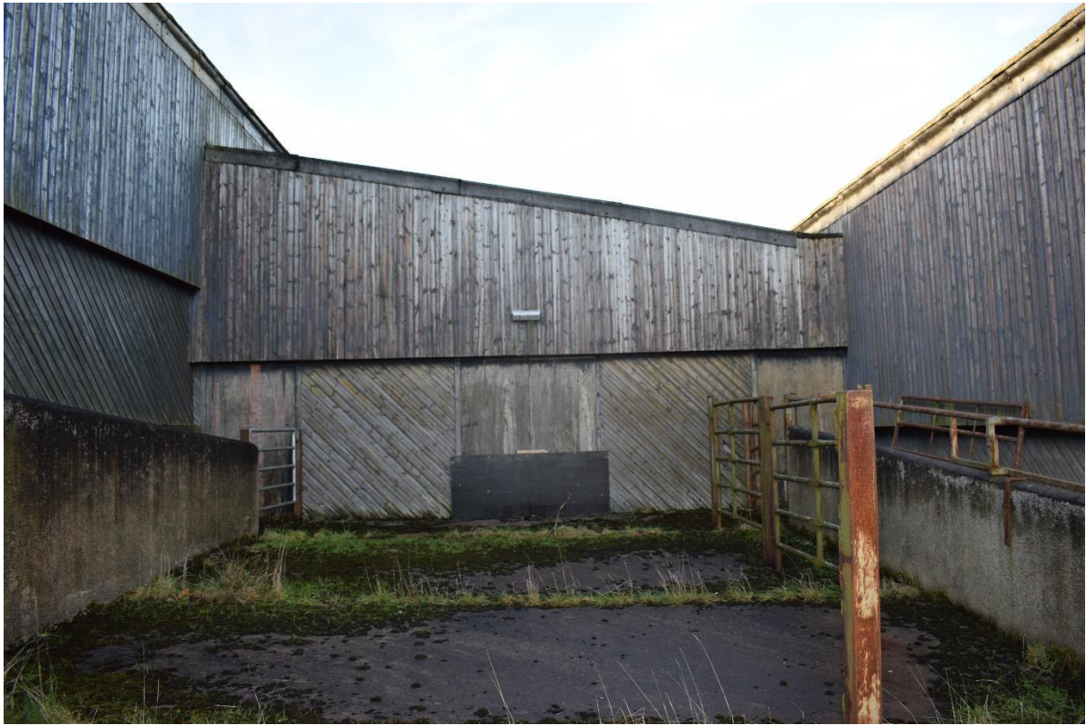
Illus 32 Building 7 SE wall cattle court with concrete ramp F38 (left) D29, D30, D31 and concrete ramp F39 (right); facing NW
