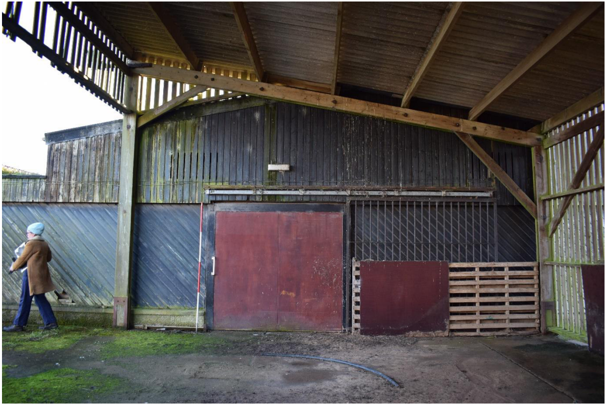
Illus 30 Building 7 SW end wall with D24 and Building 7A posts and roof (top); facing SE
