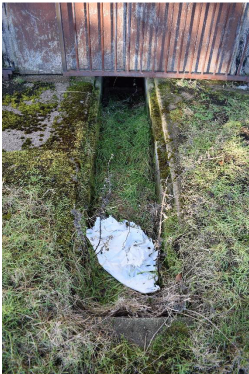
Illus 33 Building 7 SE wall concrete channel running from under door D30; facing NW
