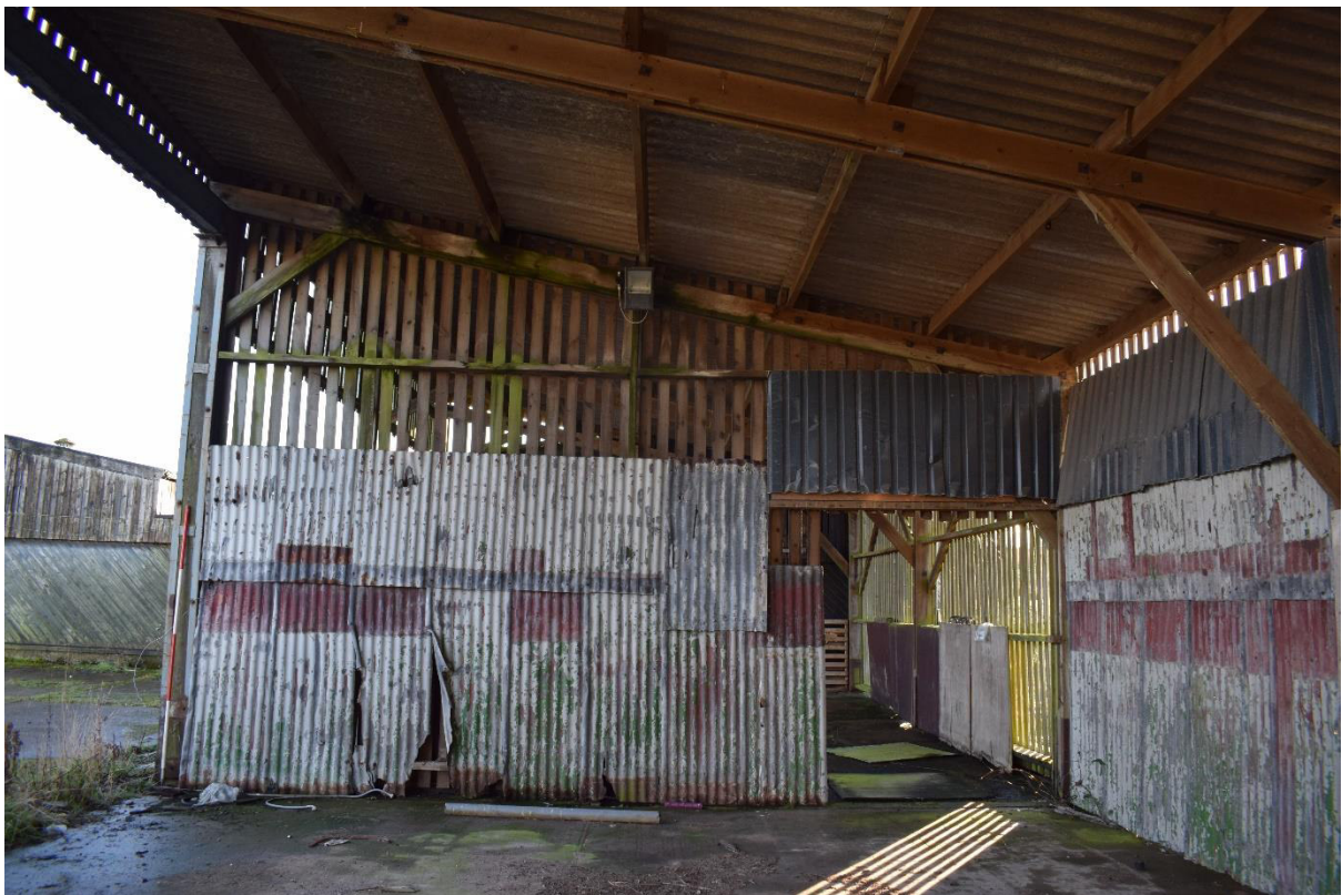
Illus 37 Building 7A partition wall showing wooden slat and metal sheet construction; facing NW
