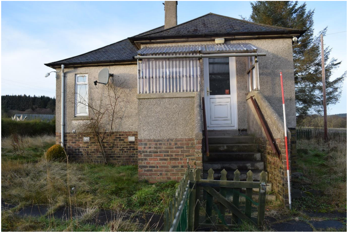
Illus 6 Building 1 E wall showing steps F2, D2 and W4, W5 (left); facing W
