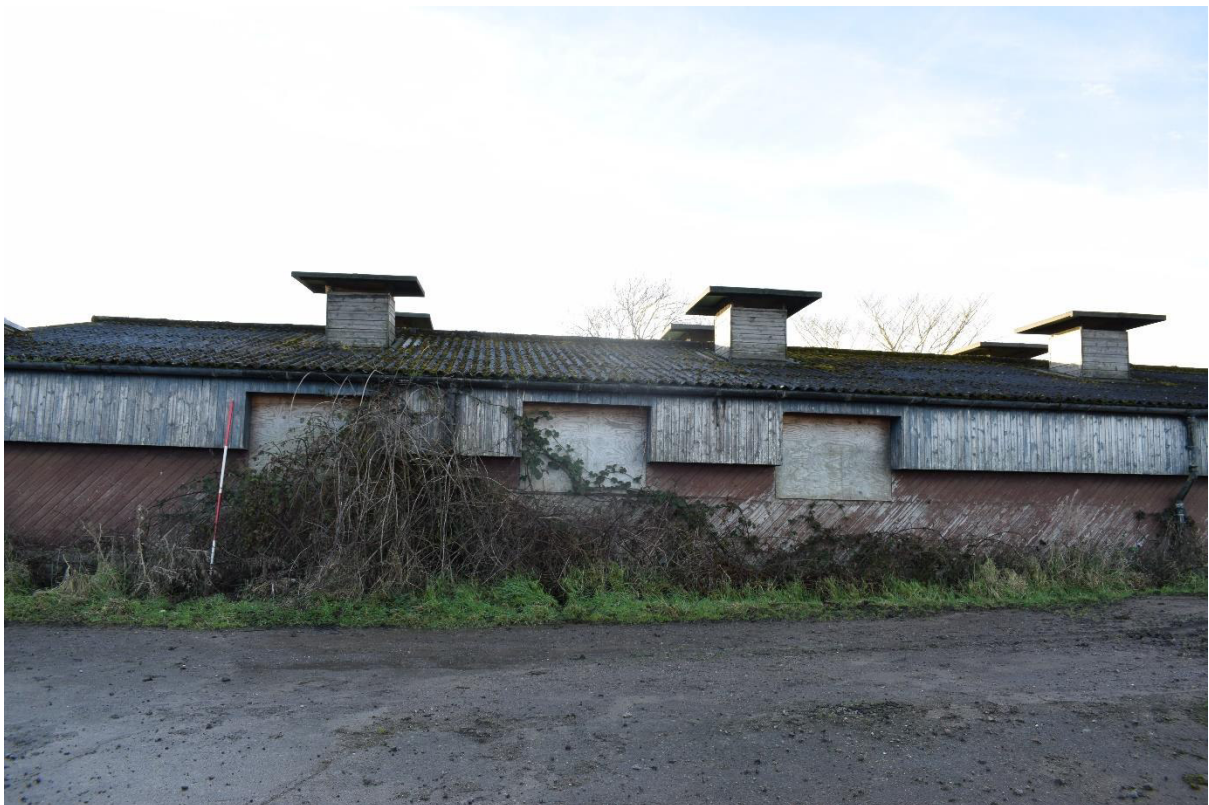
Illus 45 Building 10 NE wall with boarded up windows W31, W32, W33 and wooden vents above F30, F31, F32; facing SW
