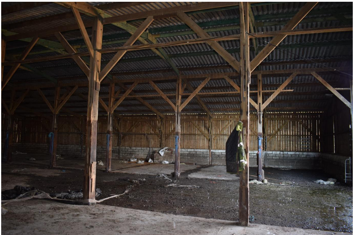
Illus 42 Building 9 interior showing wood slat construction, wood posts and asbestos roof; facing SW
