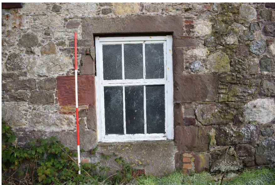
Illus 2 E wing Room 16 W wall D31 converted into window W49; facing E
