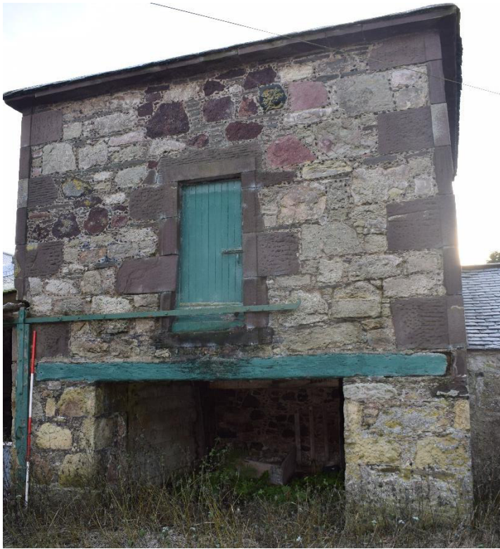
Illus 16 Doocot Room 34 N façade D36 (ground floor) with D21 above; facing S
