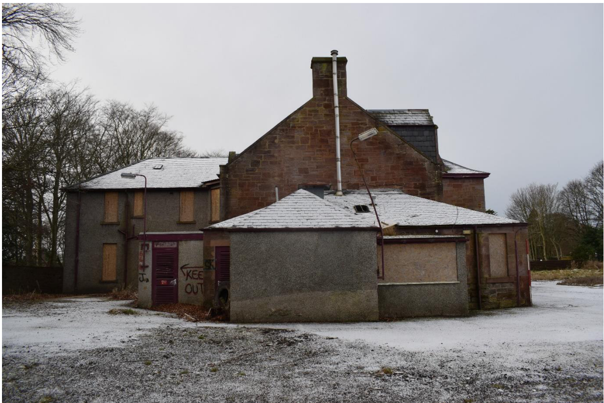
Illus 15 Phase 1 gable (centre), Phase 2 sandstone extension (right), Phase 3 SE extension (left), Phase 4 lean-to extensions (foreground); facing SW
