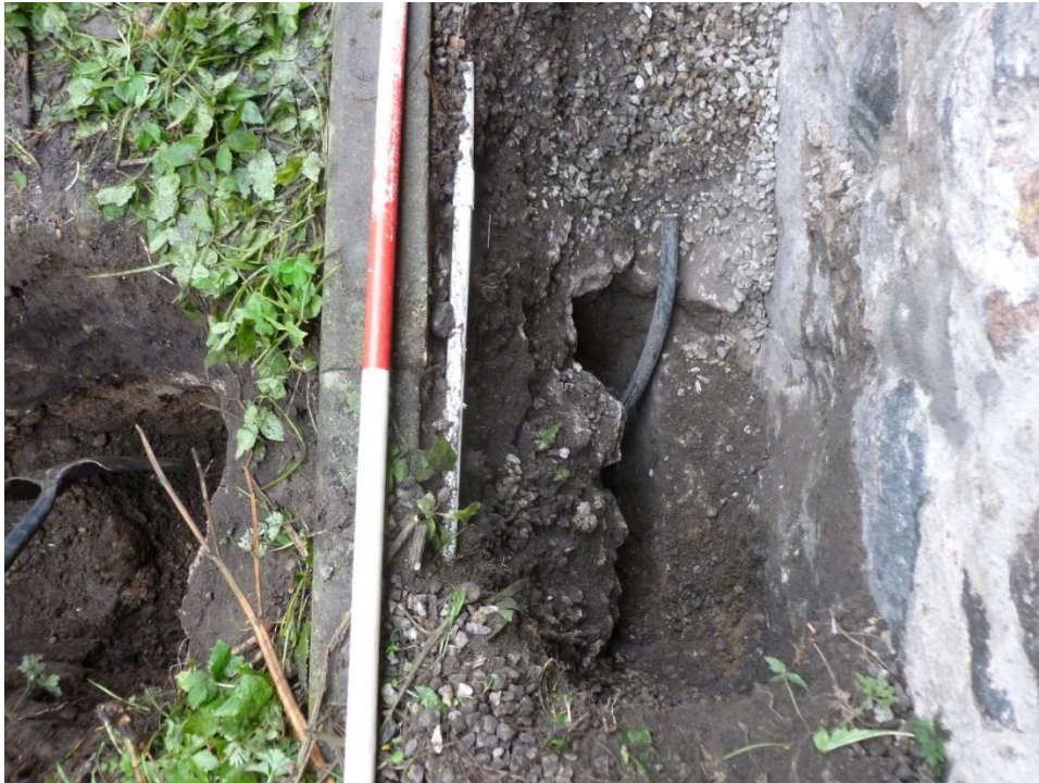
Illus 4 Trench 21 NE wall of Provost Skene's House (right), foundation F3 (centre right) with telephone cable and concrete foundation and kerbing under ranging rod; facing NE
