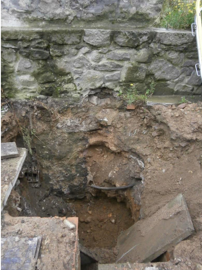
Illus 5 TP20 showing wall F5 with natural subsoil below and wall scar F5 (centre) which has been removed by machine; facing SW
