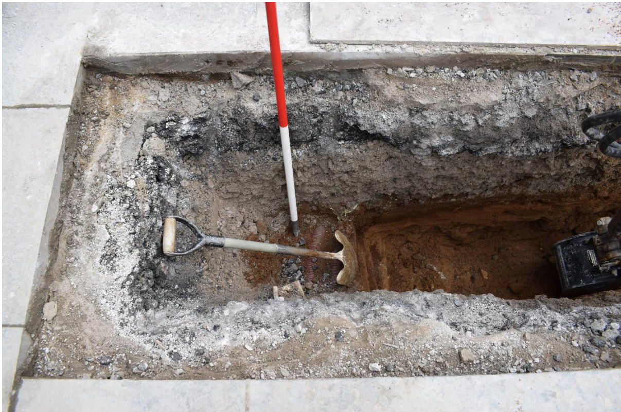
Illus 9 NE end of trench showing natural pebble and sand natural at 0.75m deep and cabling (left)
