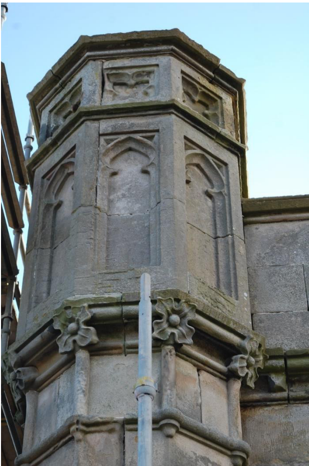
Illus 44 Tower detail of top of octagonal chimney flue F34; facing E
