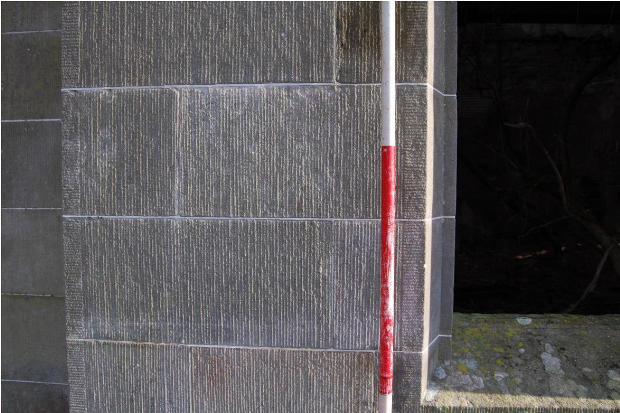
Illus 19 Detail of tooling on sandstone ashlar, window W1, west gable; facing E
