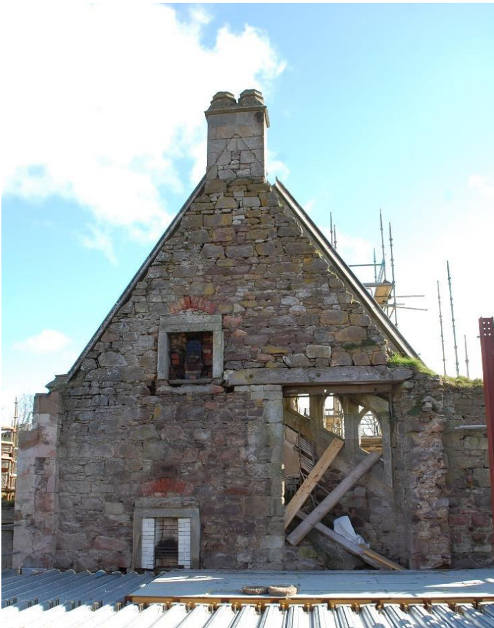
Illus 56 Gable Room 63 with D36 right leading to W43, fireplace F63 below fireplace F64 above; facing E
