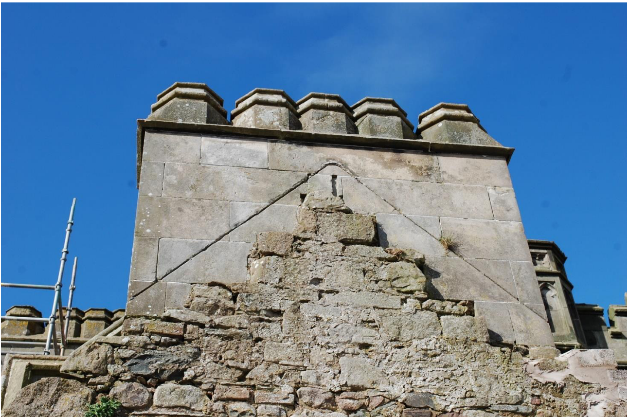
Illus 48 Gable and chimney W wall above Room 57 W gable with sandstone chimney pots in situ (F72) of ashlar sandstone with Phase 1 roof raggle; facing W
