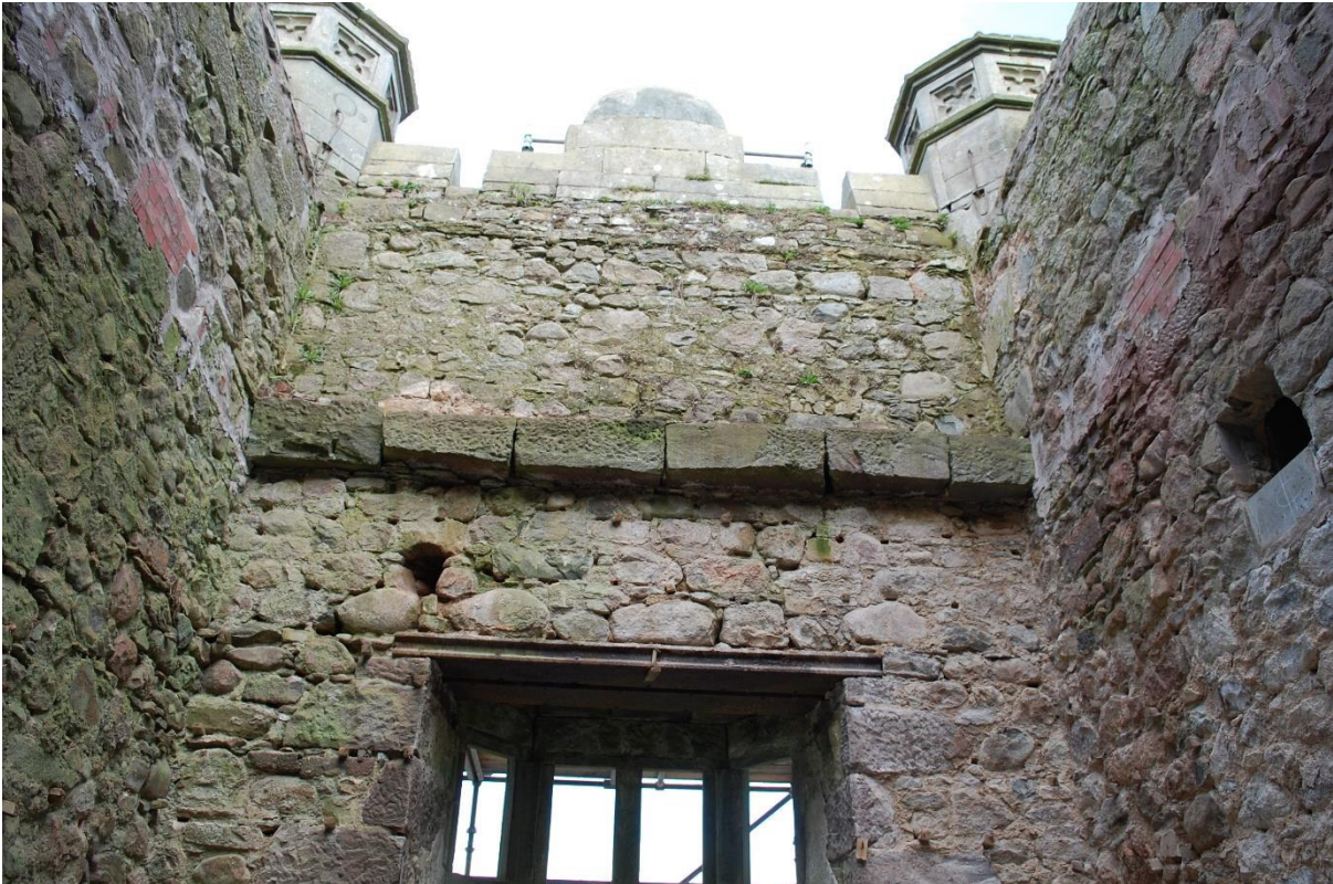
Illus 45 Above Room 52 wall above W33B showing stone corbels where floor has been removed from upper level of tower; facing N
