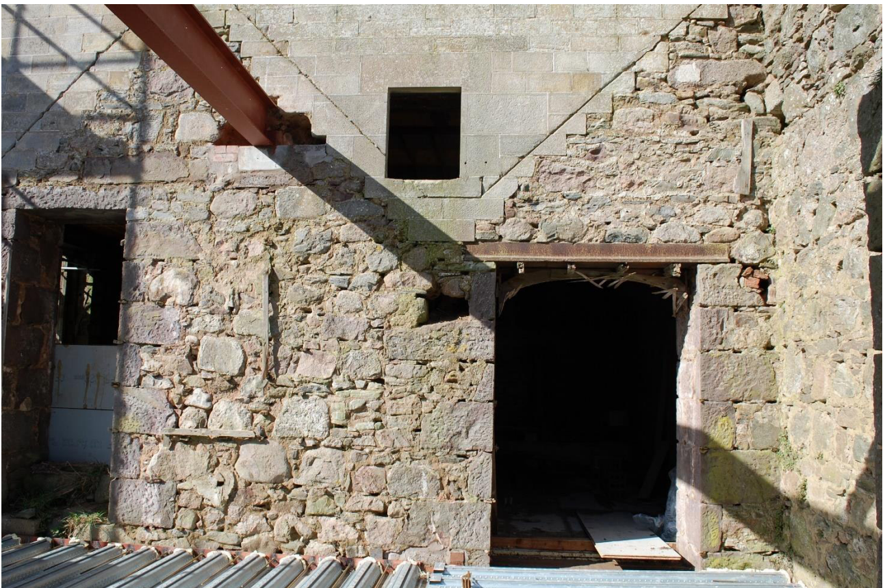
Illus 46 Room 57 W wall D24, W51, D70 (right) with wall above including Phase 1 roof raggle (F67 cut into ashlar sandstone; facing W
