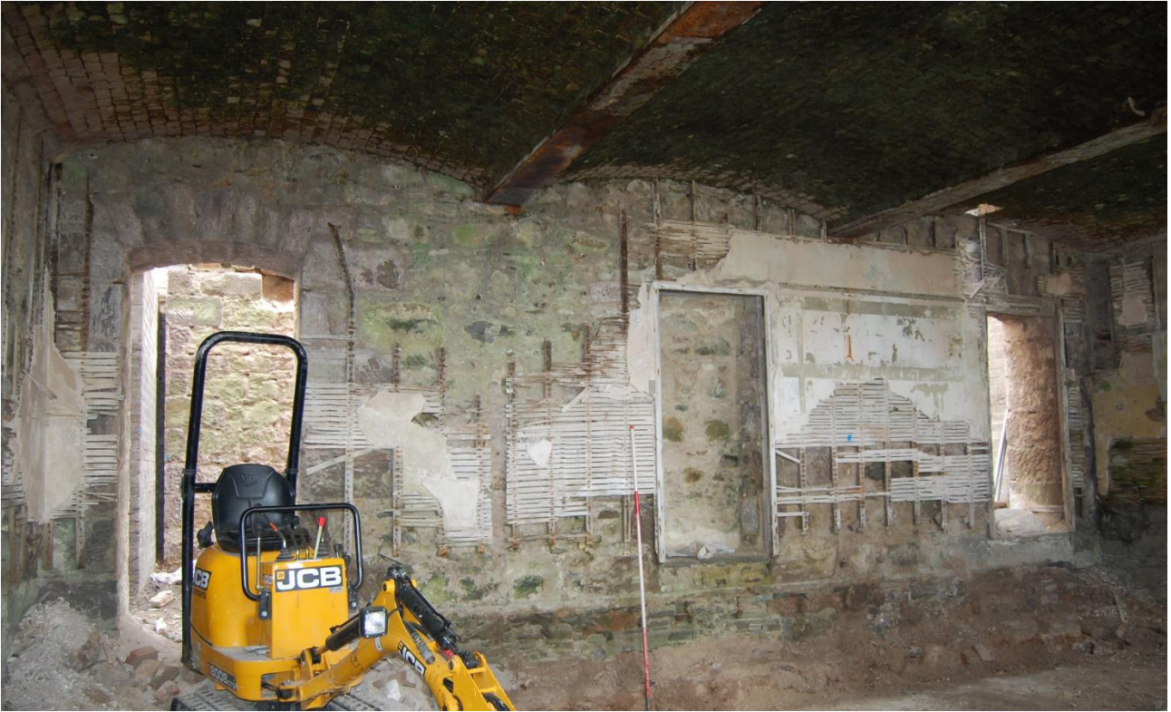
Illus 17 Room 3 N wall with brick vaulting above and D13 (left) blocked door D22, D23 (right)
