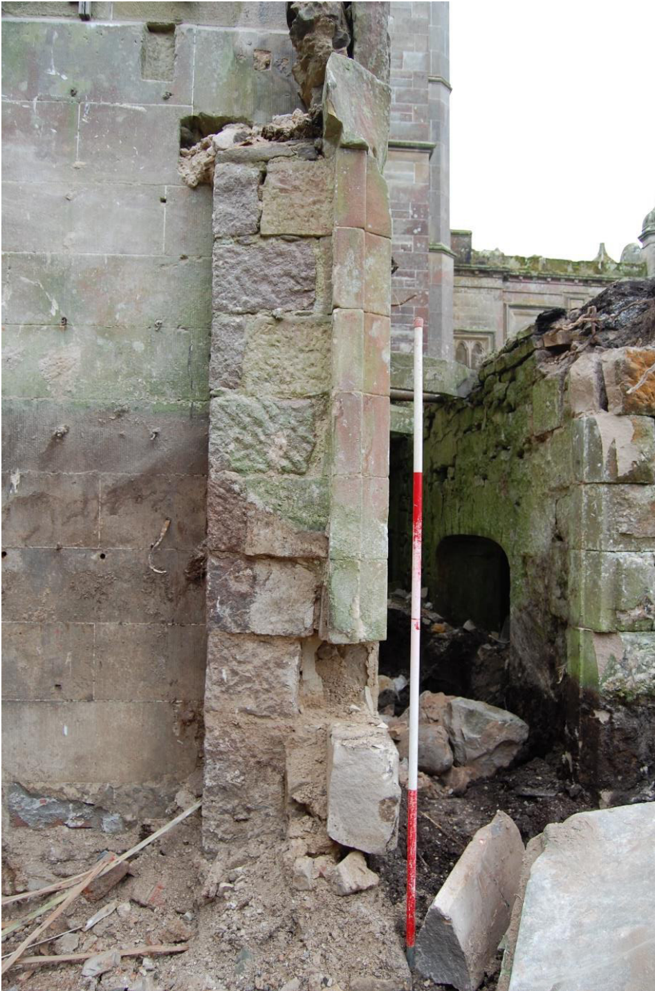
Illus 25 Ashlar sandstone facing on Phase 1 building, NE external corner Room 17 with ashlar finish (left); facing W
