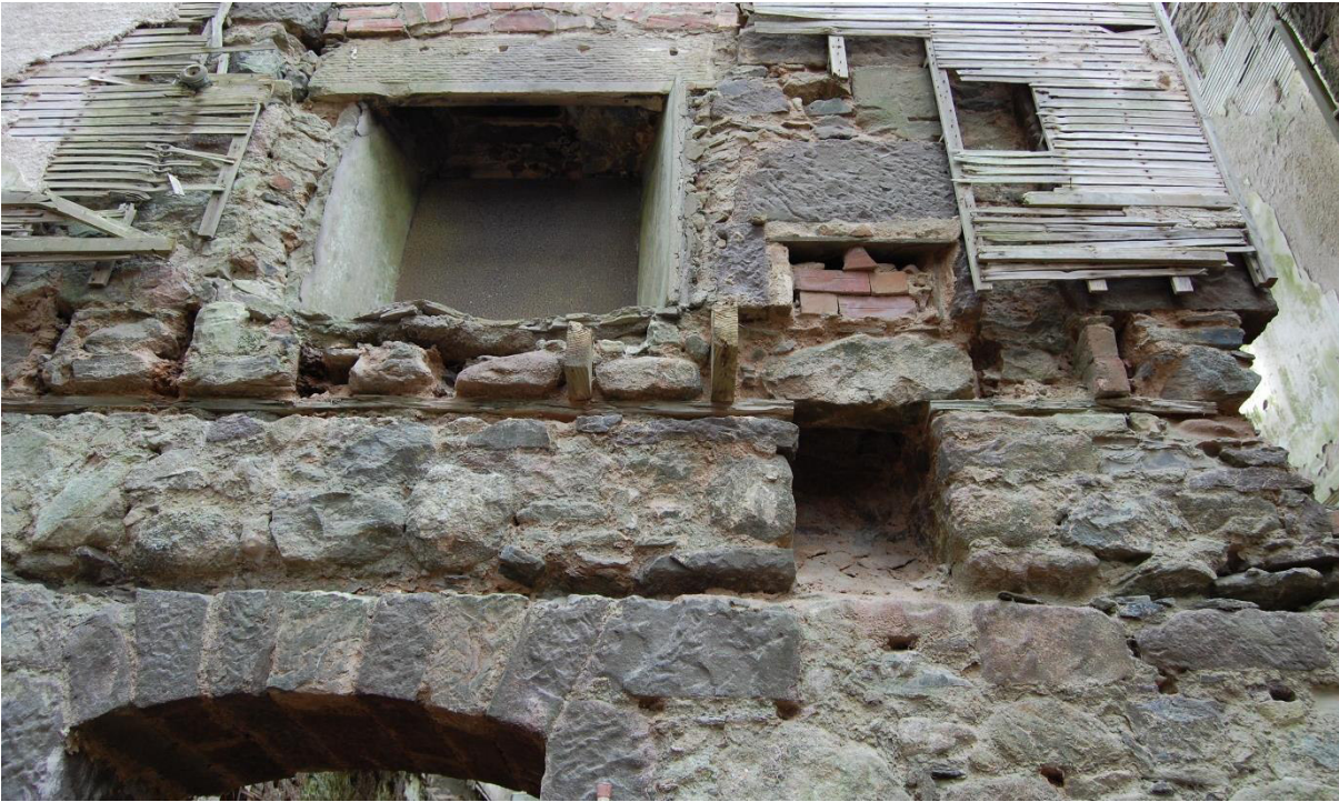
Illus 21 South wall corridor Room 7 with Door D11 (bottom left) Flue 3 (centre) and fireplace F5 (left top); facing S
