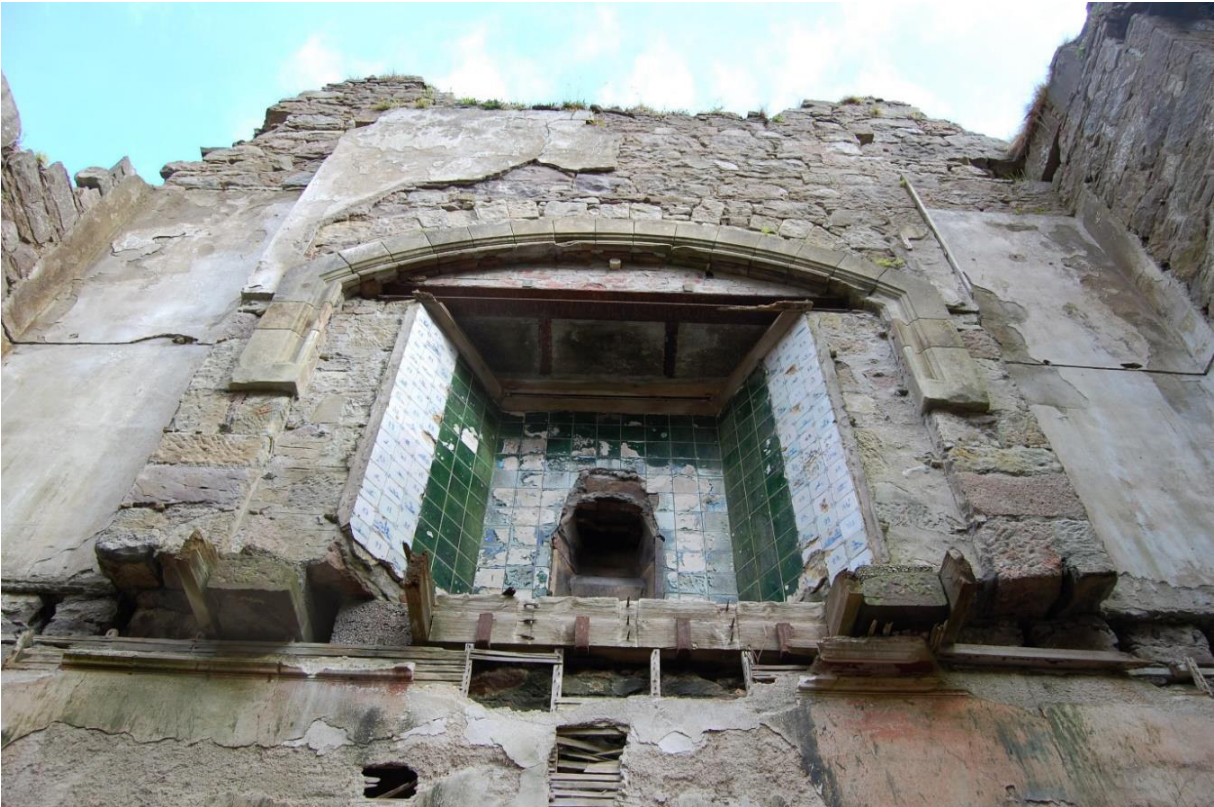
Illus 53 Room 33 fireplace built into decorative window F33 N wall ground floor; facing N
