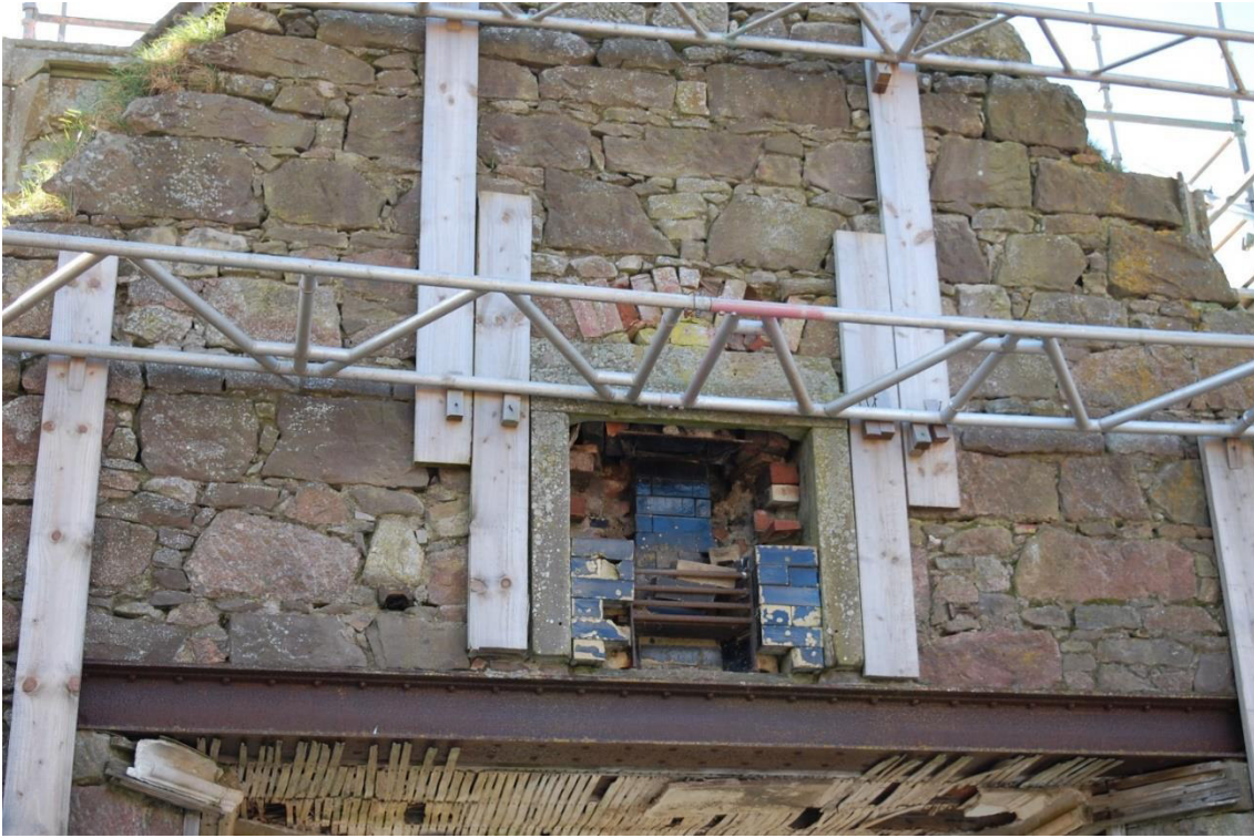
Illus 55 Room 60 F61, sandstone surround, brick relieving arch over and brick insert including blue painted bricks; facing S
