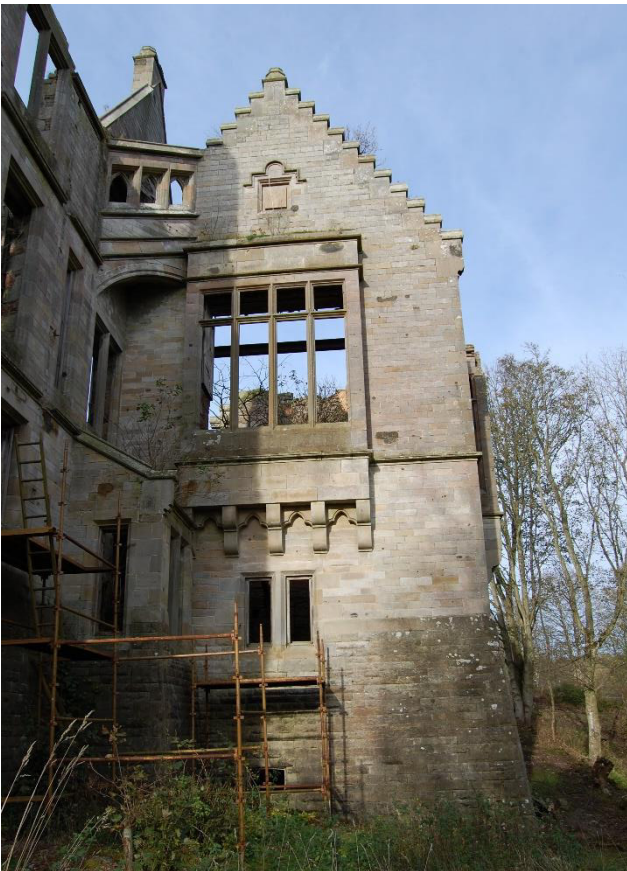
Illus 52 Crowstep gable on south wall east wing Room 19 with window W43 (top left), W17/A (centre) and plaque P4 (top); facing N
