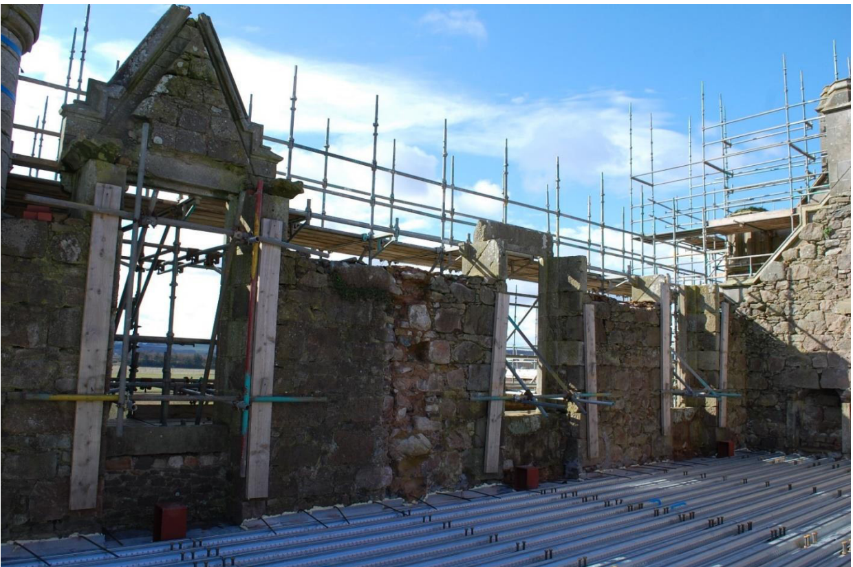
Illus 54 Rooms 45 and 62 S wall W14B left W13 B centre W12B right; facing SW
