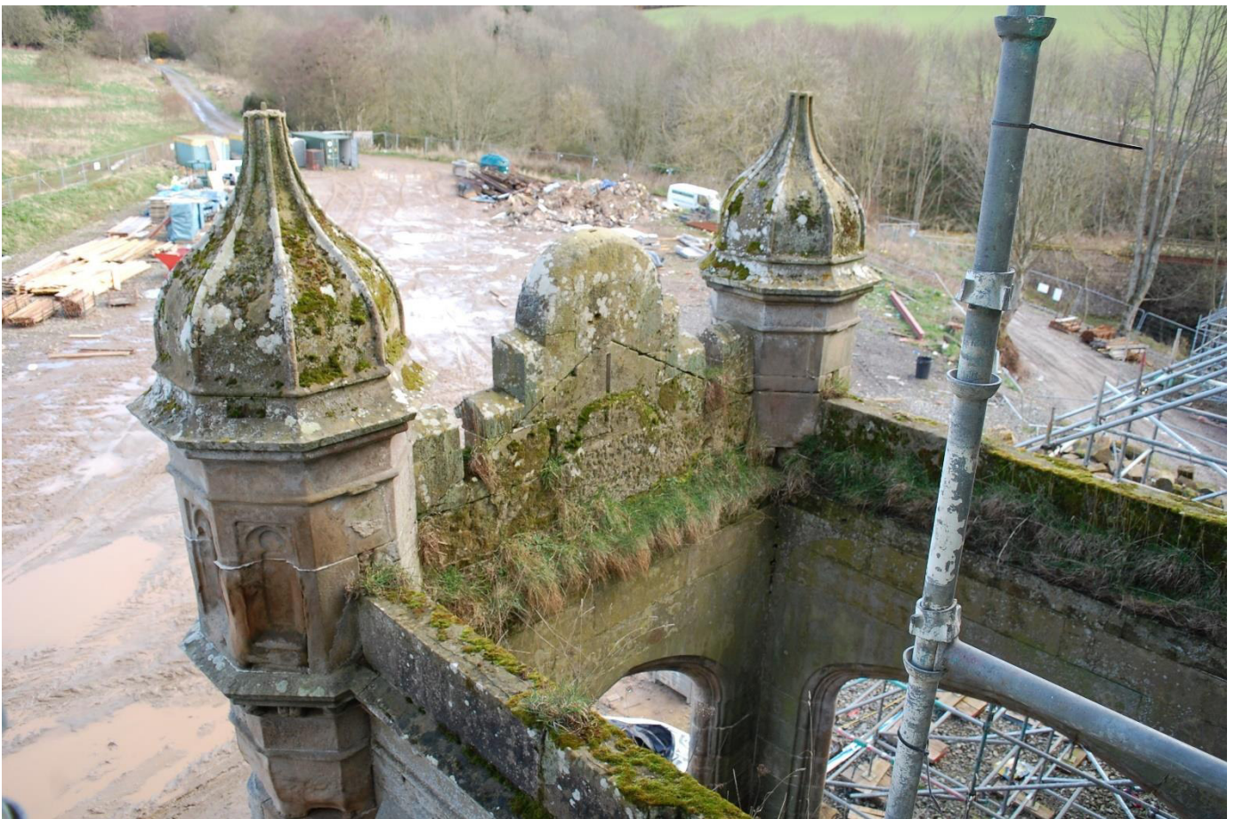
Illus 32 Wall heads Room 20 porte cochere F31 left F32 right; facing NE
