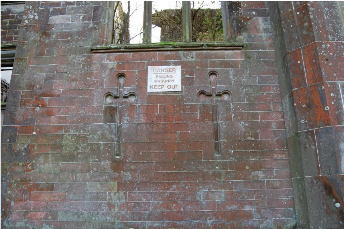
Illus 33 Exterior N wall Room 23 incised crosses (F28) with W31A (above); facing S
