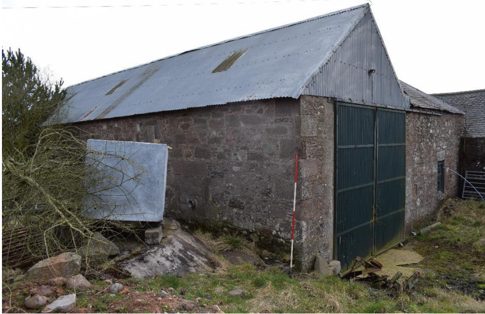
Illus 14 Farm from the W showing D1 (right) and former location of horse mill (left) with concrete tank under metal tank (left); facing E
