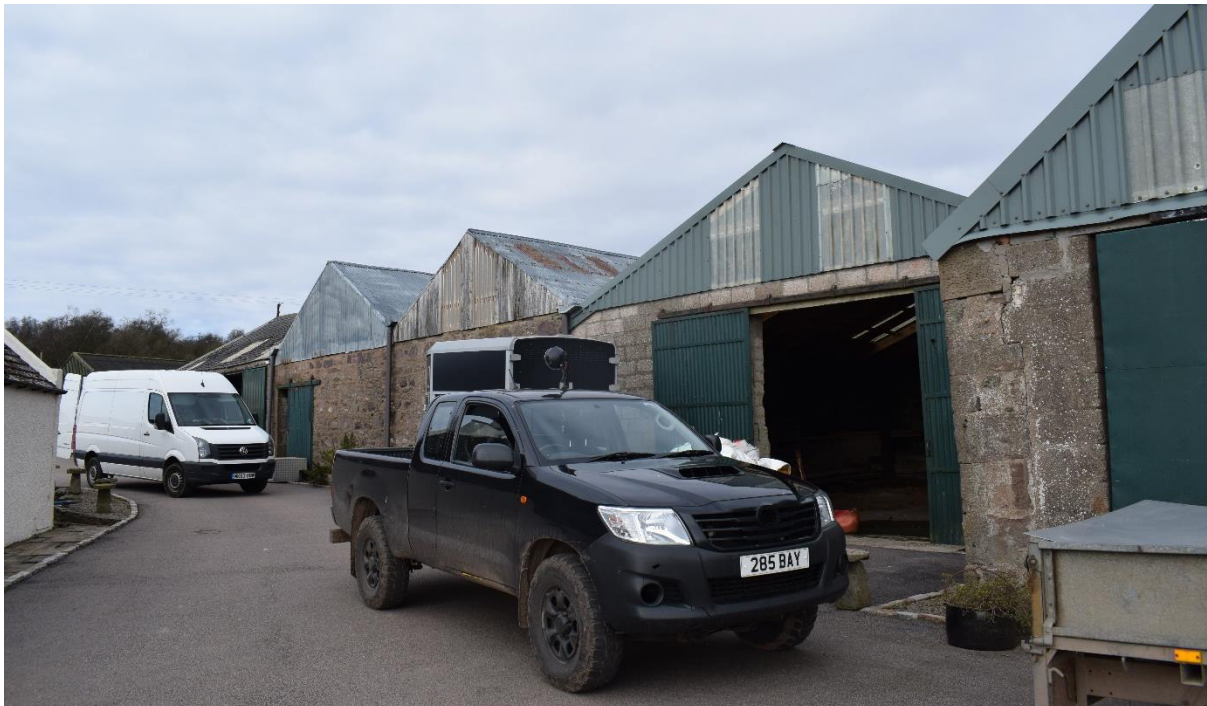
Illus 13 SE façade with Phase 2 Room 5 SE gable (right), Phase 3 breeze block infill (centre), Phase 2 granite wall (left of centre) and Phase 1 SW wing (left); facing W
