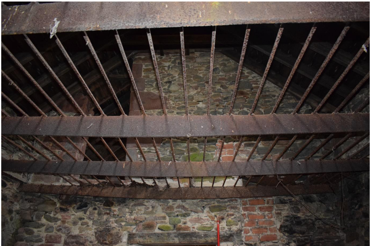
Illus 18 Room 2 iron frame and mesh F26 for drying grain with D3 (left) and blocked aperture F11 (right) grain chute leading to wooden chute in Room 1; facing SE
