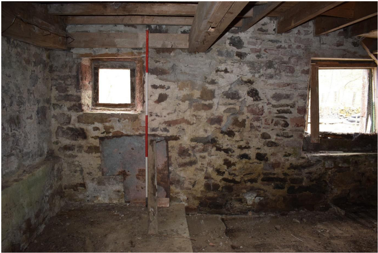
Illus 12 SW wall SE end W6 (left) F6 (behind metal sheet), concrete plinth F17 (bottom) and W5 (right) with wooden platform F28 (above); facing SW
