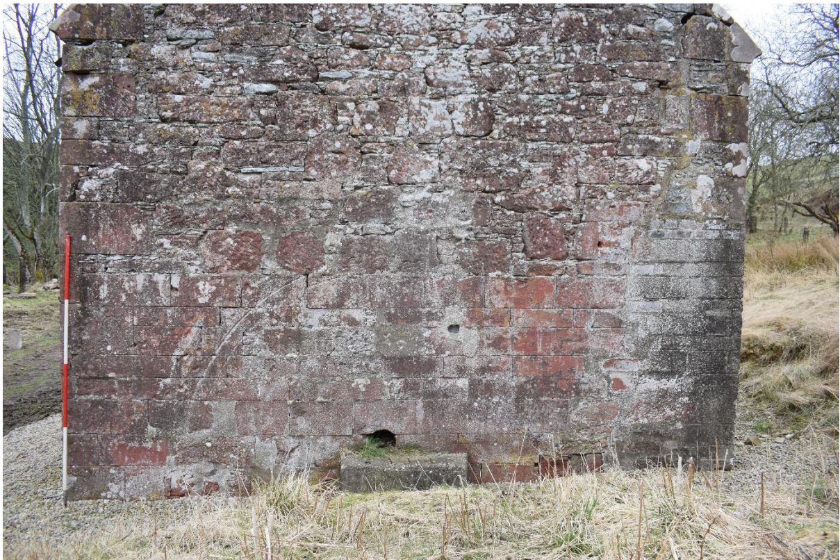
Illus 21 SE gable lower section showing concrete outer headstock (F9) and circular axletree aperture (F8; centre) and three incised circular scars (F7; left) on red sandstone ashlar where mill wheel has scored the ashlar; facing NW
