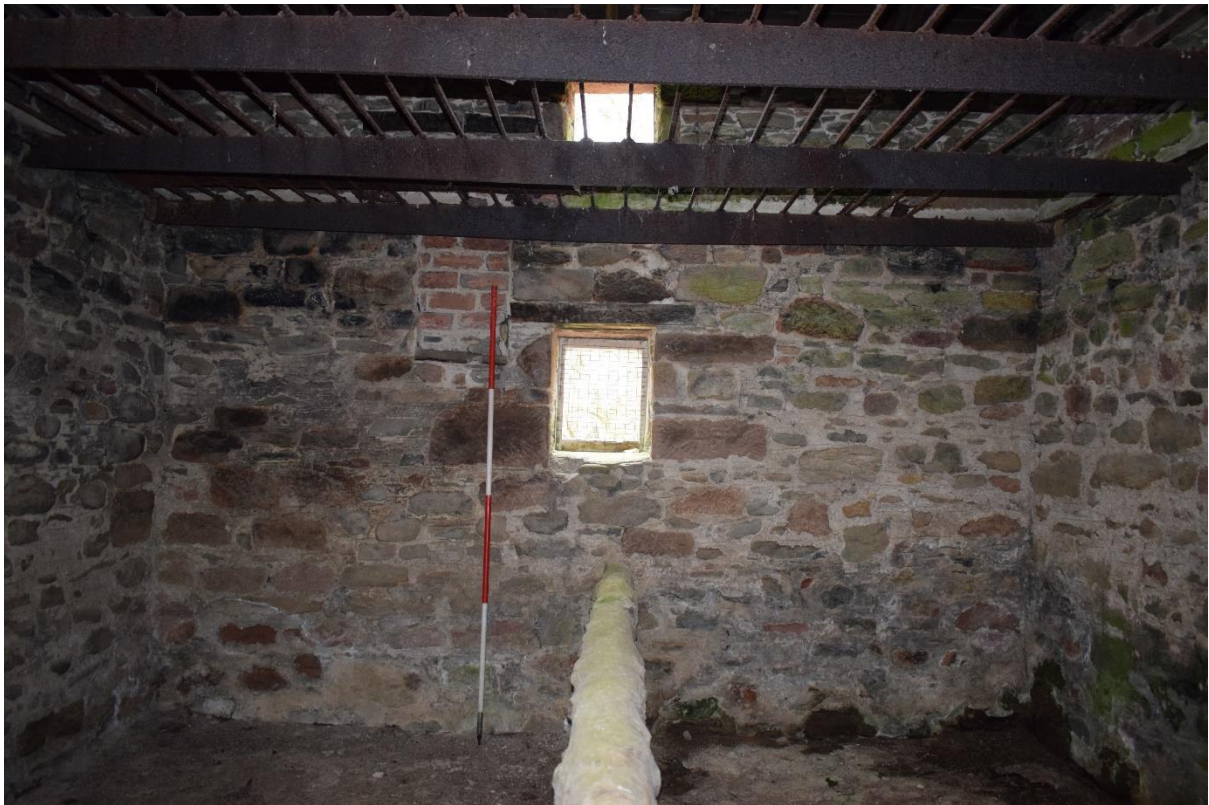
Illus 17 Room 2 NW wall showing burnt stonework and iron frame and mesh with W8 (centre) and brick-blocked aperture F10 (left) probably grain chute and Phase 3 wall F12 (bottom); facing NW.
