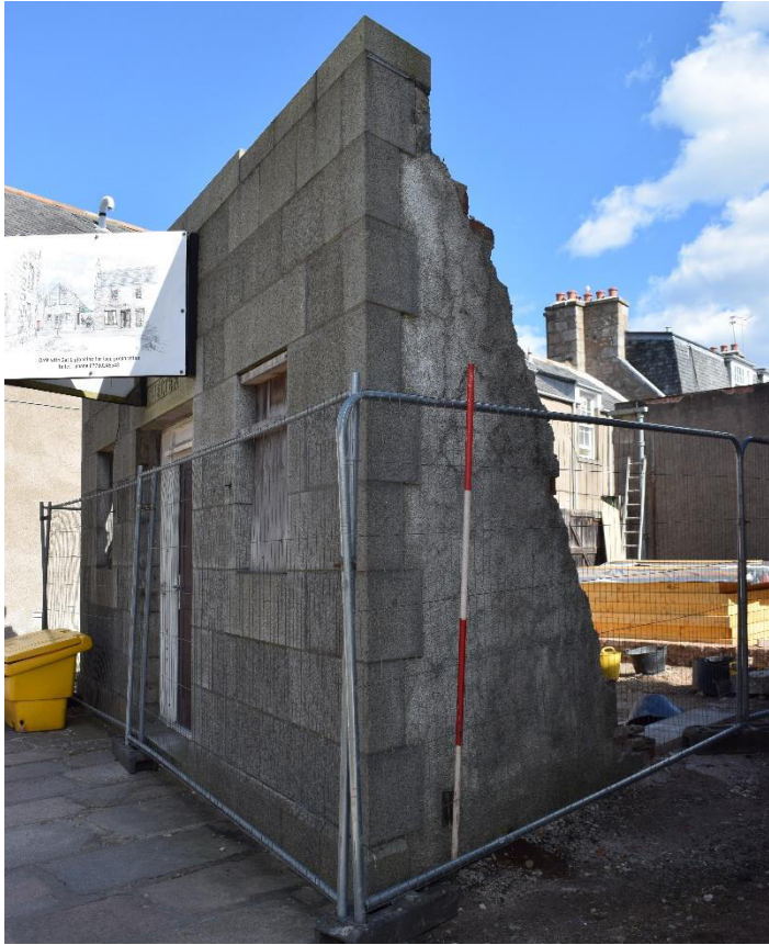
Illus 6 SW corner showing S wall cut down prior to this survey
