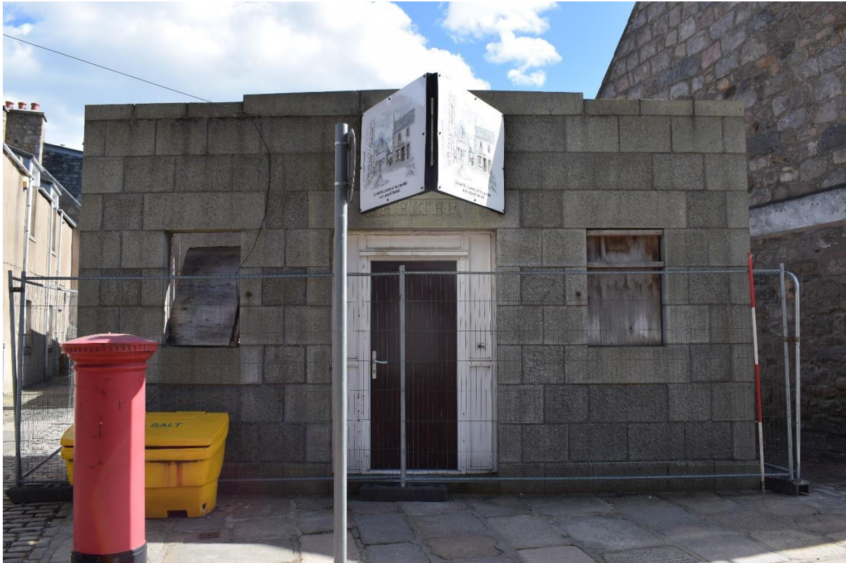
Illus 4 The West façade (exterior) with W1, D1, W2 (left to right); facing W
