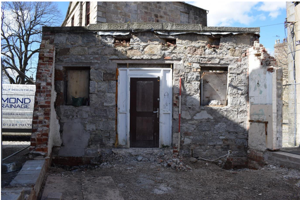
Illus 5 The West façade (interior) with W2, D1, W1 (left to right); facing W
