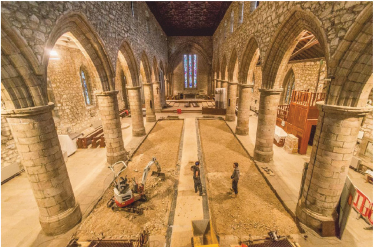
Illus 6 View of St Machar Cathedral interior during pew-removal works, with walling visible just beyond the workers on right-hand (S) side of the main aisle.
