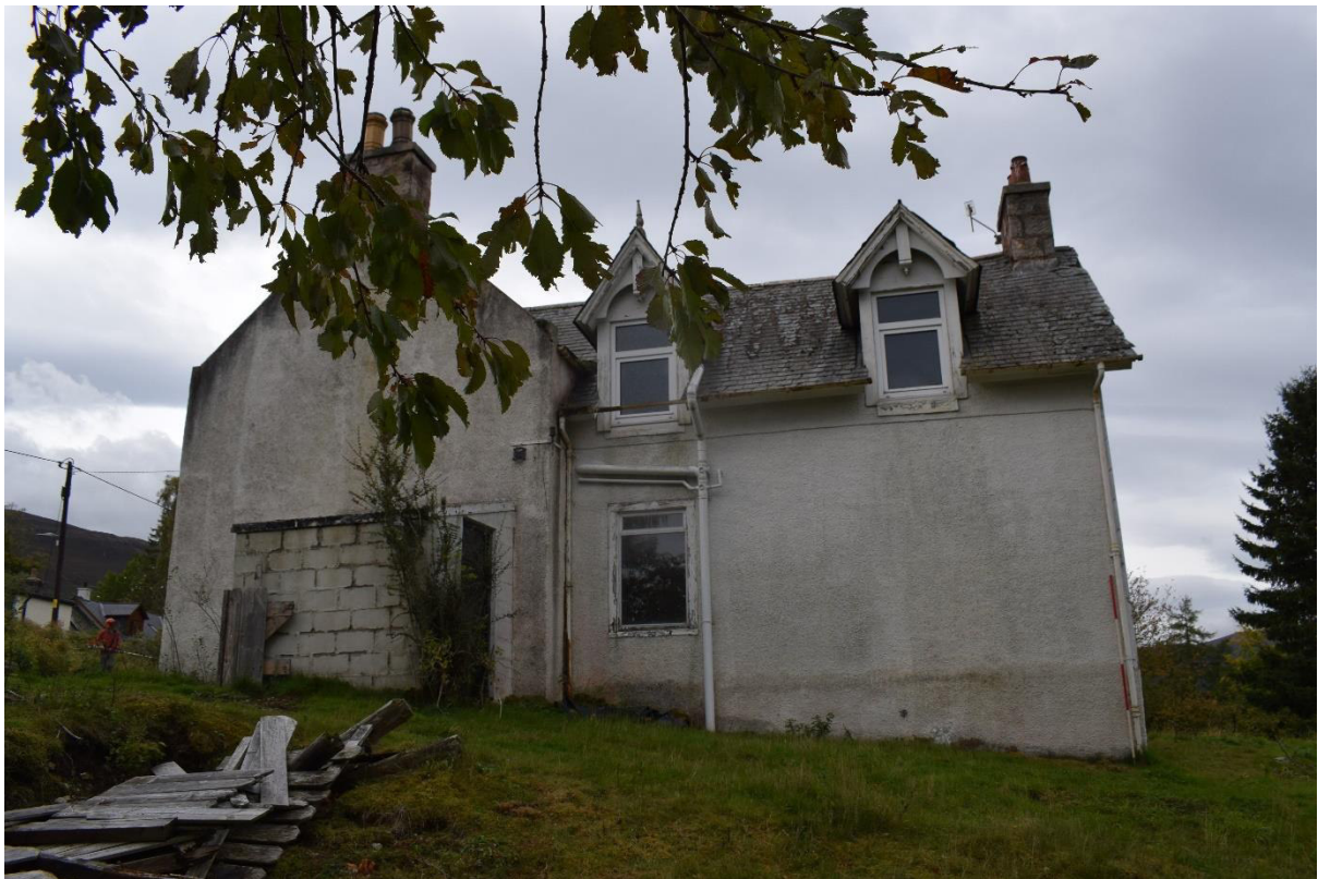
Illus 9 Room 1 (Phase 2) added on to the N of the Phase 1 cottage (left); facing W
