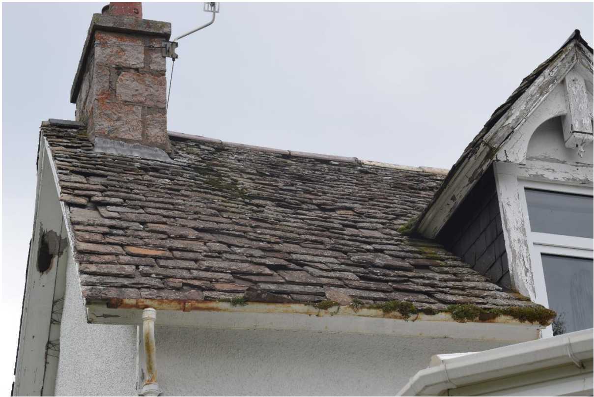
Illus 2 Grey stone roof tiles on Room 13 W facing roof; facing ESE
