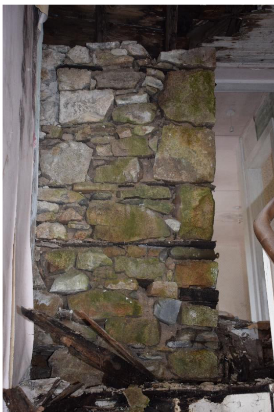
Illus 18 View of stonework for D19 halfway up stairs (not accessible as roof above has collapsed) showing possible first floor window in N wall of Phase 1 cottage; facing N
