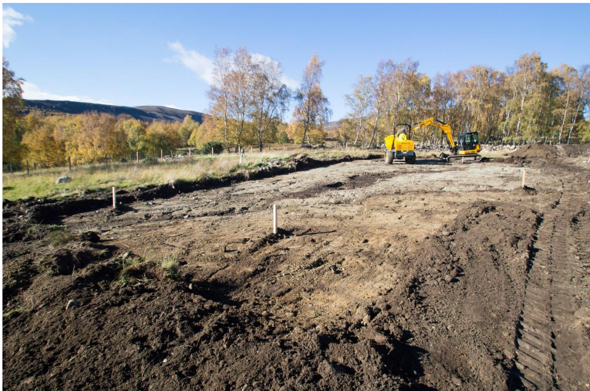
Illus 3 Soil strip nearing completion. Note dark band which comprises shallow (under 0.30m) natural gully in front of dumper, running downslope.
