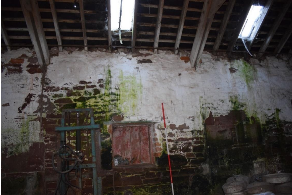
Illus 3 Building 1 Room 3 NW wall D25 with red sandstone facing, blocked with stone and whitewashed and small window W11 added; facing SE
