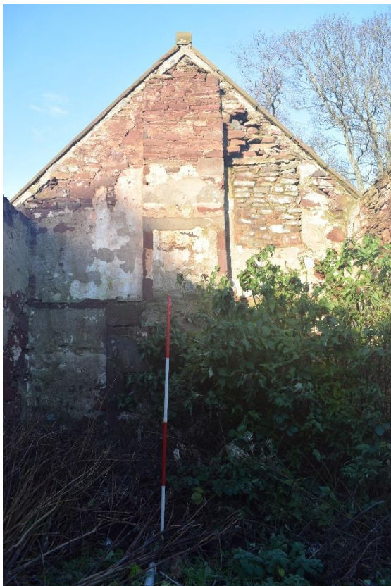
Illus 22 Interior of NNW gable with chimney (centre), D41 (top right) showing overgrown interior; facing NNW
