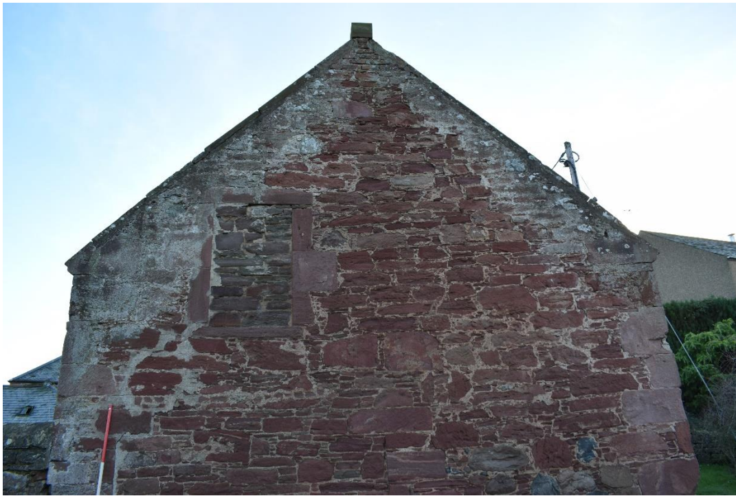
Illus 23 NNW gable upper section showing D41 (top left) with dated skewputt F3 (left); facing SSE
