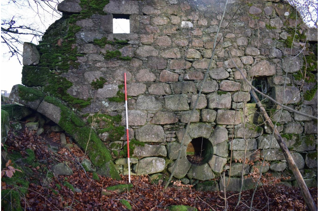
Illus 22 Building 3 S gable with W14 (top left) W15 (right), F1 (centre), F2 (left); facing N
