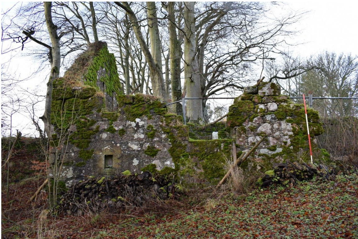
Illus 21 Building 3 E wall with windows W11 and W12 (left) and W13 (centre); facing W
