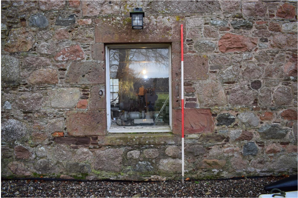
Illus 4 Building 1 W façade Window W1; this will be converted to a door; facing E
