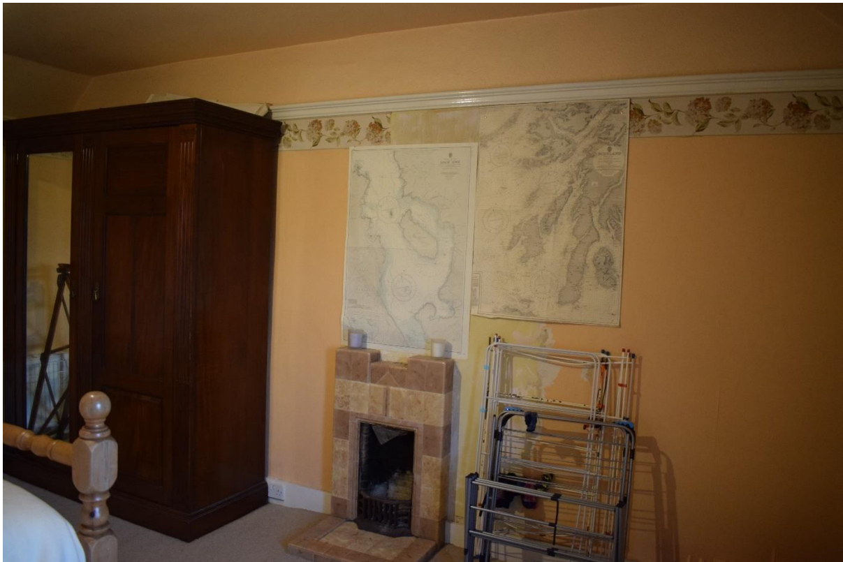
Illus 6 Building 1 Room 1; a door will be inserted behind the wardrobe to access Room 2; facing NE
