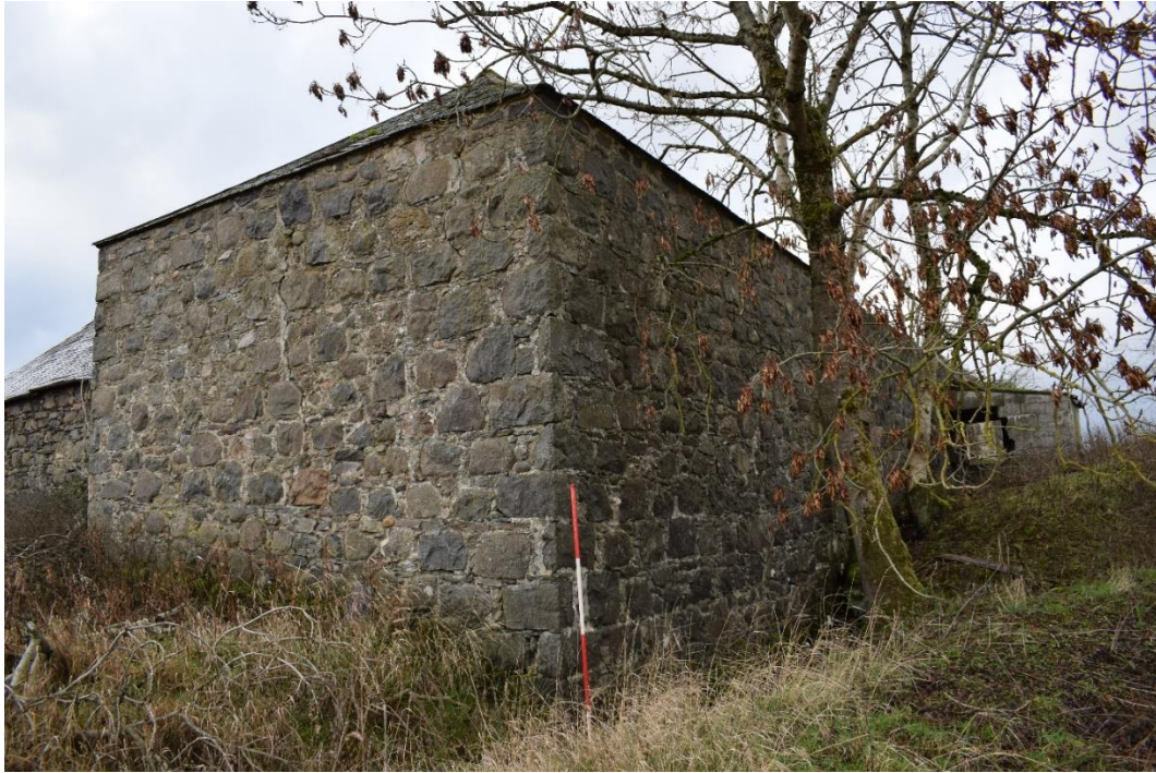
Illus 4 NE corner of Room 7 showing the infilled lade (at the bottom of the ranging rod); facing SW
