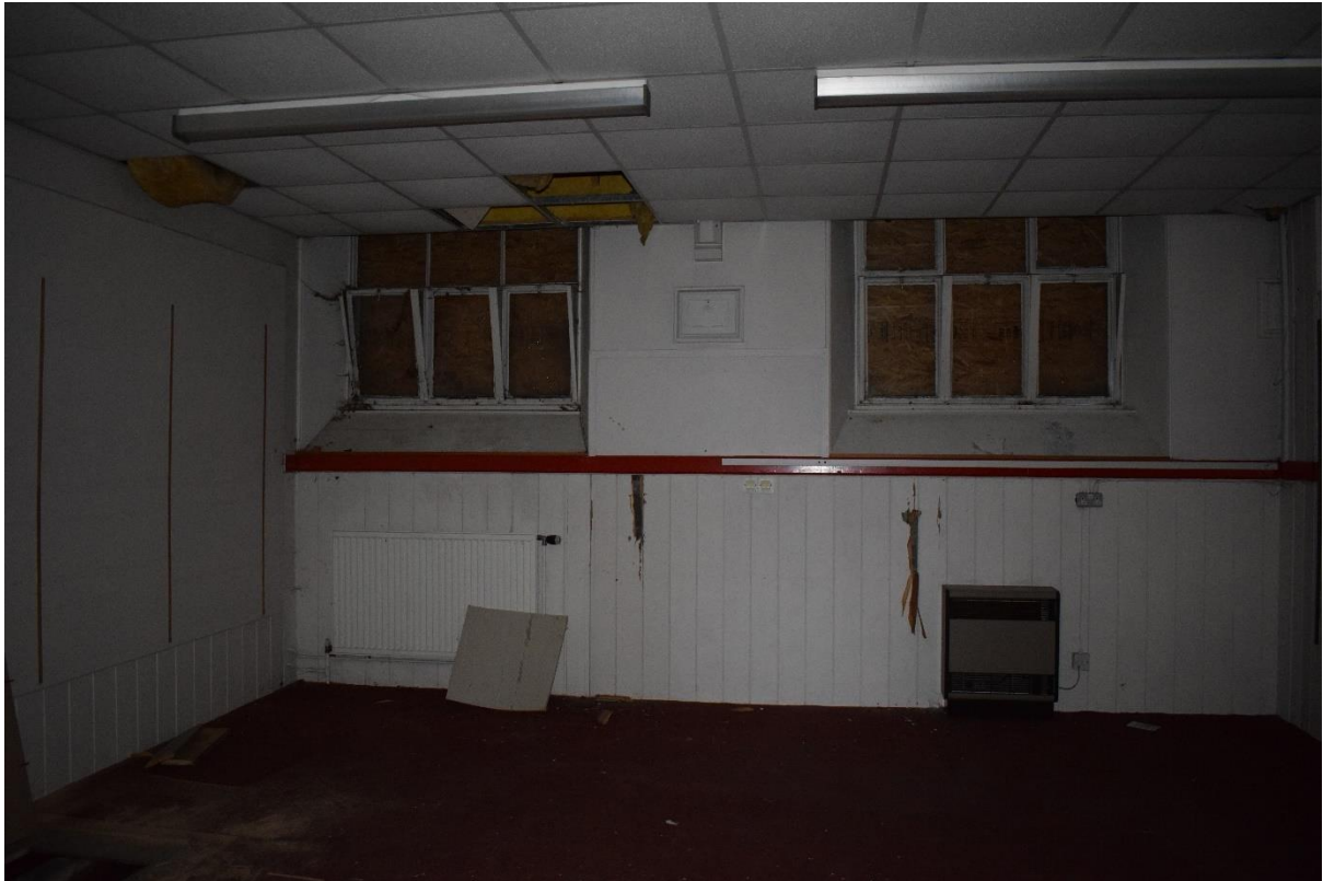
Illus 10 Building 1 Building Room 6 S wall W43, W37 showing original wood panelling, wall partitions and lowered ceiling; facing S
