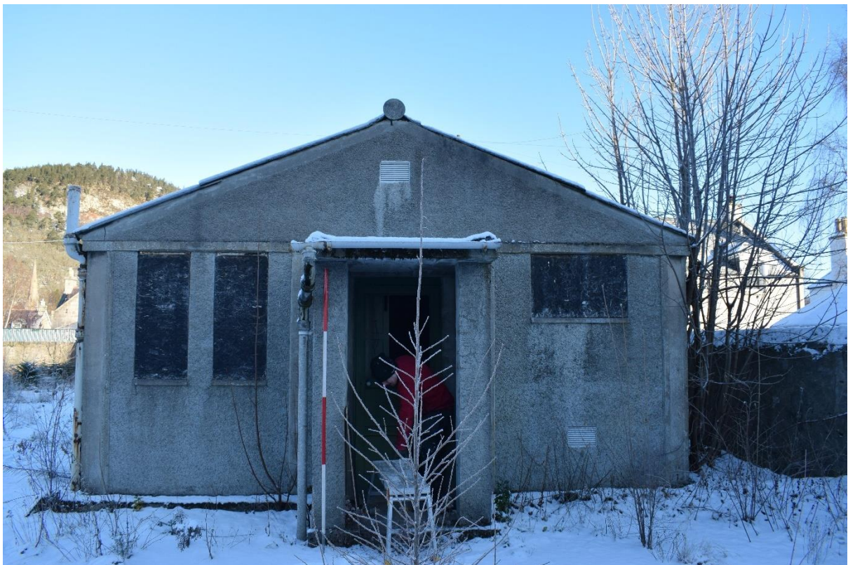
Illus 33 Building 6 S gable with W25 (left), W26, D9 and W27 (right); facing N
