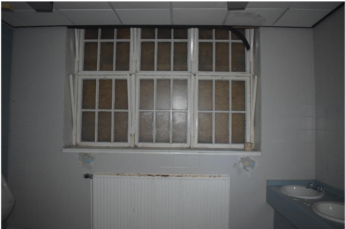
Illus 7 Building 1 Room 2 N wall window W46 showing modern wall partitions to create bathroom and lowered ceilings; facing N
