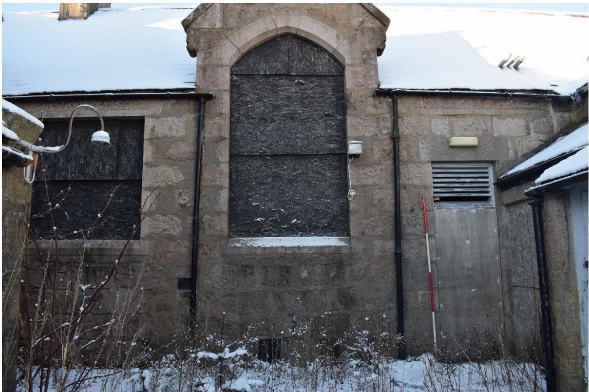
Illus 9 Room 4 E wall windows W67 and W61 (centre) and blocked door D21 (right); facing W
