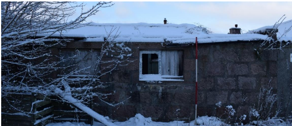
Illus 21 Building 3 E façade with W4 (centre) and W2 and W3 (left, behind tree); facing W
