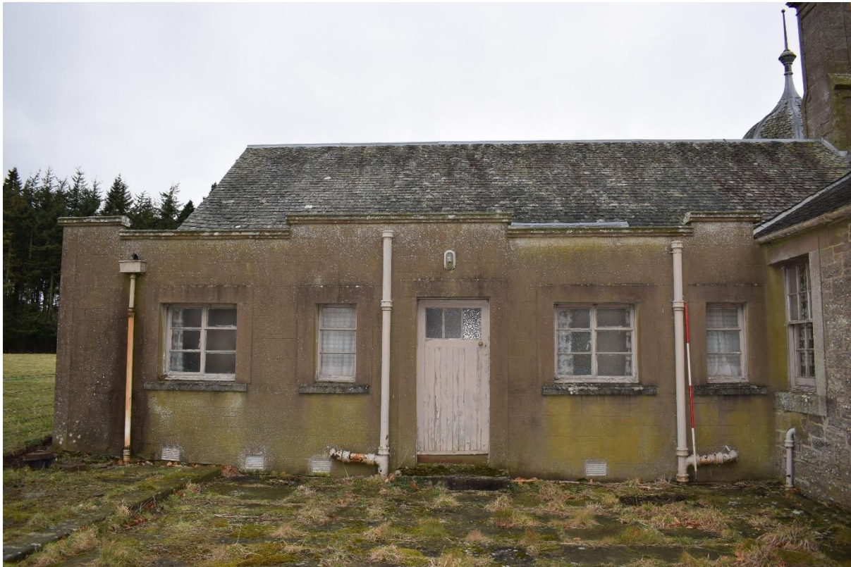
Illus 51 WSW courtyard NNW wall concrete extension W53, W54, D8, W55, W25 (l-r); the wall at the left of this photograph has been harled following the demolition of the rest of the adjoining house in 1955; facing NNW
