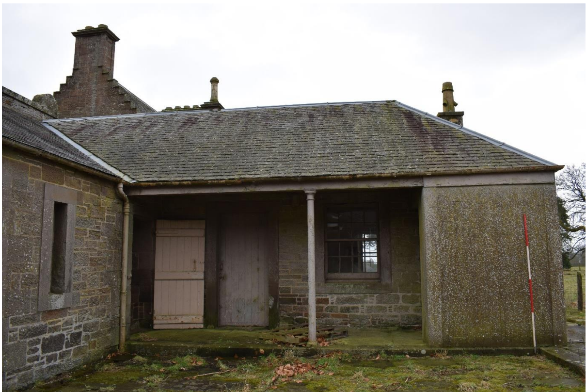
Illus 50 WSW courtyard SSE wall D10 (centre) W57 (right) showing harled wall (right) where remainder of courtyard was demolished in 1955; facing SSE
