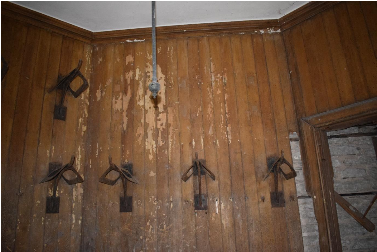
Illus 26 Room 12 the tack room with saddle racks on SW wall; facing SW
