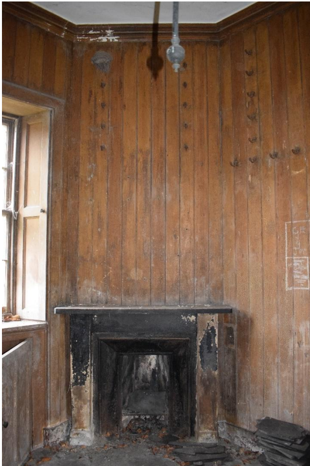
Illus 25 Room 12 the tack room with fireplace F17, W11 (left) and wood paneling; facing NE
