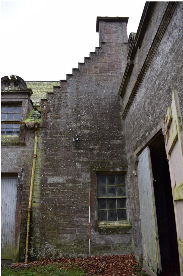
Illus 11 Stables NNW elevation W71 with later wall Room 8 attached facing SSE
