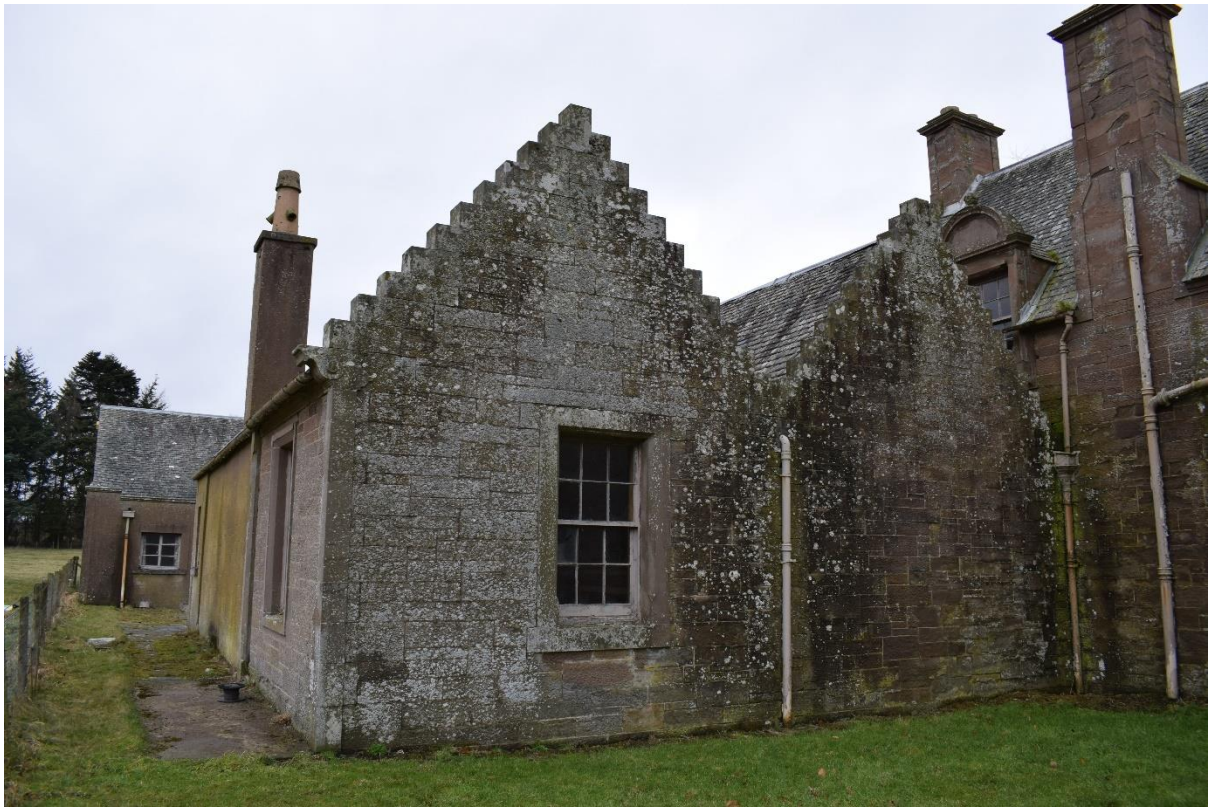
Illus 49 Rooms 6 and 7 WSW M-gabled crow-stepped extension with W1 (left); facing N
