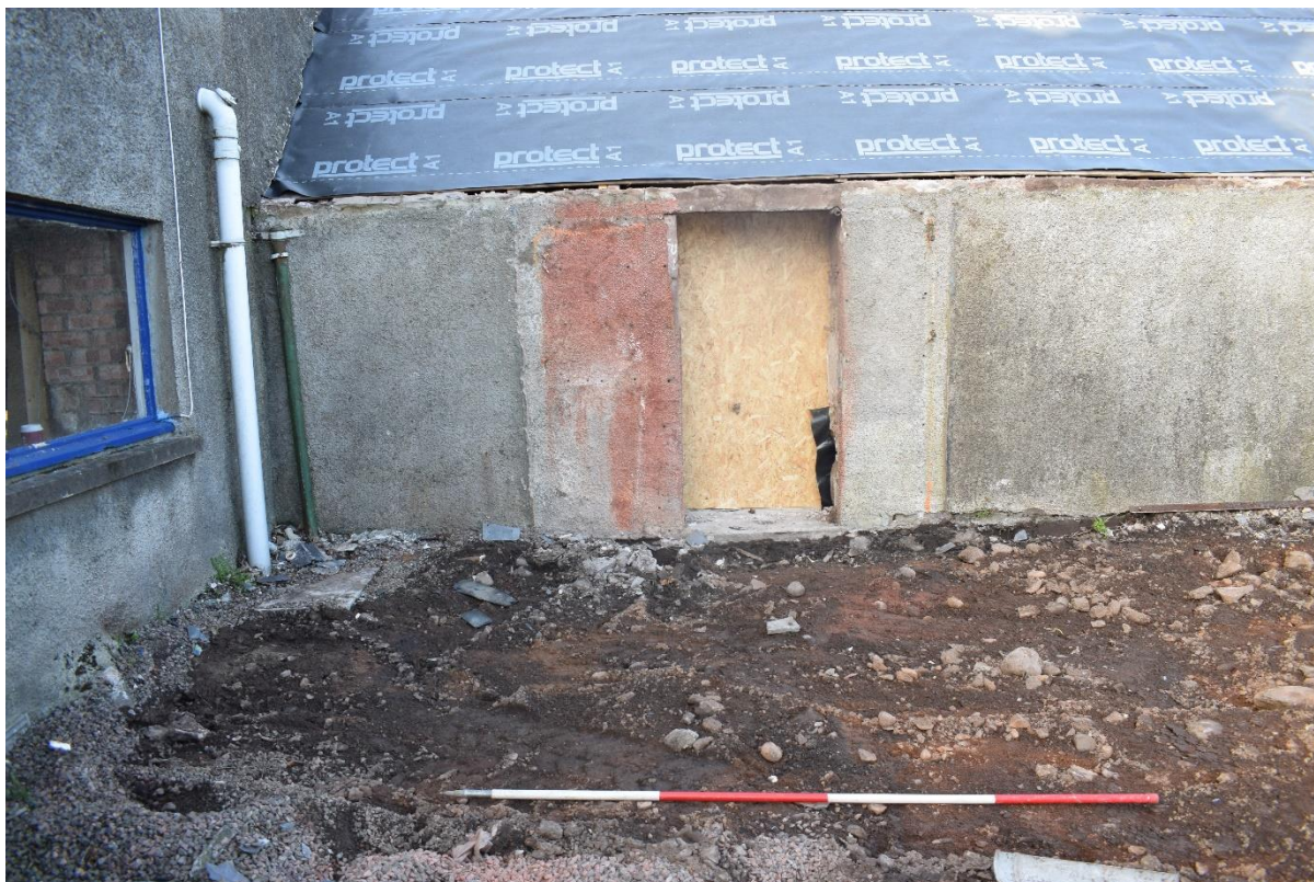
Illus 4 Area B stripped of concrete showing soil and concrete mix below; facing WSW
