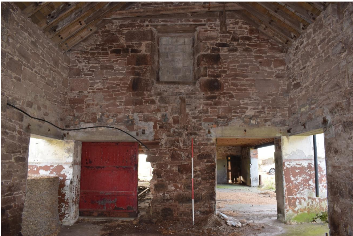
Illus 13 NW exterior wall Rooms 8 and 9 showing doors D22 (left), D21 (right) and D23 (above); facing SE. Note the walls on the L and R of this photograph are not included in the current development.
