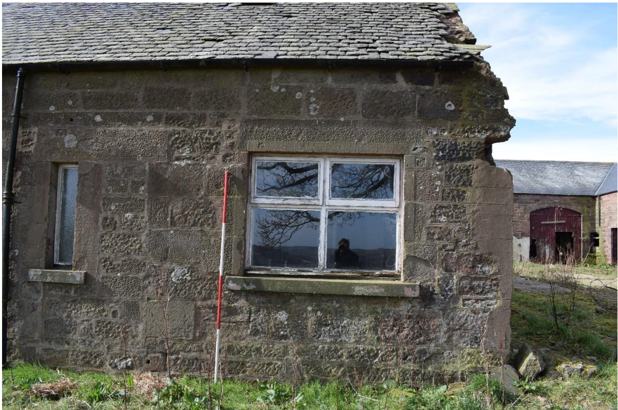
Illus 6 Farmhouse Room 6 NE façade showing sandstone sills, lintels and jambs with steading building removed (right); facing SW
