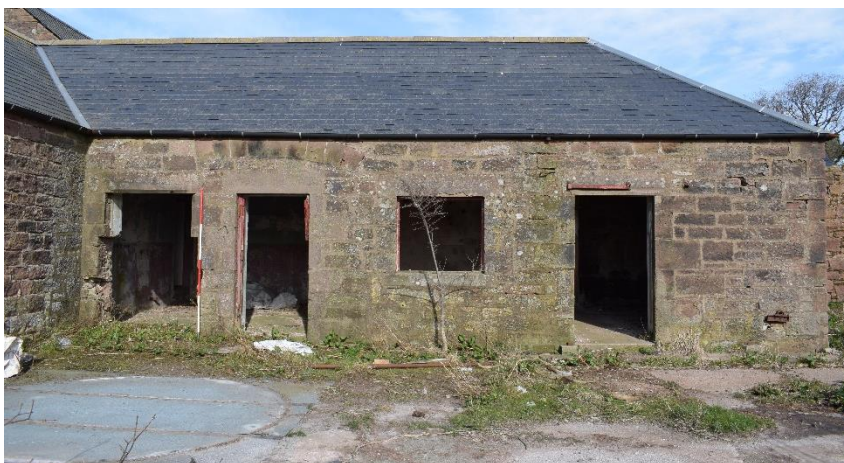
Illus 9 Room 7 SE wall W7, D6, W8, D7 (l-r); facing NW
