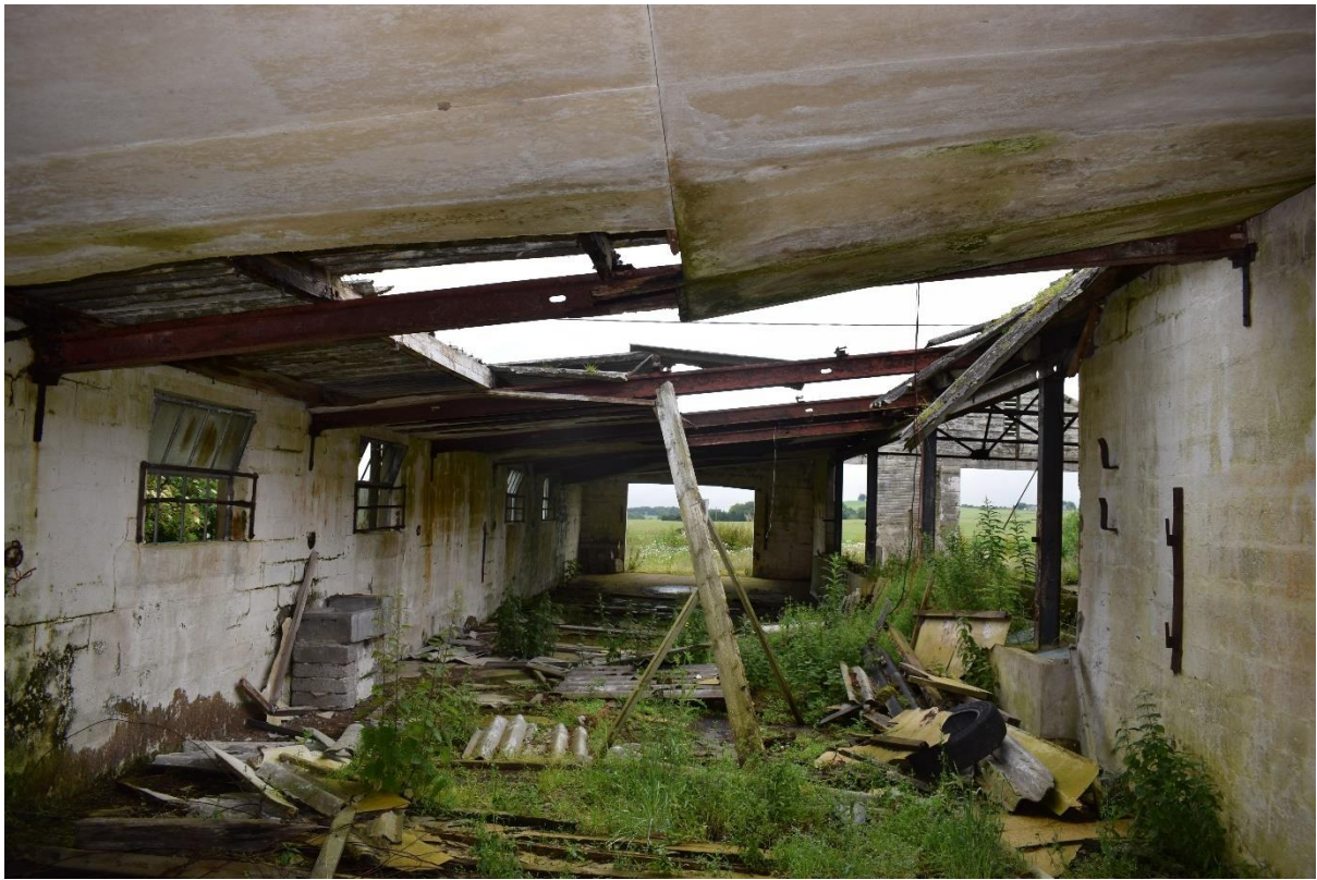
Illus 25 Building 6 interior showing collapsing roof and asbestos roofing broken on floor; facing NNE
