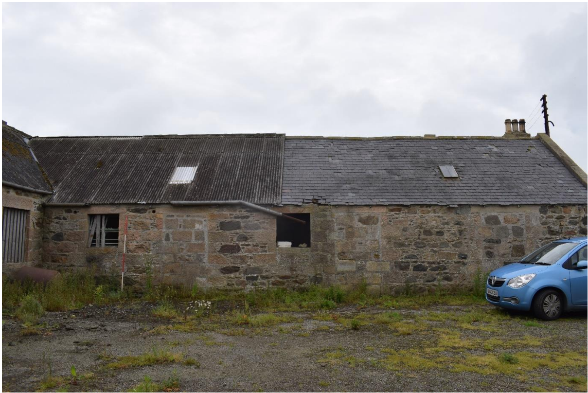
Illus 15 Building 4 E wing WNW wall W4, D9, W17, D7, D6; facing ESE
