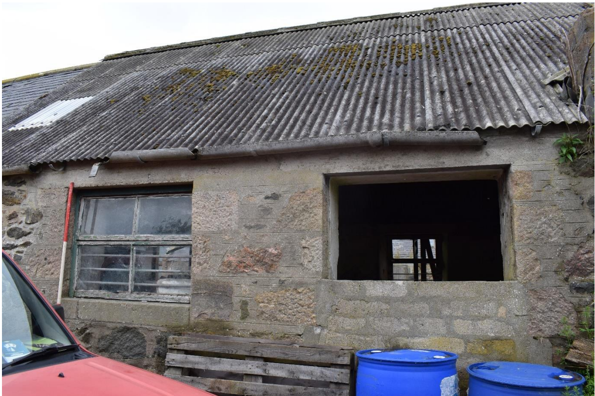
Illus 18 Building 4 E wing W3 (left) with new concrete sill, D2 (right) blocked with concrete
