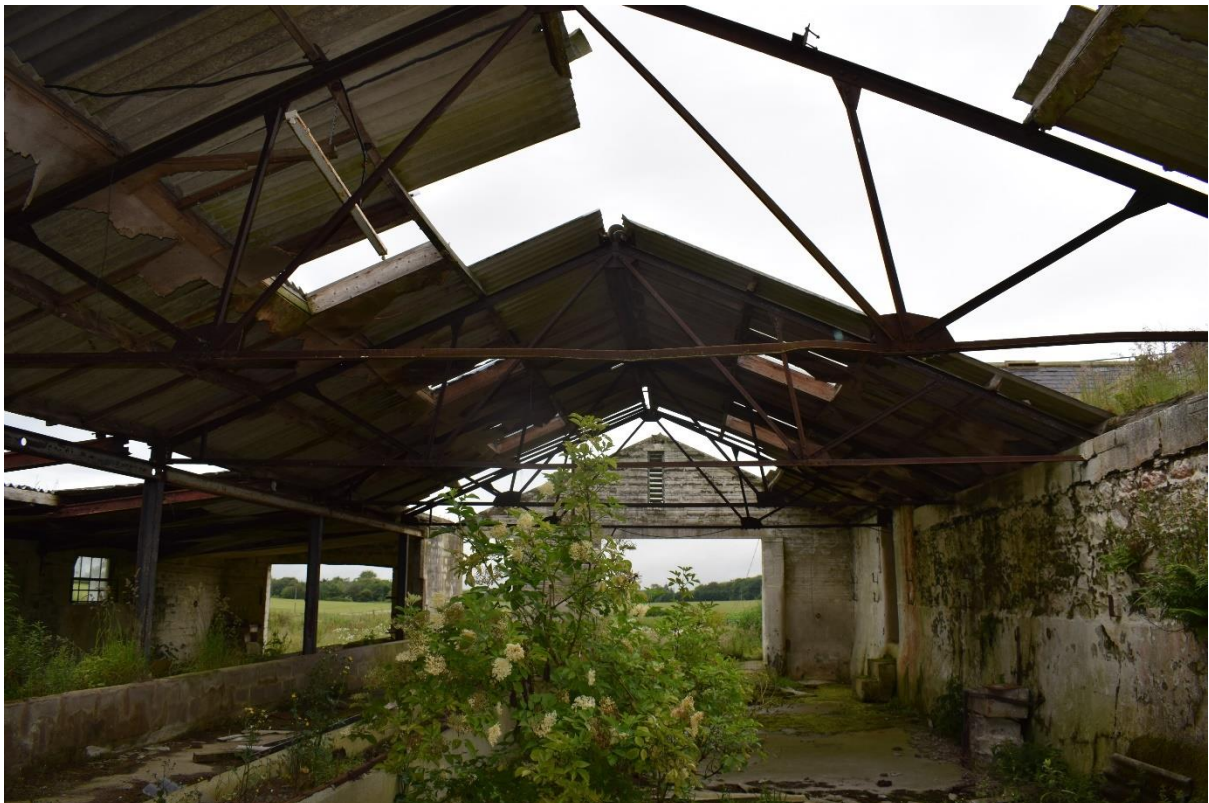
Illus 22 Building 5 interior; facing NNE showing collapsing roof and asbestos roofing broken on floor
