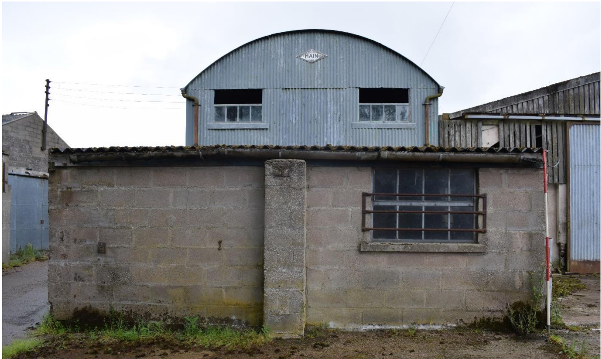
Illus 3 Building 1 WNW end showing concrete base and metal upper floor; facing ESE
