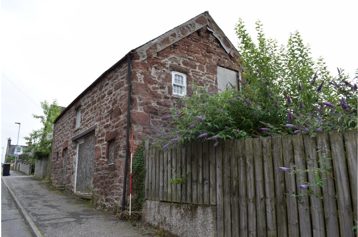
Illus 6 SW gable with W6 (left), blocked door (D4; right) and roof raggle F3; facing NE
