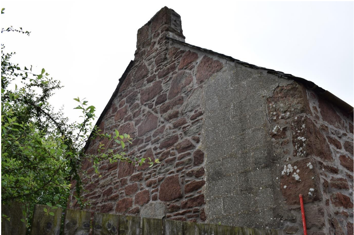
Illus 5 NE gable with roof raggle F1 (left), blocked door D5 (right) and sandstone chimney F2 (top); facing S
