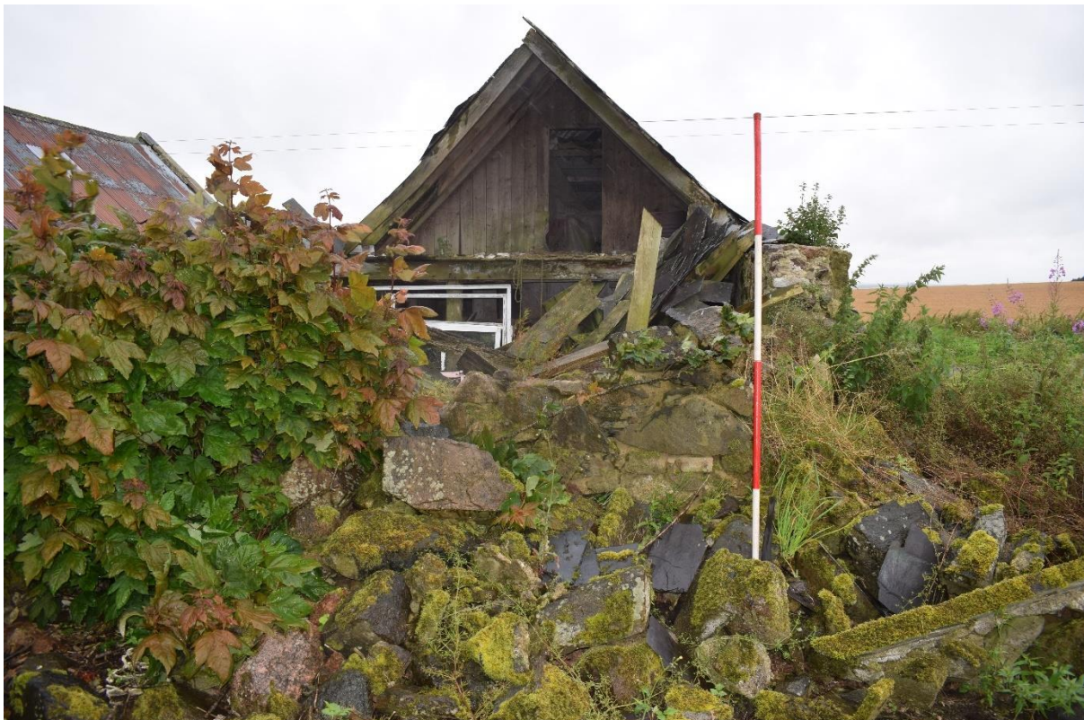
Illus 4 Building 1 collapsed NE gable; facing SW
