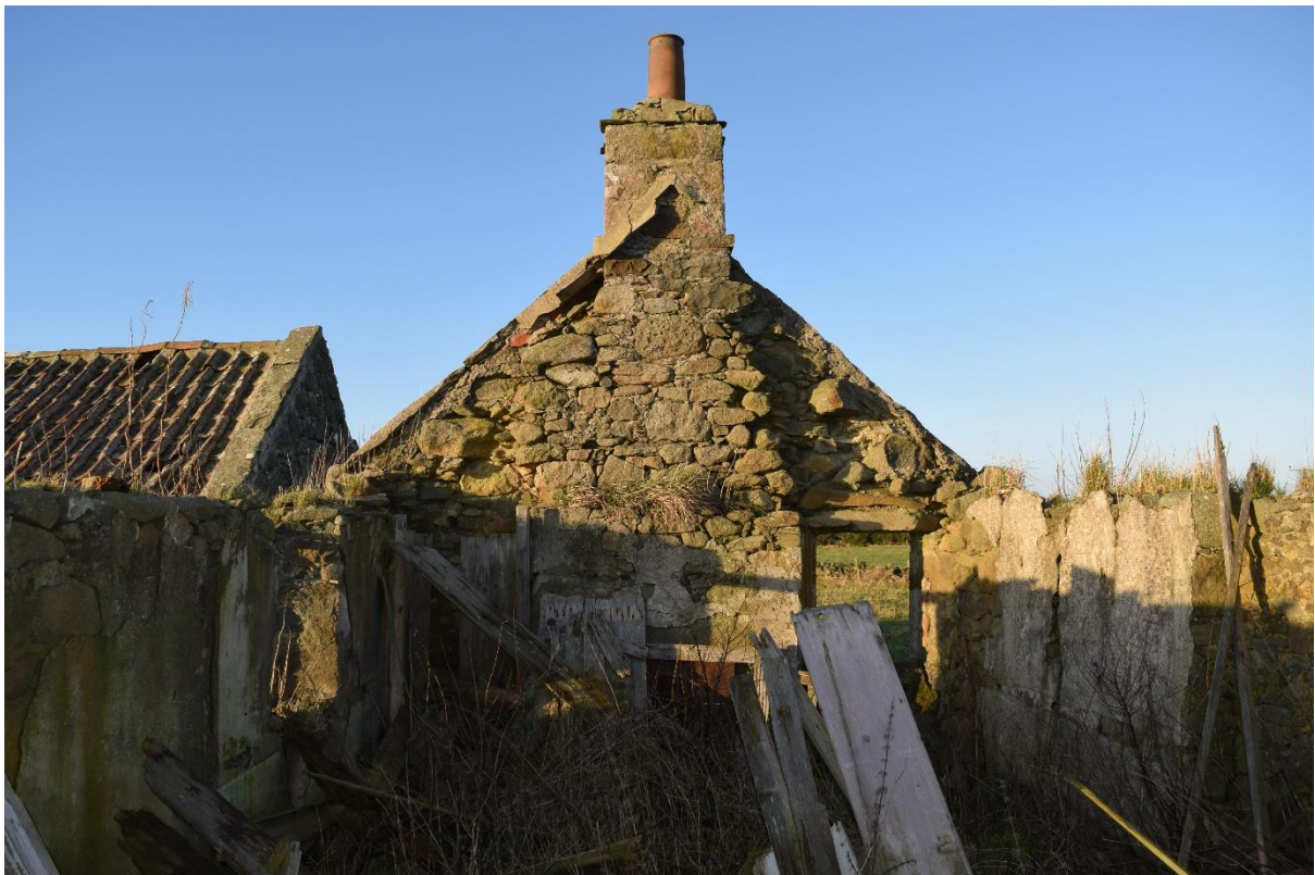
Illus 5 Building 1 Room 1 interior of W gable showing collapsed roof and rubble interior; facing W
