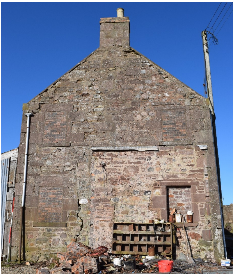
Illus 16 Room 10B SE gable with W1 (top left), W2 (top right), W3 (bottom left) W4 blocked with stone (bottom right); facing NW
