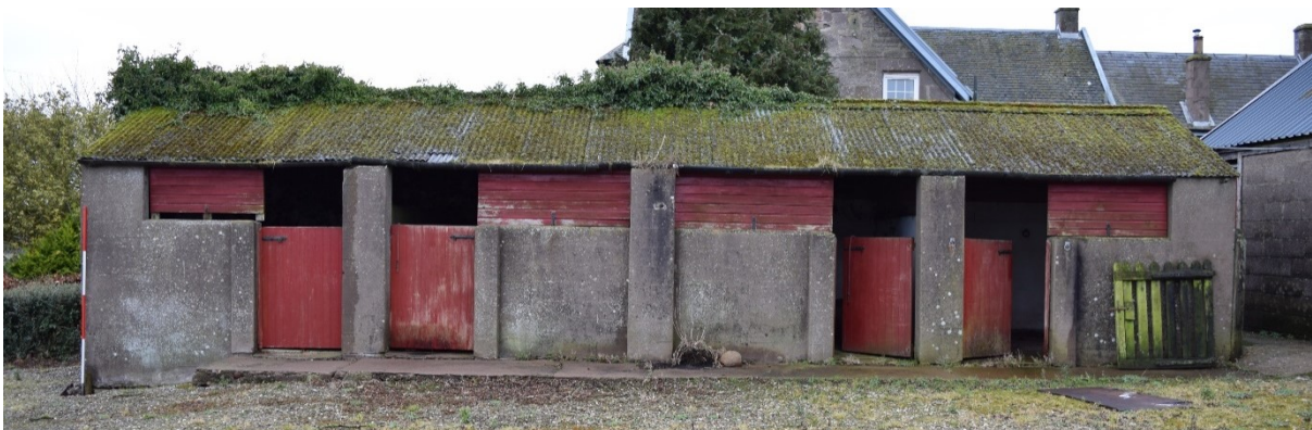
Illus 22 NE façade Rooms 1-4, stabling for horses in concrete blockwork; facing SW
