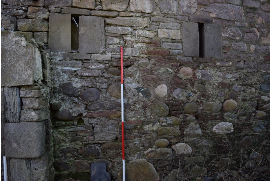
Illus 19 Room 16 NE wall exterior windows W27 (left) W28 (right) with Phase 2 wall of Room 18 (left showing SW jamb D12); facing SW
