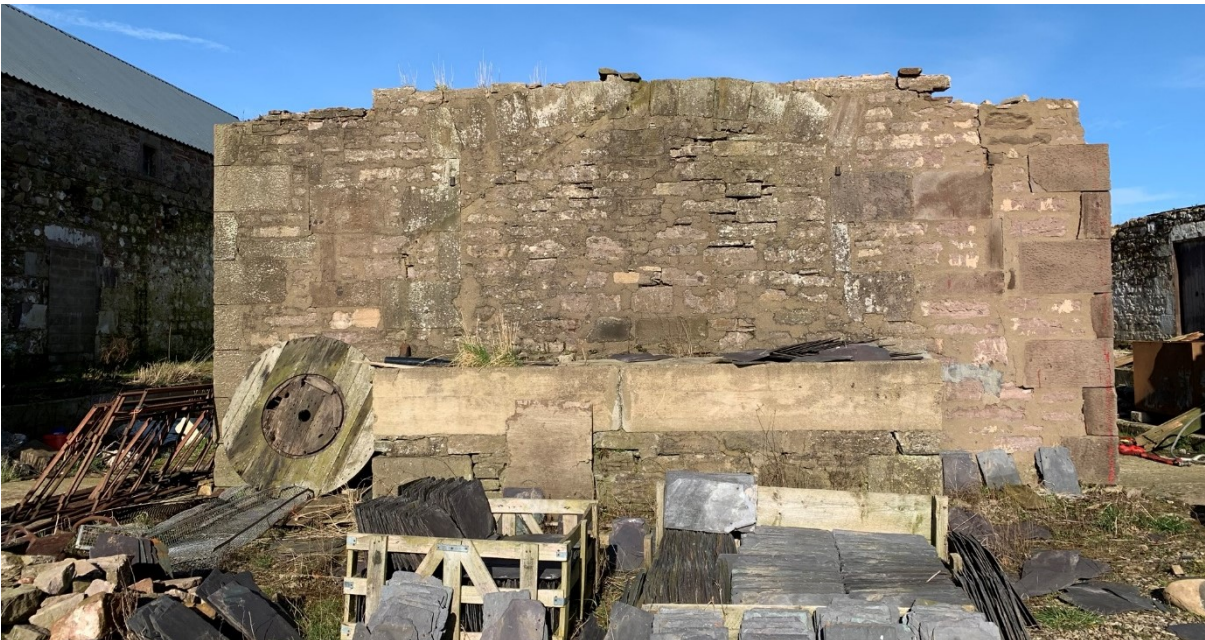
Illus 10 Cart door D39 blocked (centre) with D8 (left) and D9 (right); facing NW
