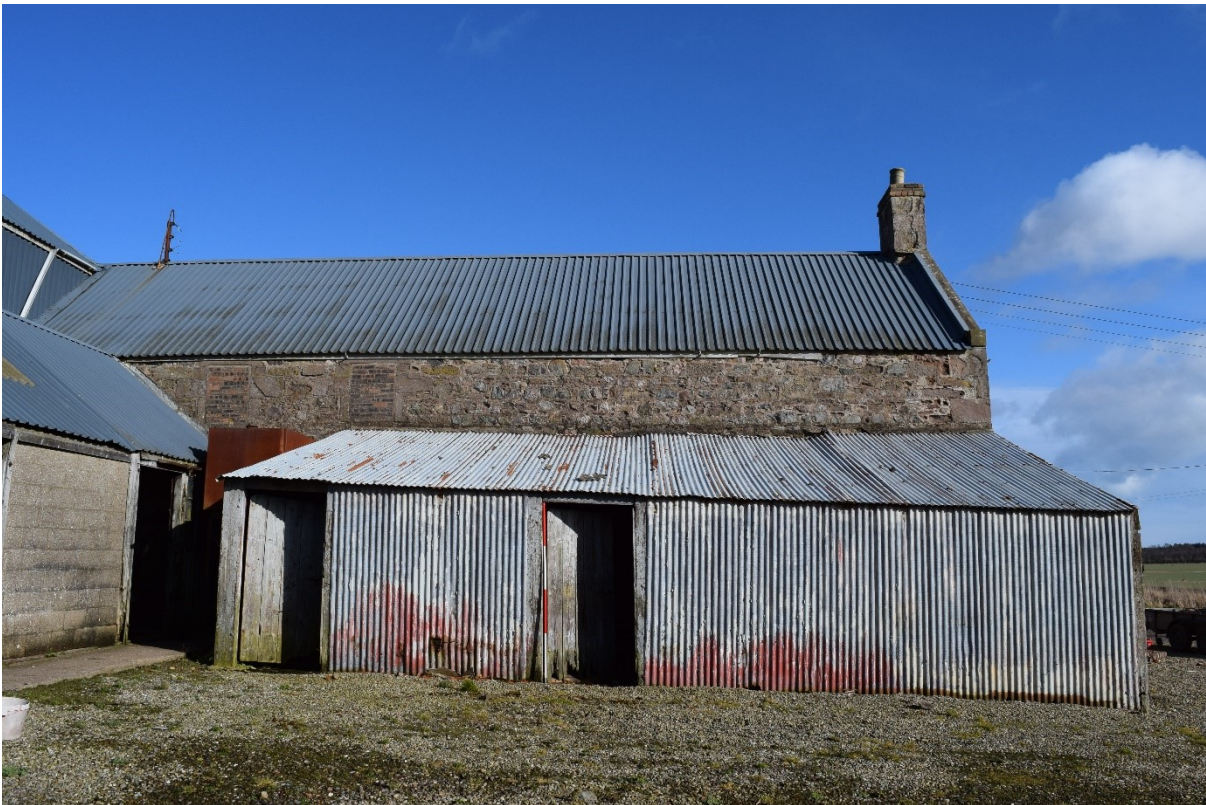
Illus 15 Room 10B SW façade with blocked windows W5 and W6 (top left) and Room 13 metal lean-to shed (foreground); facing NE
