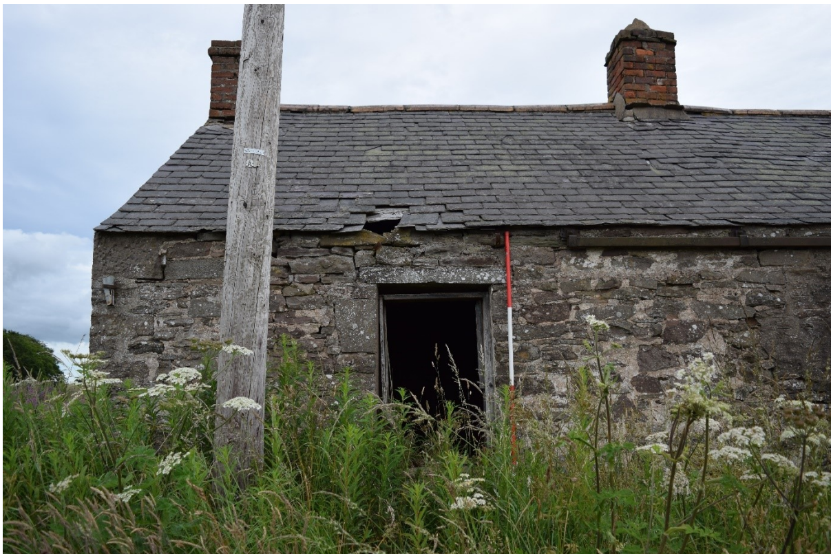
Illus 4 Room 1 SW wall W1 with brick chimneys F1 (left) and F2 (right); facing NE
