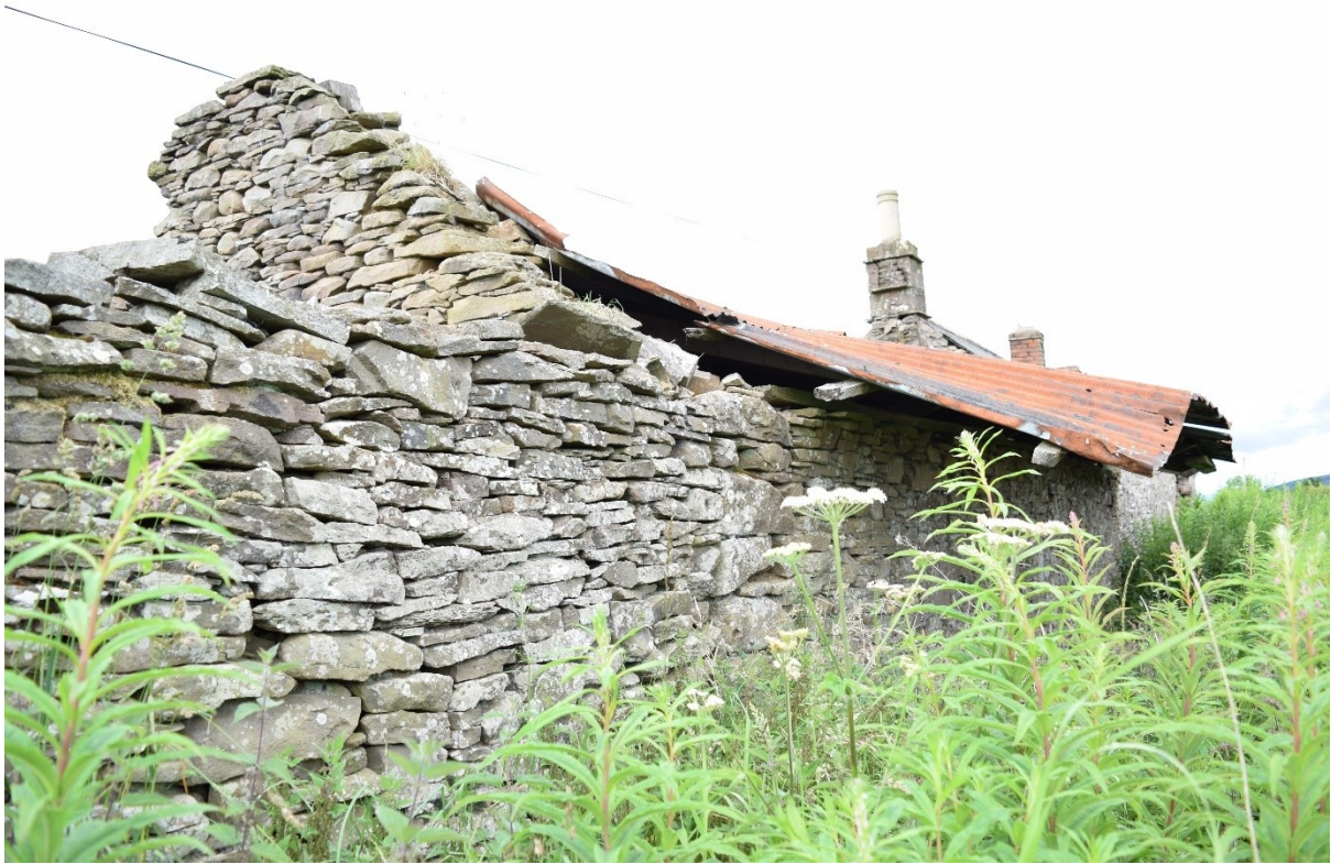
Illus 7 NE wall showing slipped corrugated metal roof; facing WNW
